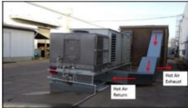
Figure 2.2 Modular Data Center: Hot Air Data Center Return Duct
