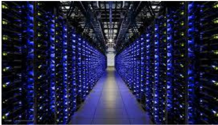
Figure 1 Facebook data center [1]
