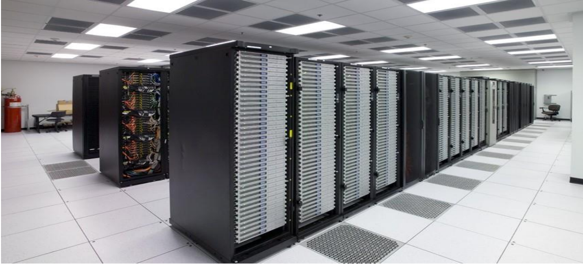
Fig 1: USC Data Center
