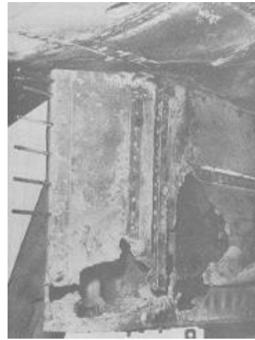
Figure 1.2: X-15 Lower Pylon damage due to localized heat flux [2].
