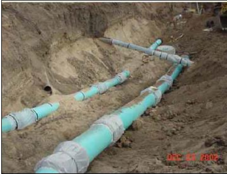
Figure 1-13 Failure of PVC Pipe due to Improper Bedding Conditions (Lackey, 2010)
