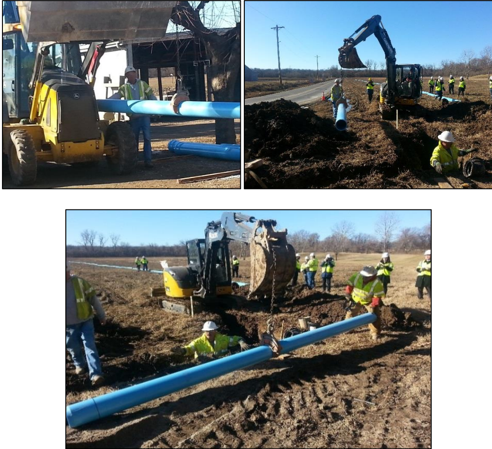
Figure 4-26 iPVC pipe Pilot Installation by MOAW at Meramec River Bottom Road, St Louis County, MO. (Source: AW)
