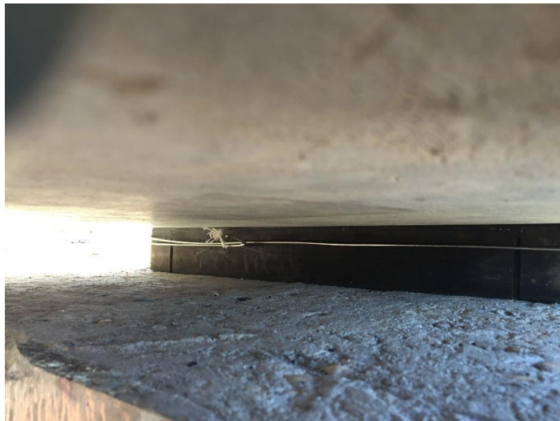
Figure 3-5 Thermocouple on bearing pad
