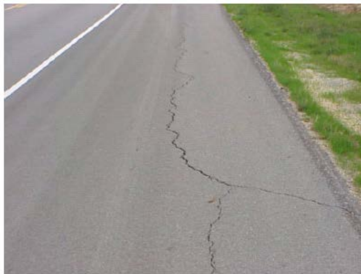
Figure 2:2 Pavement distress due to expansive soil movement (Manosuthikij, 2008)
