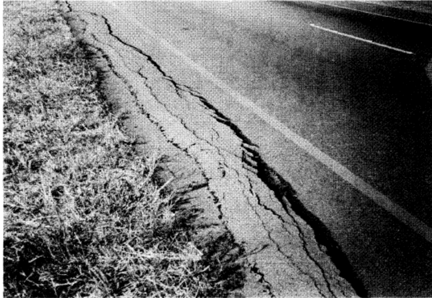
Figure 2:31 Crack at pavement edge after installing vertical barrier (Steinberg, 1989)
