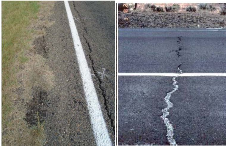
Figure 2:7 Longitudinal and transverse cracking (Hedayati, 2014)
