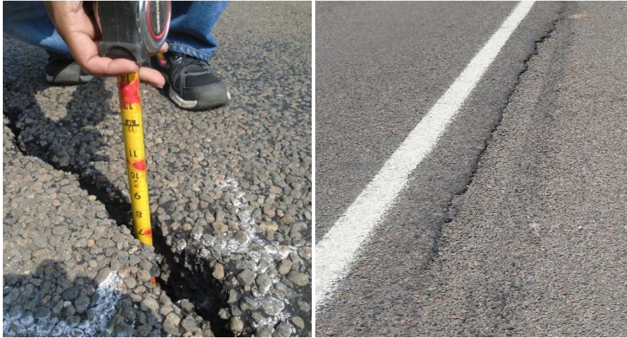
Figure 3:1 Distress condition in pavements
