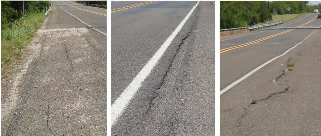
Figure 2:4 Pavement distress in Texas Highways
