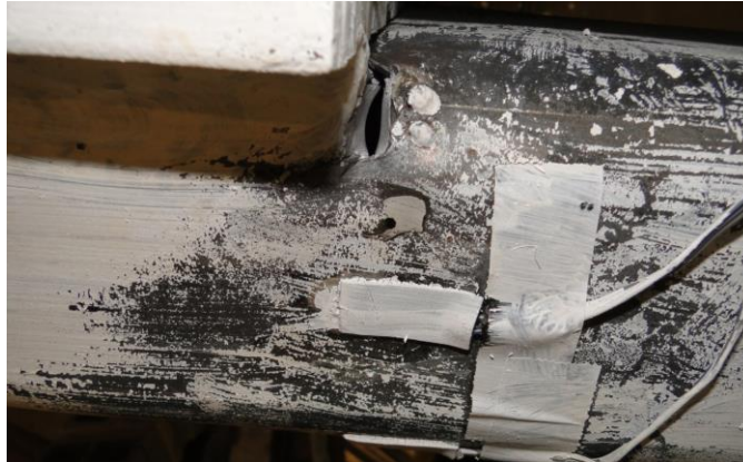
Figure 4-29 Fracture on the flange of HSS at +0.09 rad member rotation
