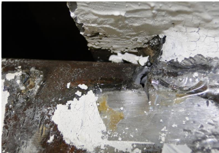
Figure 4-22 Fracture on the west flange at the end of the weld
