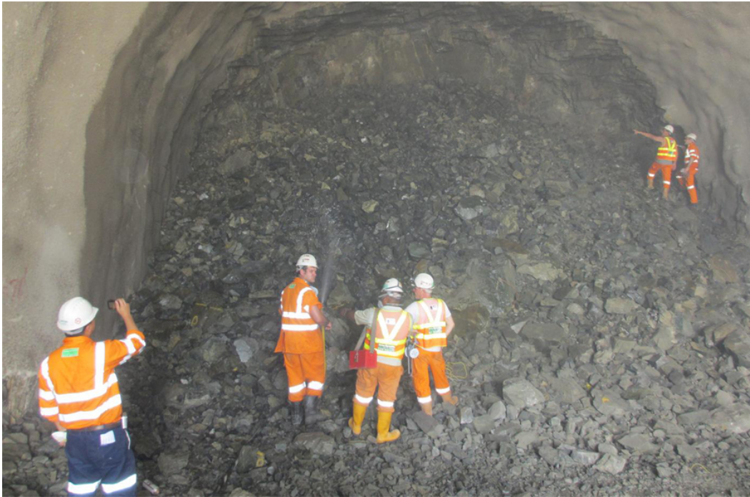
Figure 1-2 Tunnel Surface after Blast (Tunneltalk, 2017a)
