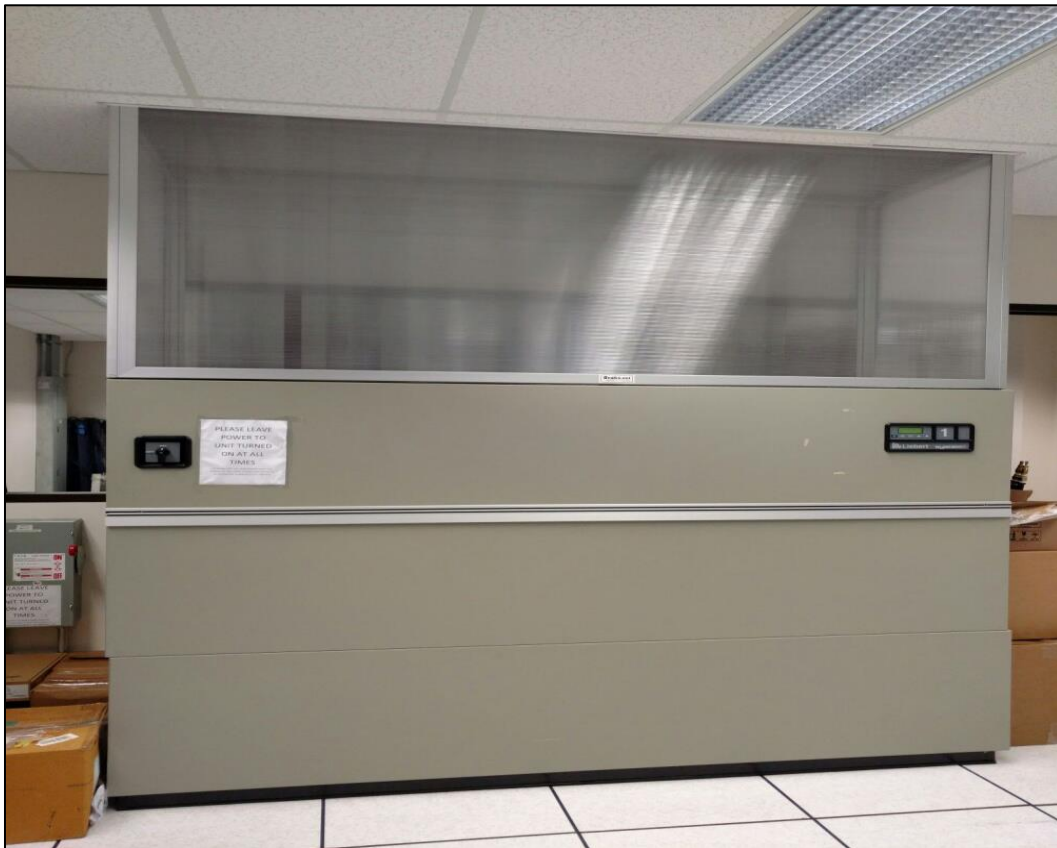
Figure 2-10 CRAH Unit in Data Center lab at UT Arlington
