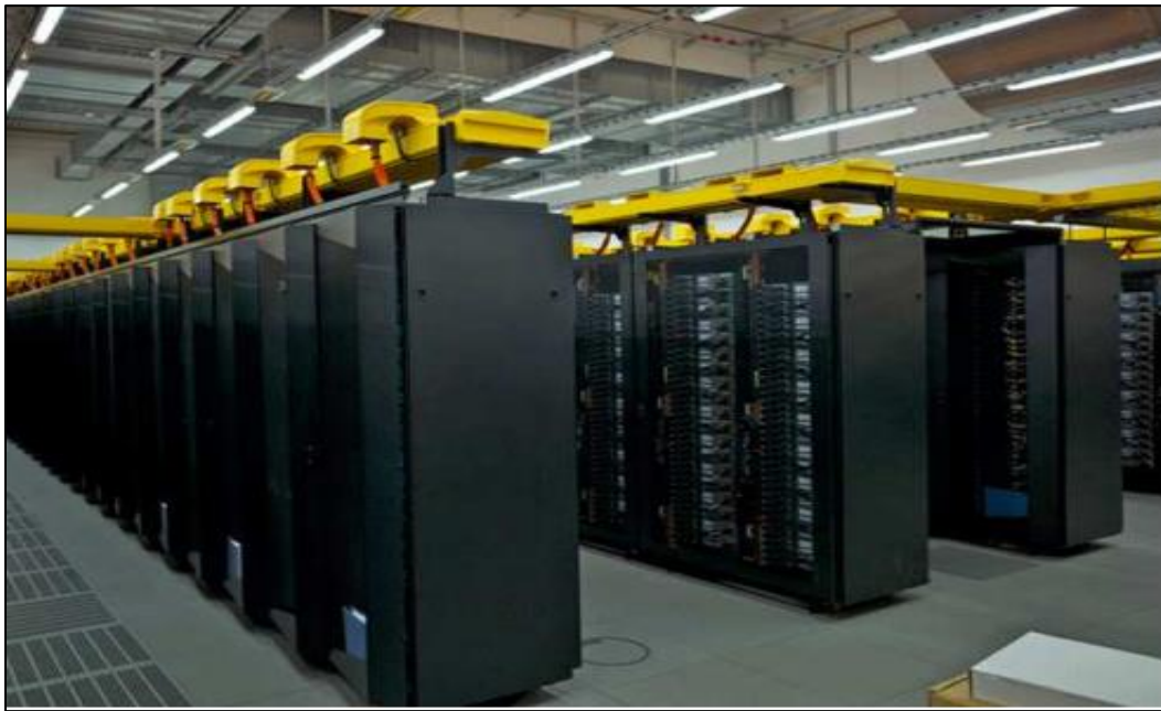
Figure 1-6 Liquid-based Cooling at IBM [4]
