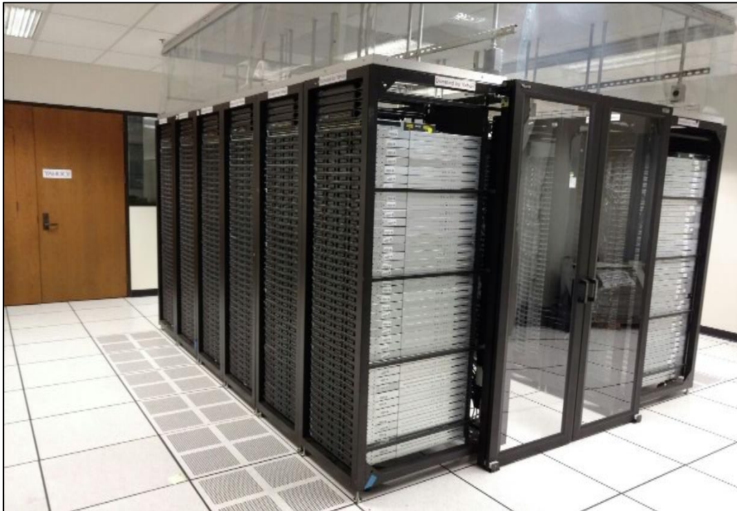
Figure 1-3 Infrastructure for Air Cooling of Server Racks in Data Center at UTA
