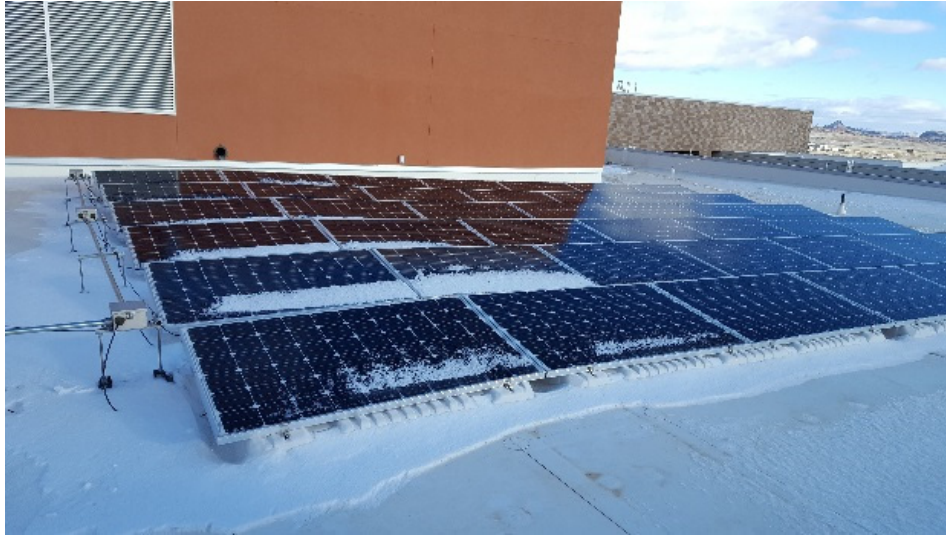
Figure 3-6 Snow accumulated in the PV modules
