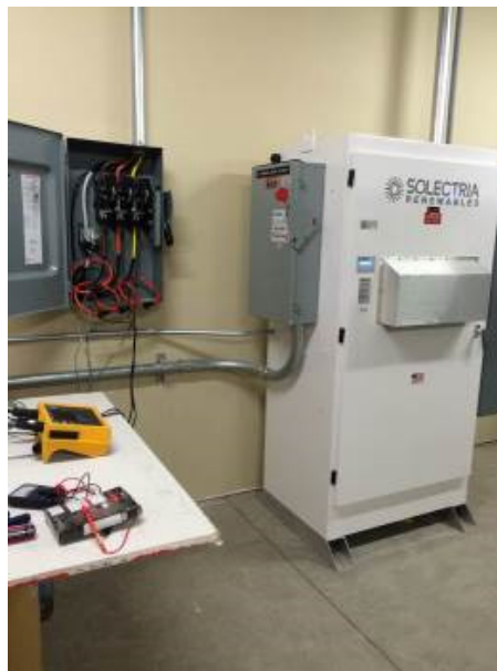
Figure 2-1 Power Logger (Fluke 1735) installed in the output of the Inverter
