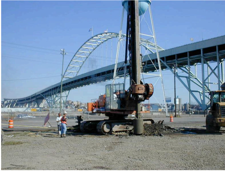
Figure 2-5 Rotasonic Sampling for a CSO Tunnel at Portland, Oregon (Hung et al. 2009, p. 3-18)
