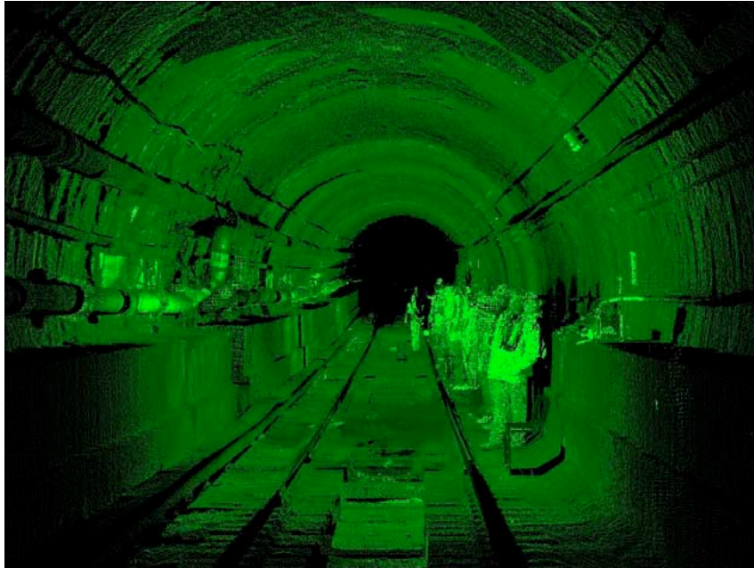
Figure 2-3 3D Laser Scanning Tunnel Survey Results in Actual Scanned Points (Hung et al. 2009, p. 3-7)
