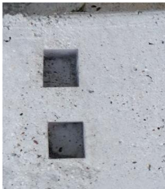
Figure 8 Artificial voids in Beam 6
