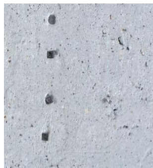
Figure 5 Artificial voids in Beam 3
