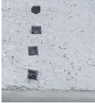
Figure 6 Artificial voids in Beam 4
