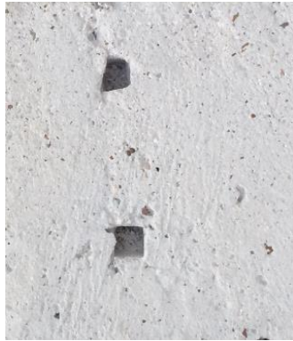
Figure 7 Artificial voids in Beam 5
