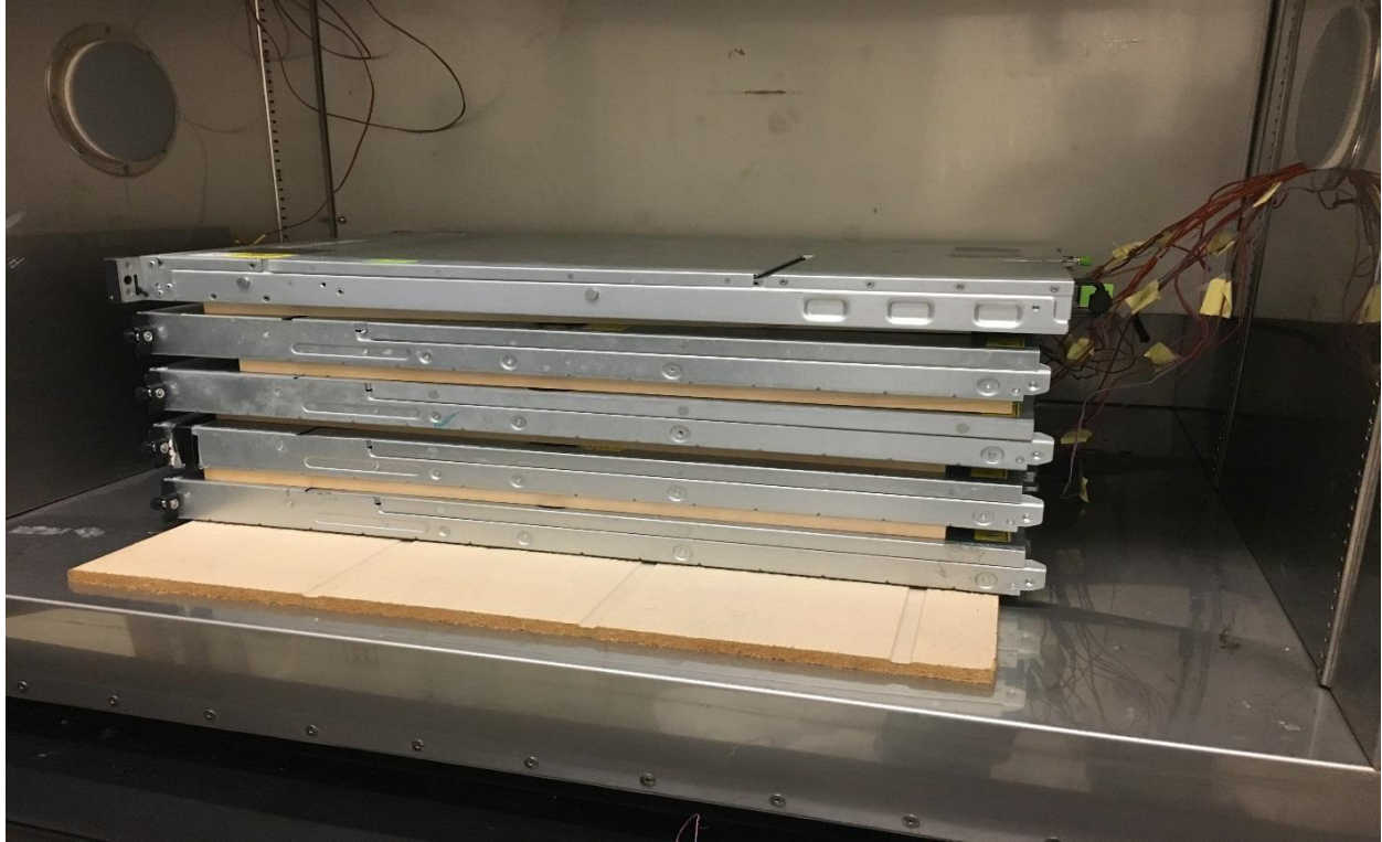
Fig 12: Server in rack placed inside the environmental chamber.
