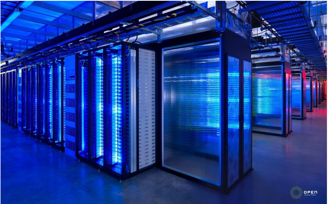
Fig 1: Open compute project data center [7]
