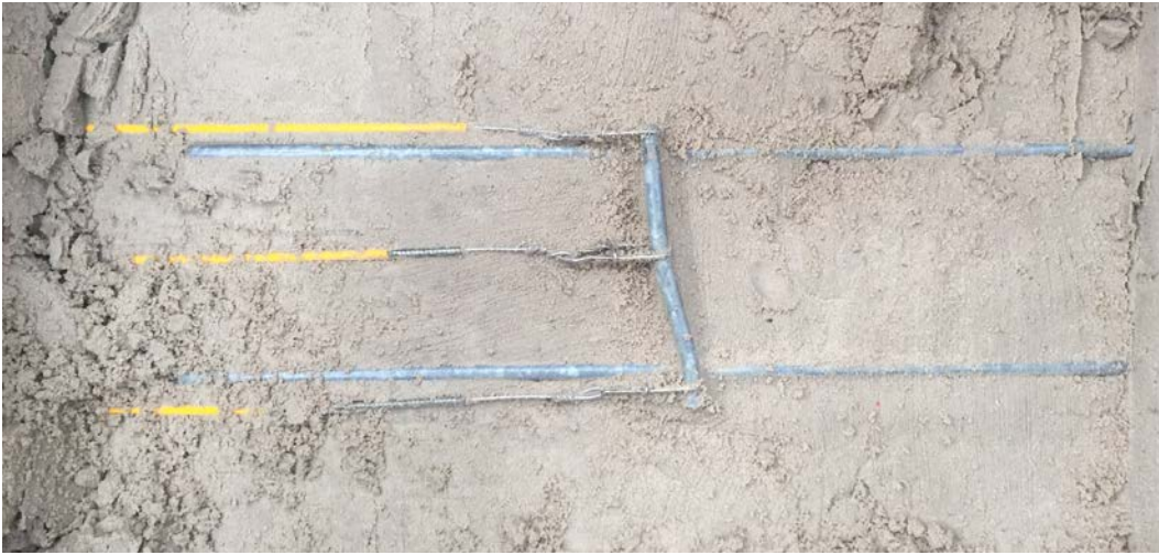
Photograph 4-4 Weld Failure MW71 x MW71 – 100 x 300
