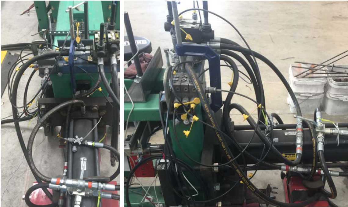
Photograph 3-10 Hydraulic Flow Control System
