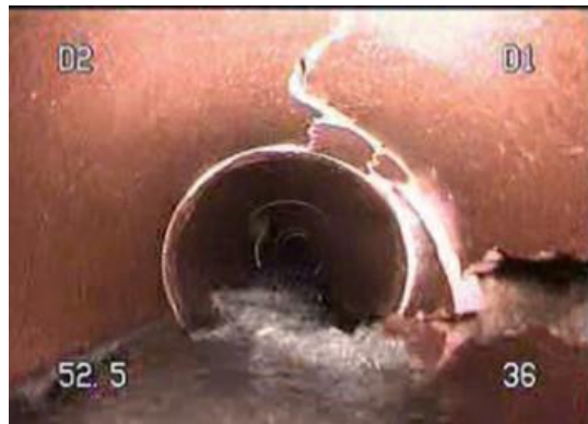
Figure 1-15 Broken and fracture-multiple are detected through CCTV
