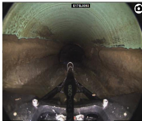
Figure 4-52 Significant defects in line 49 (DAE)
