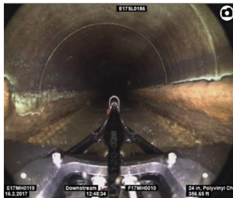
Figure 4-55 Significant defects in line 53 (DAE)
