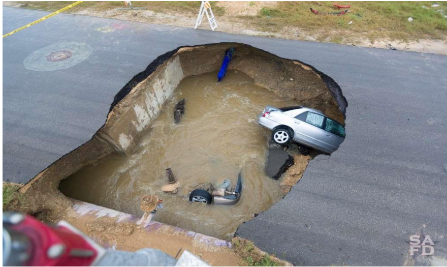
Figure 1-1 Road collapsing in San Antonio after a sewer main ruptured underground (San Antonio Express-News 2016)
