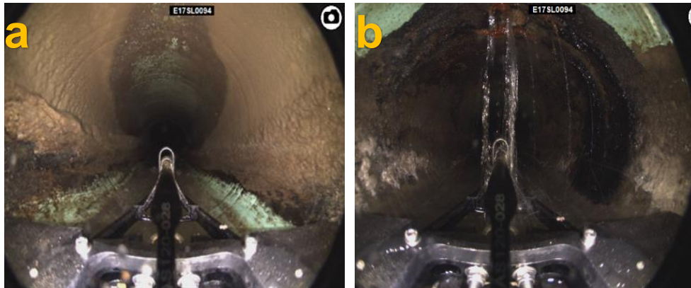
Figure 4-51 Significant defects in line 48. It shows (a) DAE and (b) IRJ
