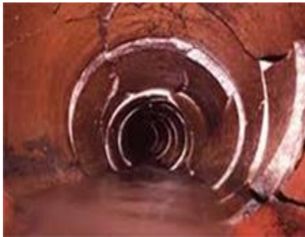
Figure 1-6 Longitudinal and circumferential fractures in vitrified clay pipes
