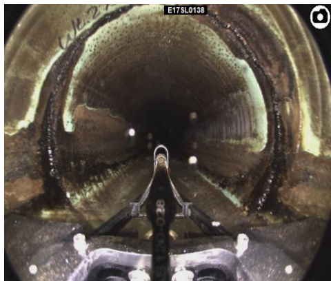
Figure 4-50 Significant defects in line 47 (DAG and DAE)
