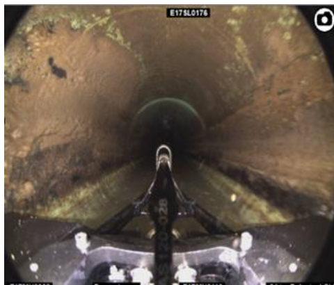
Figure 4-46 Significant defects in line 39 (DAE)
