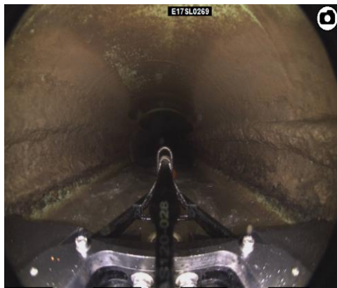
Figure 4-49 Significant defects in line 46 (DAE)
