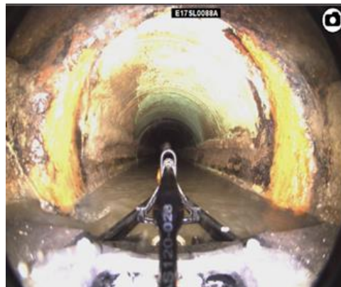
Figure 4-53 Significant defects in line 50 (DAG and DAE)
