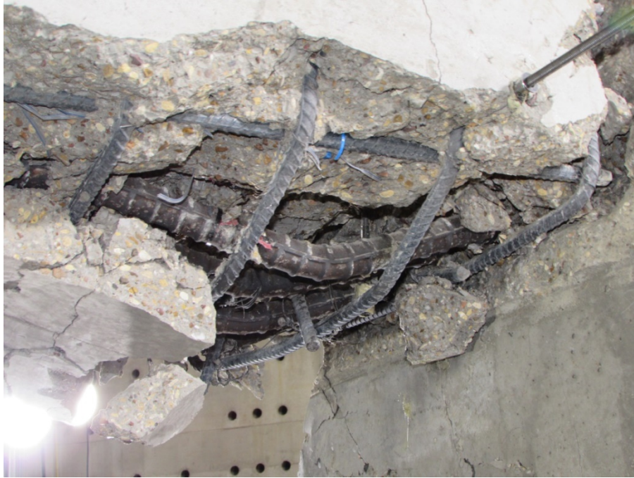
Figure 3.31 Buckled longitudinal reinforcement for RC-SP-NL
