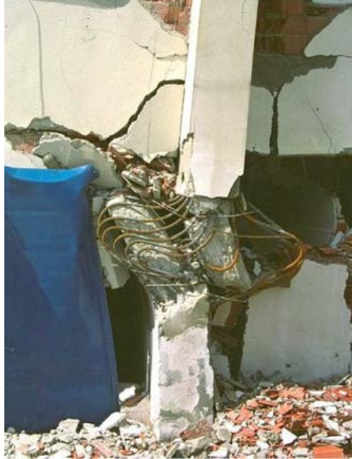
1.3 Column shear failure (Moehle et al., 2008)
