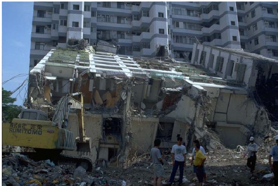
1.2 Building collapse due to story mechanism (Chi-Chi, Taiwan, 1999)
