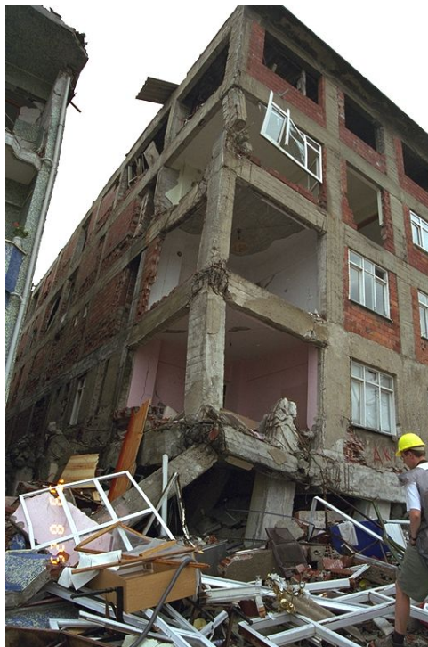
1.4 Joint shear failure
