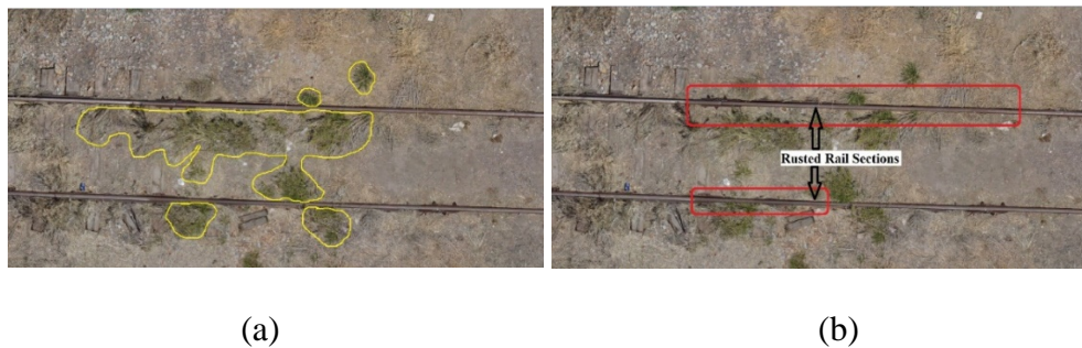
Figure 4-53. Rail Track Condition Assessment (a) Vegetation Encroachment and (b) Rusted Rail Sections
