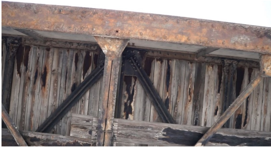
Figure 4-57. Under-bridge View Displaying Missing Rivets, Rotten and Rusted Bridge Elements
