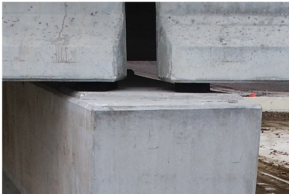
Figure 4-47. Zoomed in Images Depicting the Condition of the Bearings and Pier Cap
