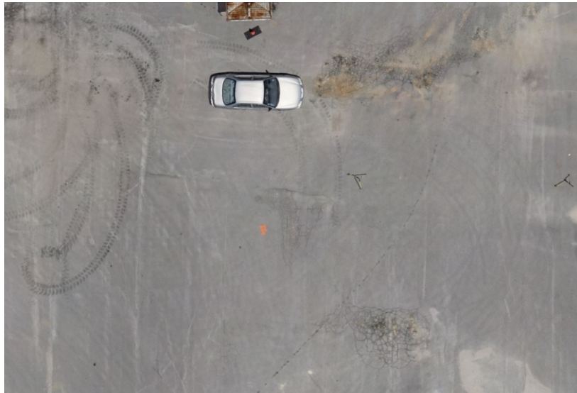
Figure 4-24. Multiple Pavement Distress
