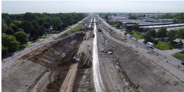
Figure 2-31. View from the UAV Used for Construction Site Monitoring (Brooks et al. 2015)
