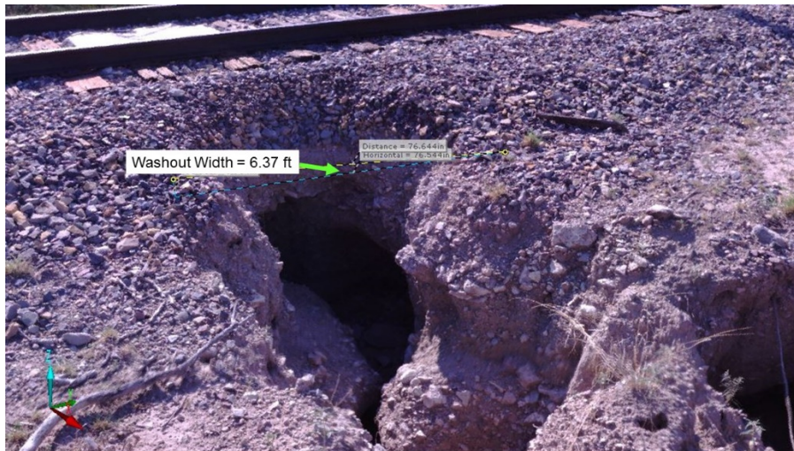
Figure 4-64. Washout Width Measured Using Data Collected from Terrestrial LiDAR
