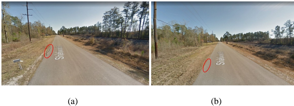
Figure 5-8. Google Map Street Images of Sherwood Dr Looking towards Tram Rd, Beaumont, Texas Captured in January 2013 (a) Sealed Cracks (b) Developing Cracks (Map data © 2018 Google)
