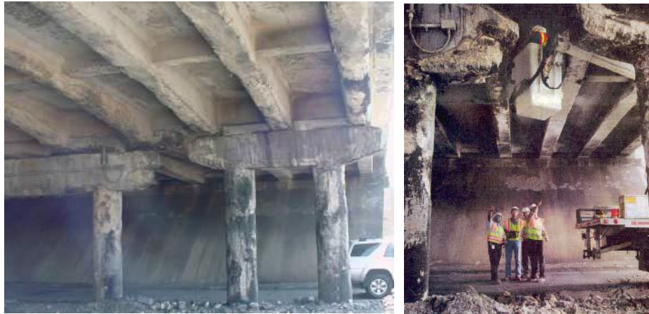
Figure 3-6 Fire Damage on Old SH183 over MacArthur
