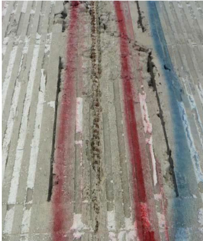
Figure 2-13 Exposed reinforcement in wall outline in red
