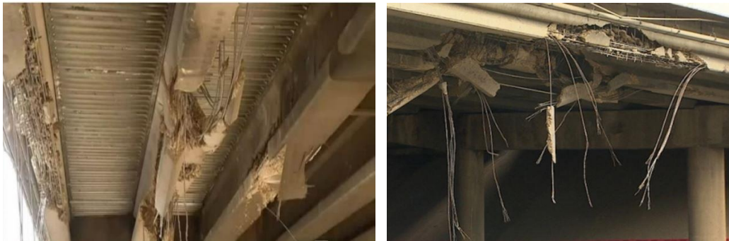
Figure 3-1 Impact Damage on Old SH183 over Loop 12
