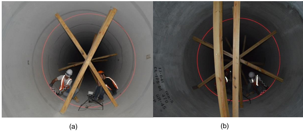
Figure 2-22 Deformed stulls at the backfill with stulls construction stage: (a) vertical stulls remained after pipe deflection, (b) deformed vertical stulls remained
