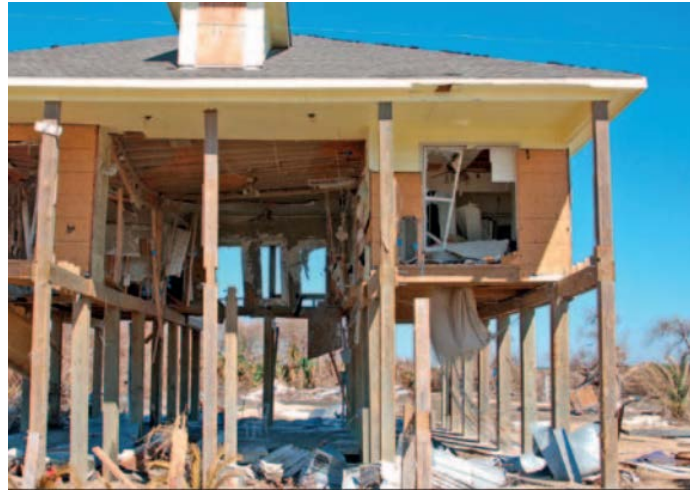
Figure 3.2 Failure of floor system but major framing system remains intact (Source: FEMA P-55 II, 2011)
