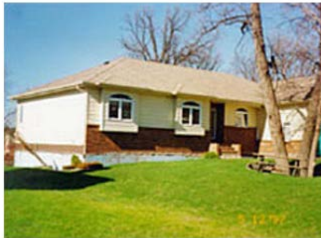
Figure 2.10 Failure of Lightweight building with a Dry- Floodproofed Basement, lifted out of the Ground by Buoyancy forces during a flood (Source: USACE)
