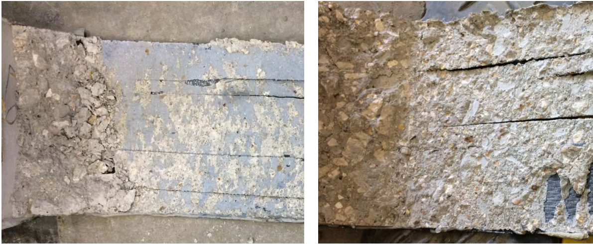
Figure 5- 24: Debonding of the FRP layer
