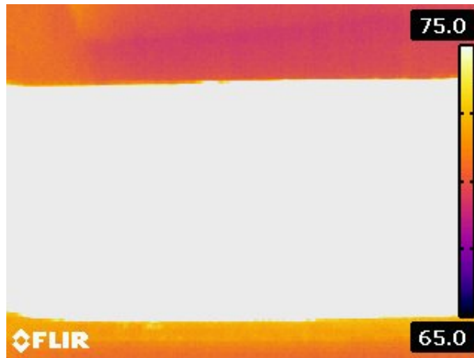
Figure 4- 29: Infrared camera picture of debonded FRP layer
