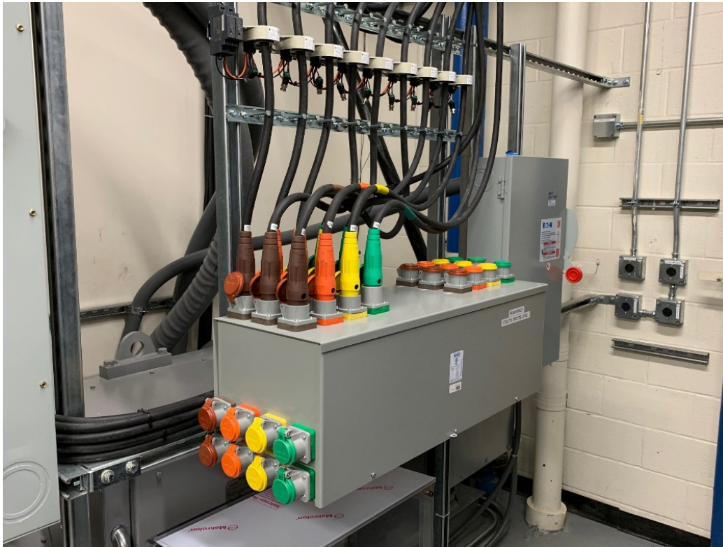
Figure 4.6: MG or utility grid power distribution box.
