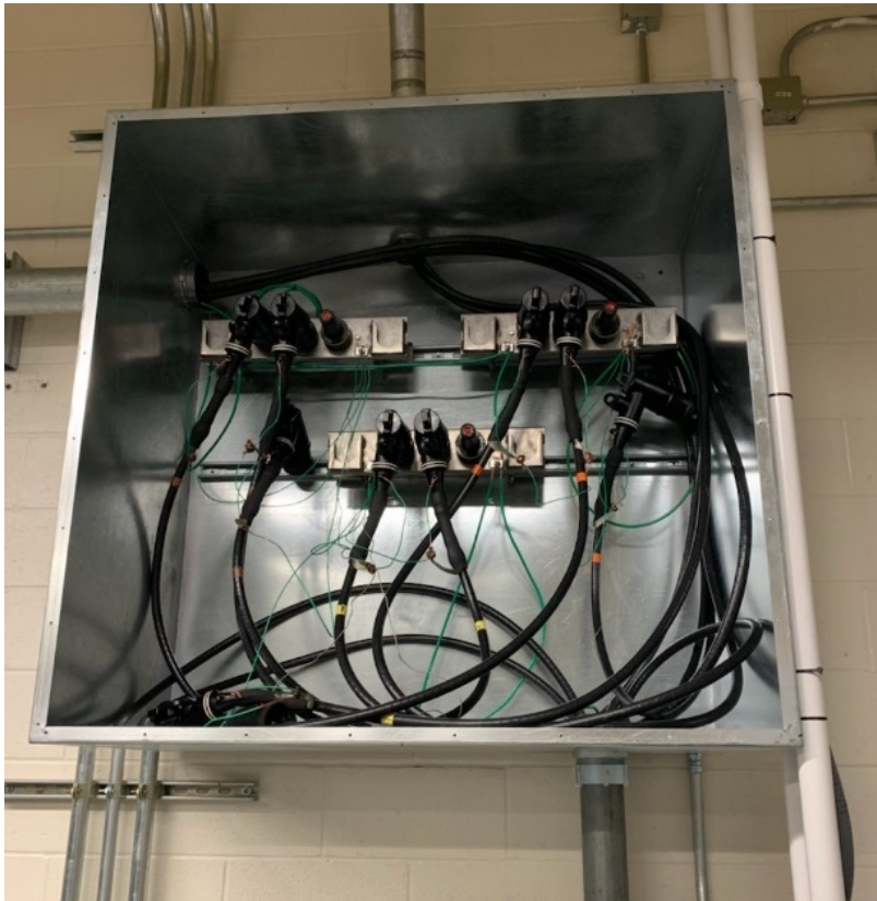
Figure 4.12: Photograph of the 4160 VAC distribution box installed in the laboratory. Each of the three blocks of connectors makes up a respective voltage phase. In each of the three blocks is three connectors. One is the input from the MV6000, one is the output to the 4160 VAC to 480 VAC transformer, and the third is the output to the 18 phase transformer/rectifier.
