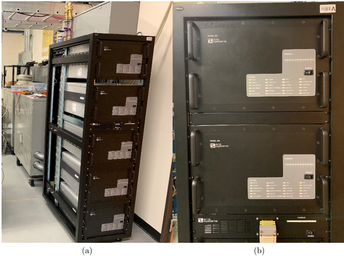
Figure 4.7: Photograph showing the installation of the two – 50 kW TDK Lambda power supplies used to convert 480 VAC to 12 kVDC (upper two supplies are the two 12 kVDC supplies and the lower three are the 1 kVDC supplies that will be discussed later.)
