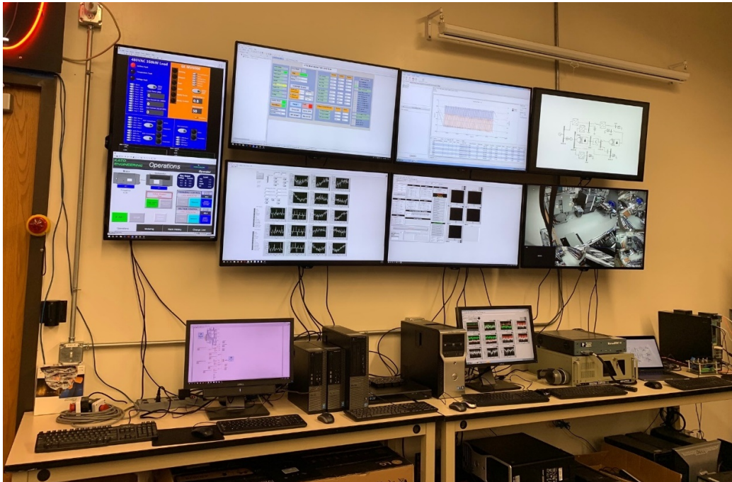
Figure 4.27: Photograph of the operator control center used to control the MVDC testbed.
