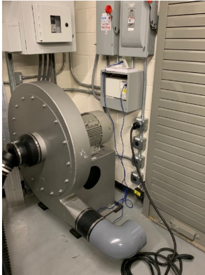
Figure 4.16: Photograph of the 15 HP blower, variable frequency drive, and braking resistor used to apply forced air cooling to the 4160 VAC transformer and 6 kVDC rectifier.
