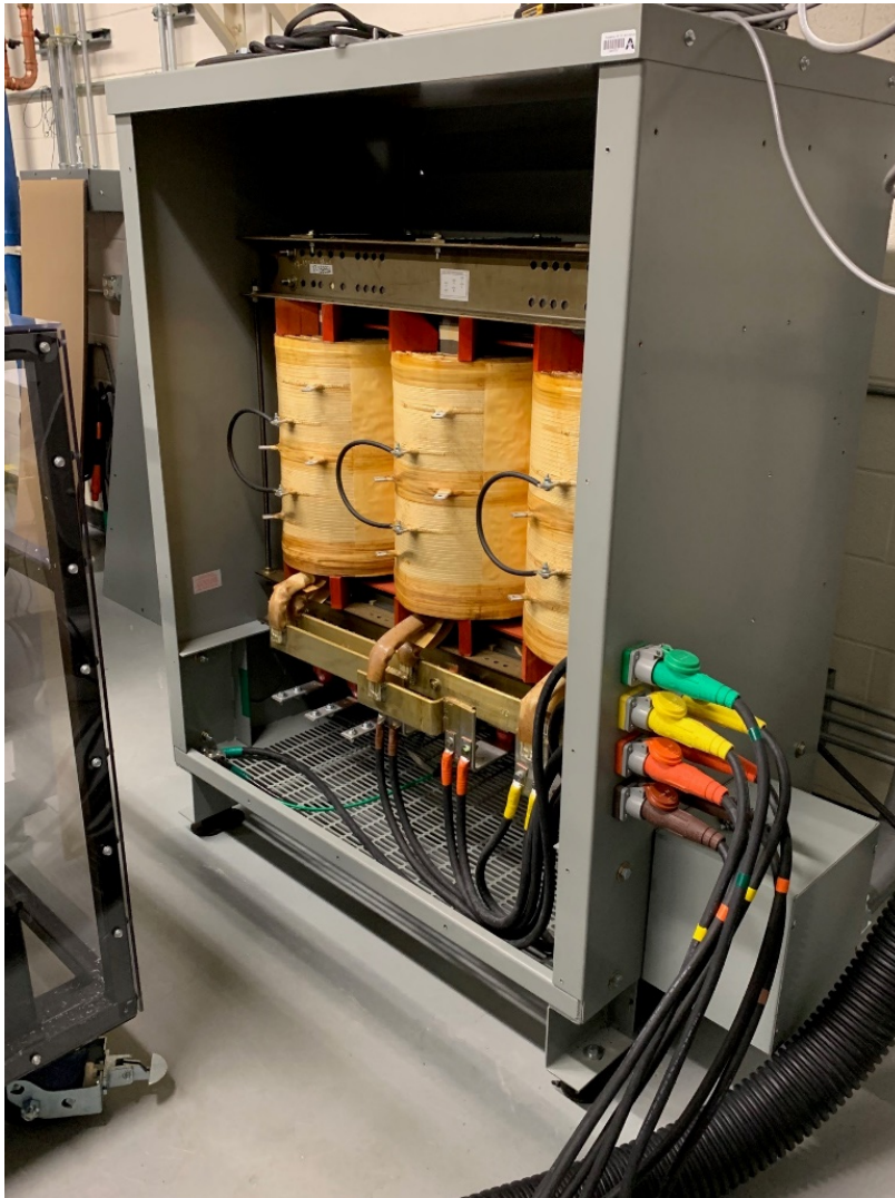
Figure 4.13: Photograph of the 500 kVA - 4160 VAC / 480 VAC step down transformer installed in the laboratory.
