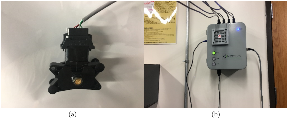
Figure 2.27: Photograph of a Nexceris Li-Ion Tamer ® off-gas sensor (a) and the data acquisition system installed at UTA (b).
