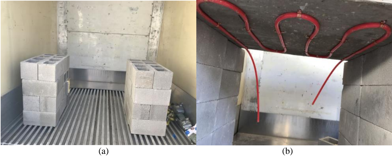
Figure 4- 1 (a) Concrete block support for 4” by 3” slab, (b) PEX Pipe network secured to base of slab
