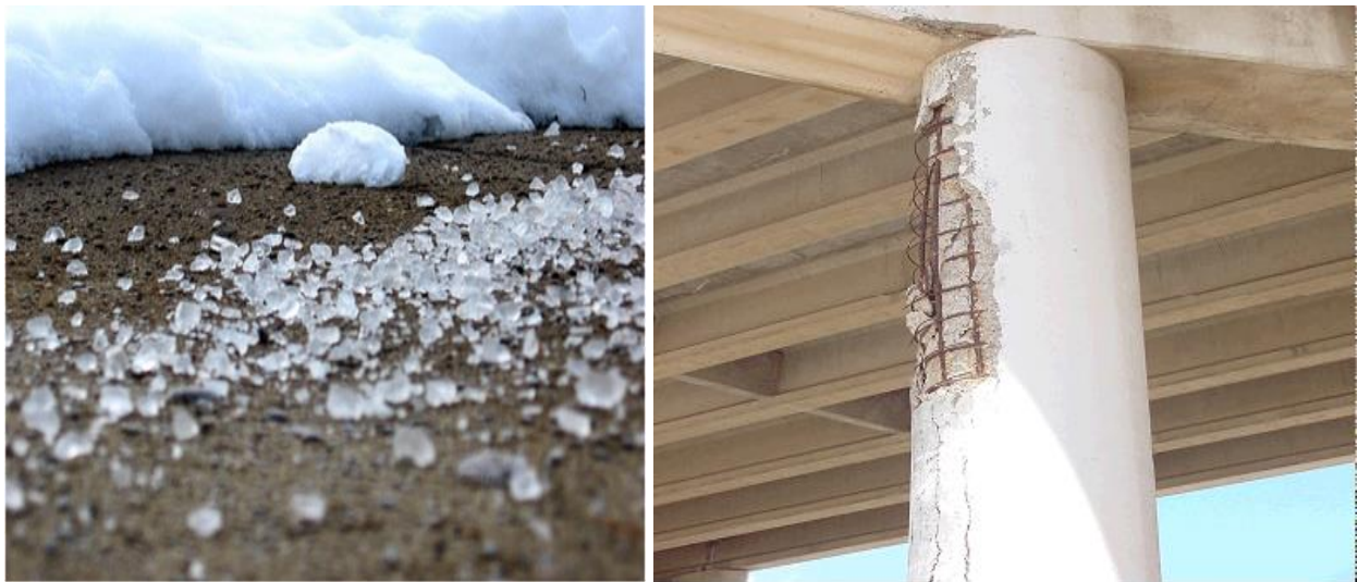
Figure 1- 3 (a) De-icing Salt causing Pits (Ryan Kartchner Concrete Construction) (b) Column deterioration from chemical solution contamination (C. Michael Lee, 2017)
