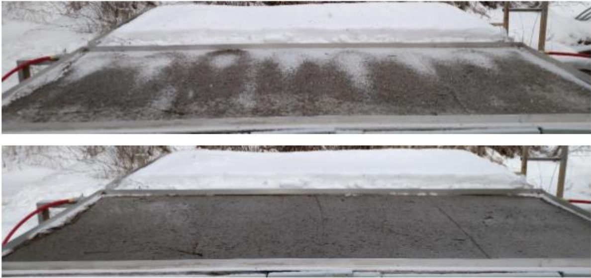
Figure 2- 8 Photographs of the heated bridge deck at 9:15 (top) and 10:00 (bottom) on the morning of 2/24/2014 (Bowers, 2016)
