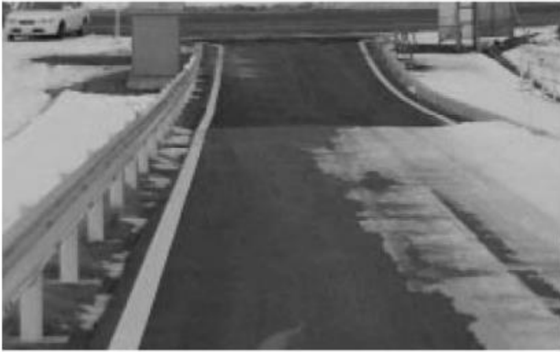
Figure 2- 16 Result of deicing installation work on a part of road (Yu, et al, 2017)
