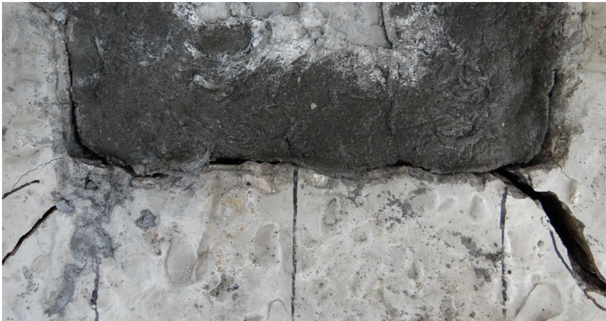
Figure 4- 27 Vertical deformation of the central repair slab and cracks propagating from the corner of the repair slab into the supporting outer slab.
