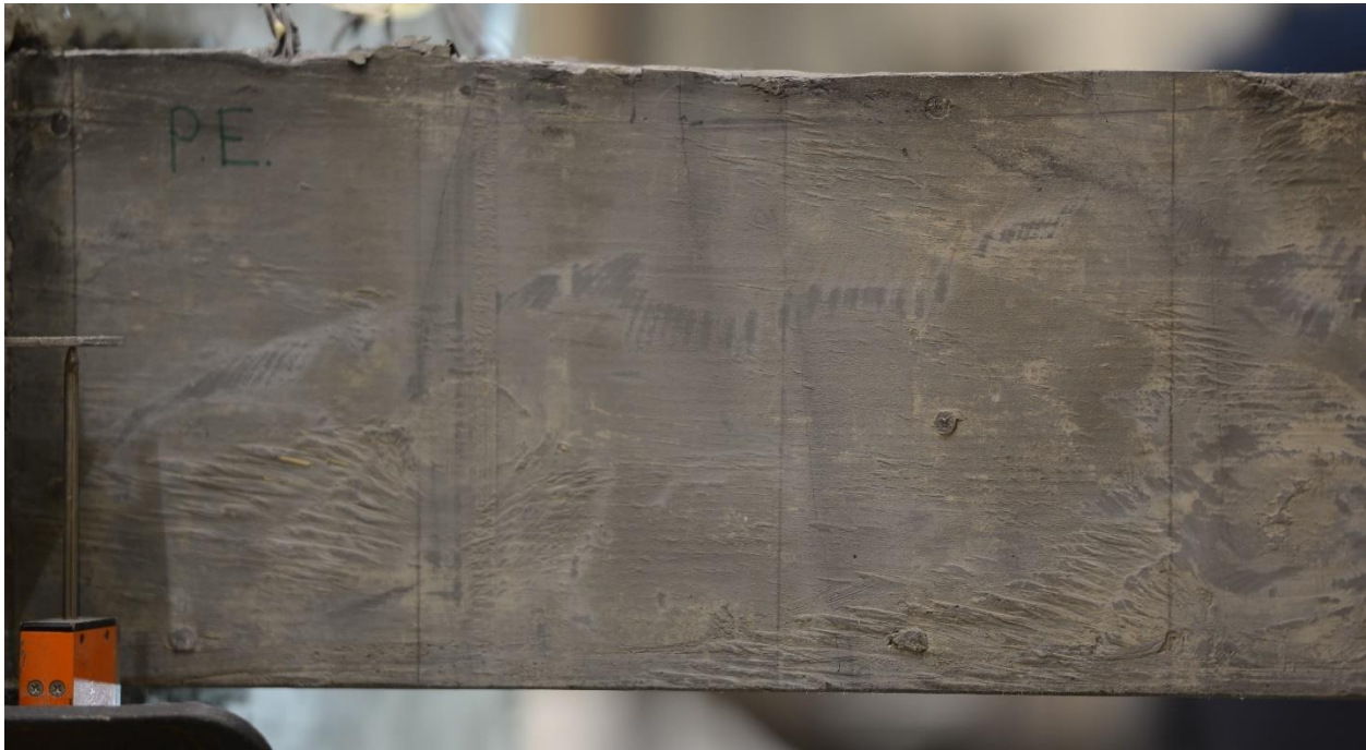
Figure 10- 1 Shrinkage cracks developed at the location of the BFRP stirrups prior to testing
