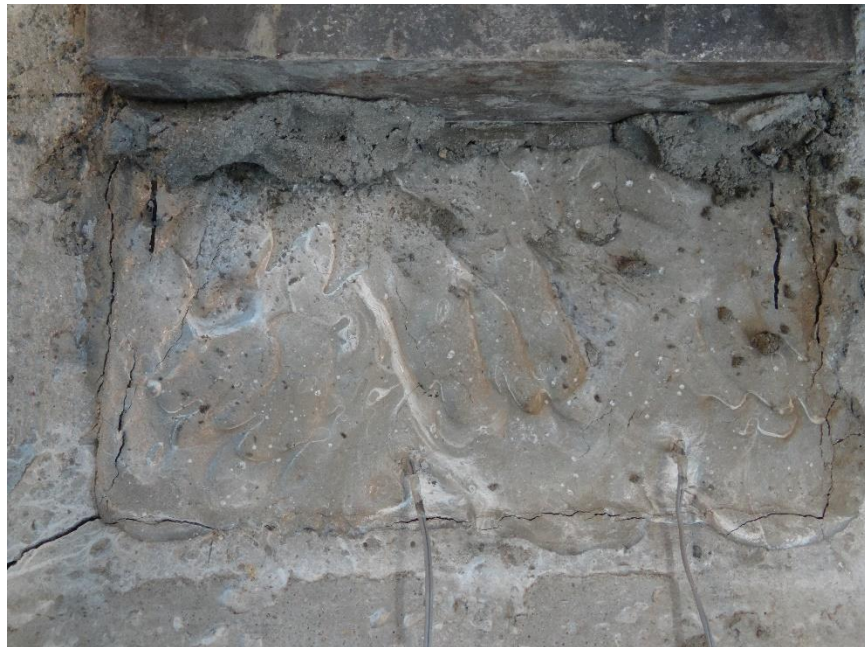
Figure 4- 18 Cracks observed at the interface between repair cast in place PC and the old concrete (outer hollow slab) post peak.
