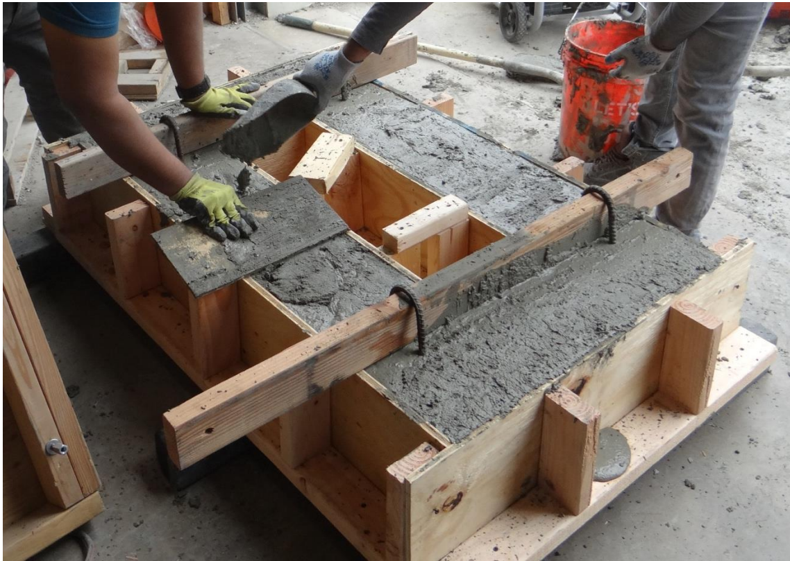
Figure 3- 17 In-lab concrete mixing is shown in top photo and casting for the outer hollow slab is shown in the bottom photo.
