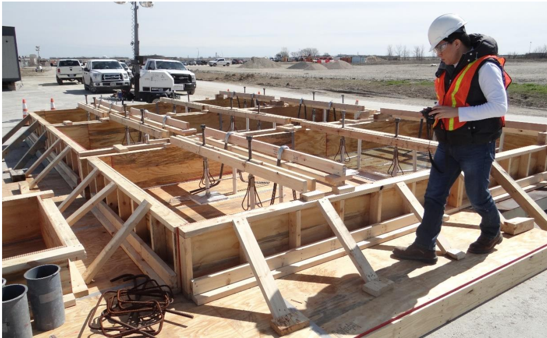
Figure 5- 5 Formwork the casting of precast UHP-FRC panels with the leveling screws installed
