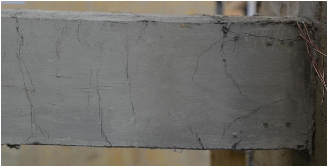
Figure 9- 32 UHP-FRC #2 at 5.0% drift
