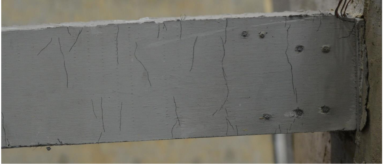
Figure 9- 14 UHP-FRC #1 at 4.0% drift
