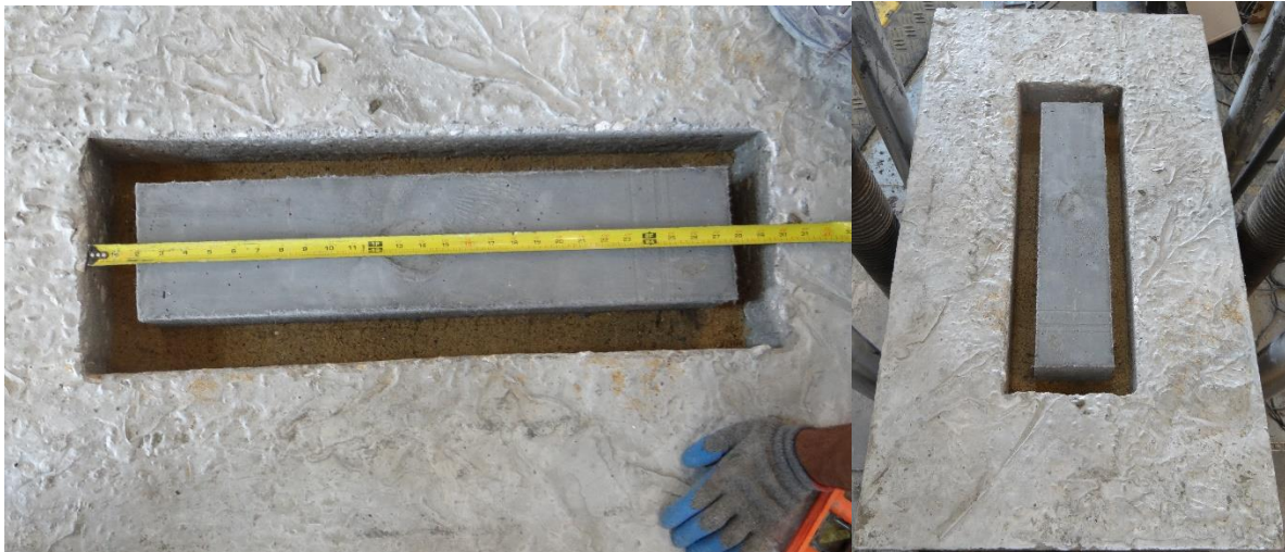
Figure 3- 27 Placement of precast UHP-FRC panel into hollow portion of outer hollow slab.
