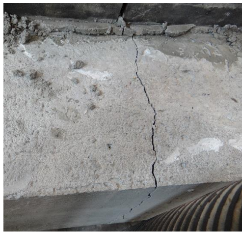
Figure 4- 20 Cracks seen at mid-span of the longer dimension extending throughout the depth of the slab.
