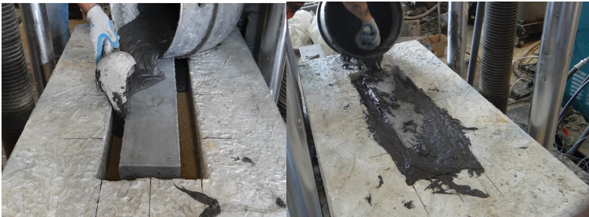
Figure 3- 28 Cast in place UHP-FRC between the precast UHP-FRC slab and outer hollow slab.
