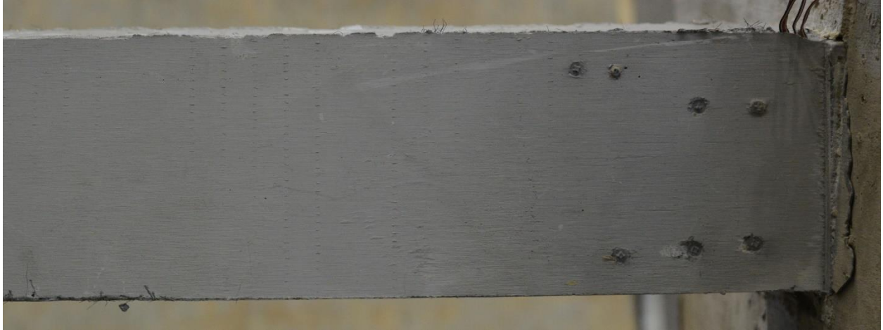
Figure 9- 10 UHP-FRC #1 at 1.75% drift
