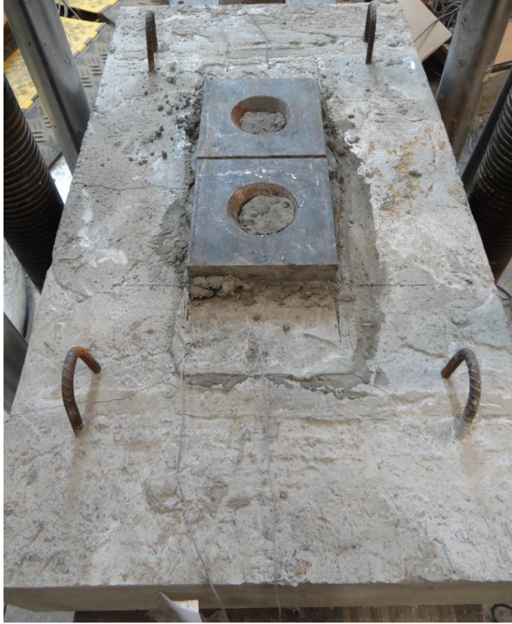
Figure 4- 19 Cracks seen in the outer slab initiating from the interface with the loading plates.
