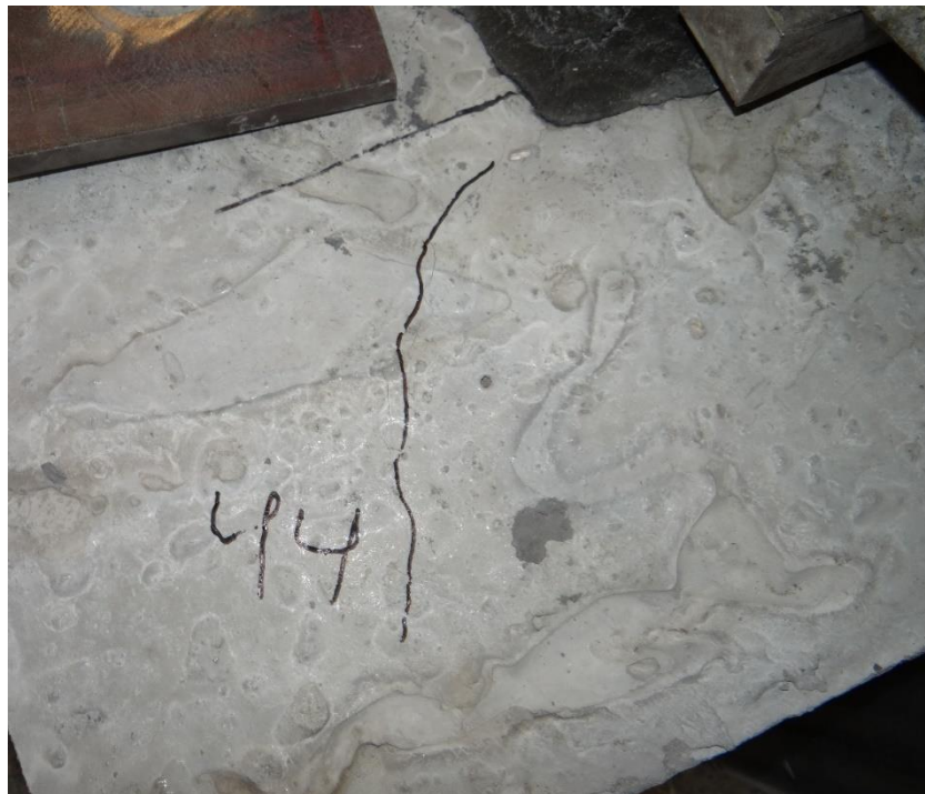
Figure 4- 25 Initiation of cracks from the corner of the repair joint at 44 kips of the post peak vertical load.
