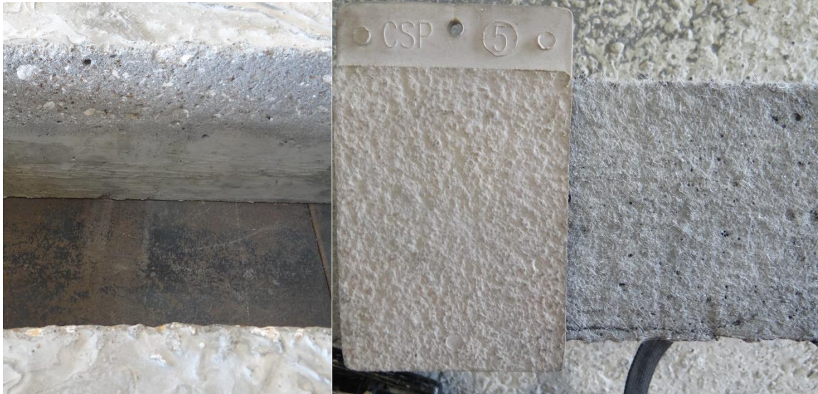
Figure 3- 25 Roughened surface of inner wall of the outer hollow slab with a depth of 4 inches with a roughness level of CSP 5.
