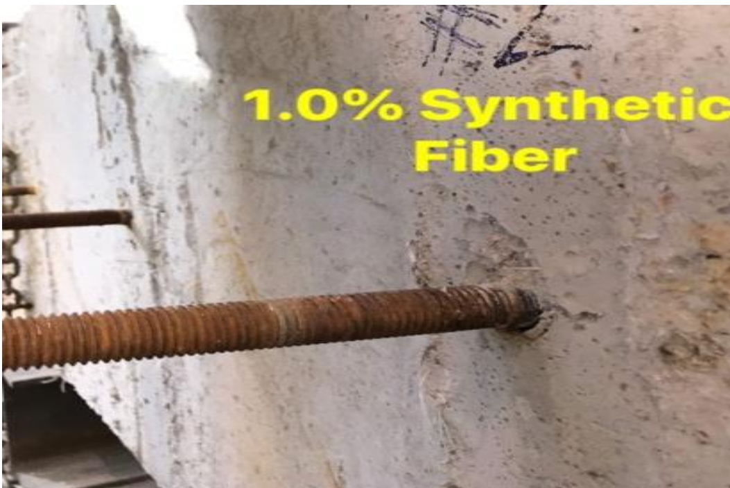
Figure 36: Steel failure preceded by concrete spall for 1.0% synthetic fiber
