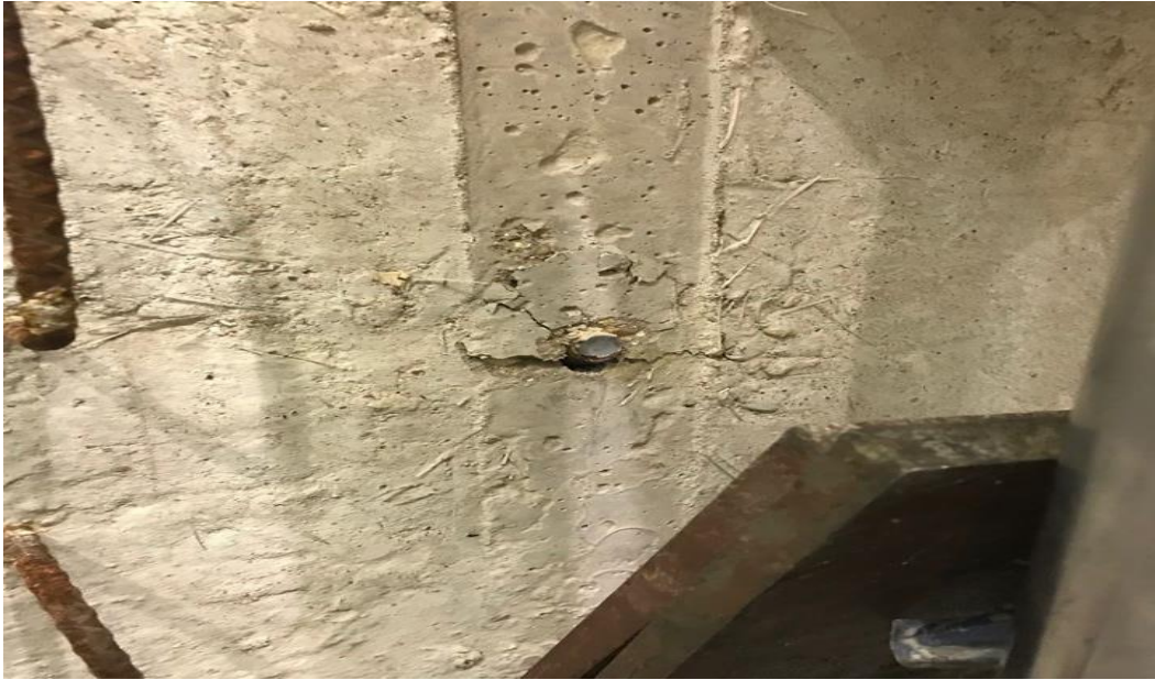
Figure 21: Steel failure proceeded by concrete spall for (0.50% Polypropylene Fiber) specimen
