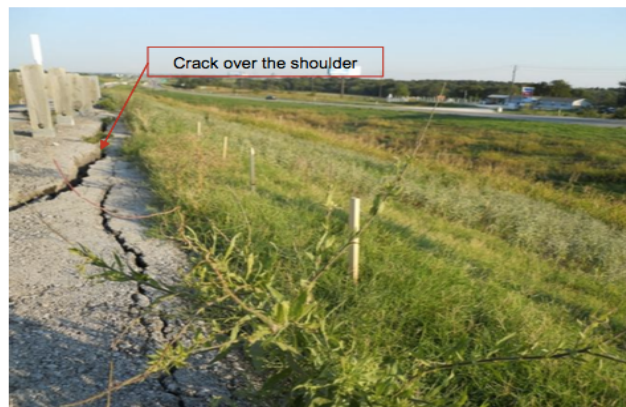
Figure 3- 2 Shoulder cracks observed at crest of US 287 slope (Khan, 2013)
