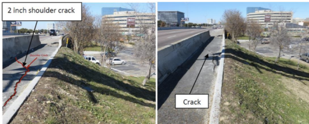
Figure 3- 11 Failure photos on shoulder of I-35 (Tamrakar, 2015)
