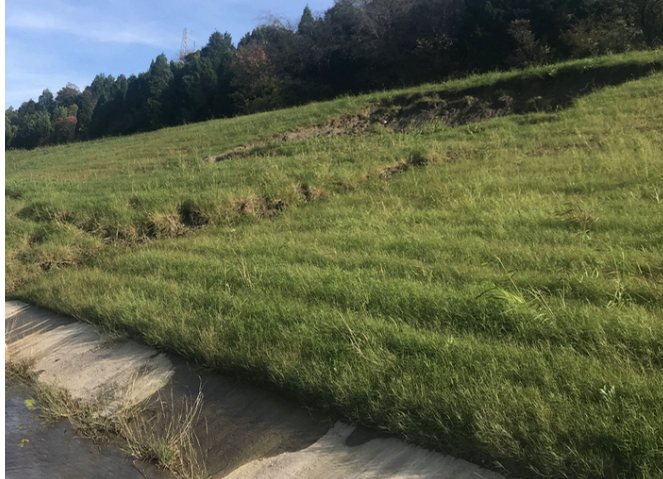
Figure 2- 2 Slope Failure off I-20 east bound near Clark Rd.
