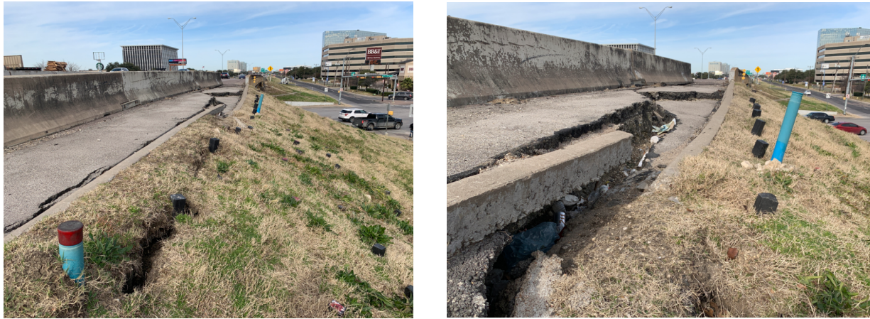
Figure 4- 15 Condition of I-35 slope near Inclinometer 1
