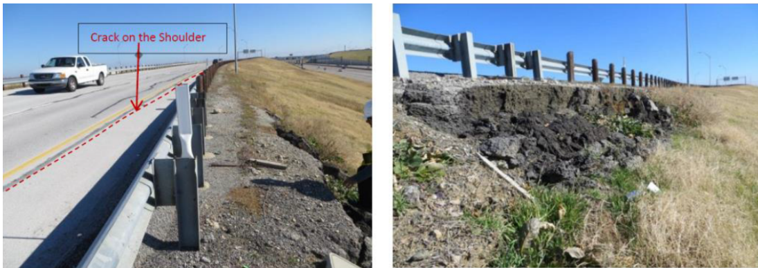
Figure 3- 19 Slope failure photos at SH-183 (Tamrakar, 2015)
