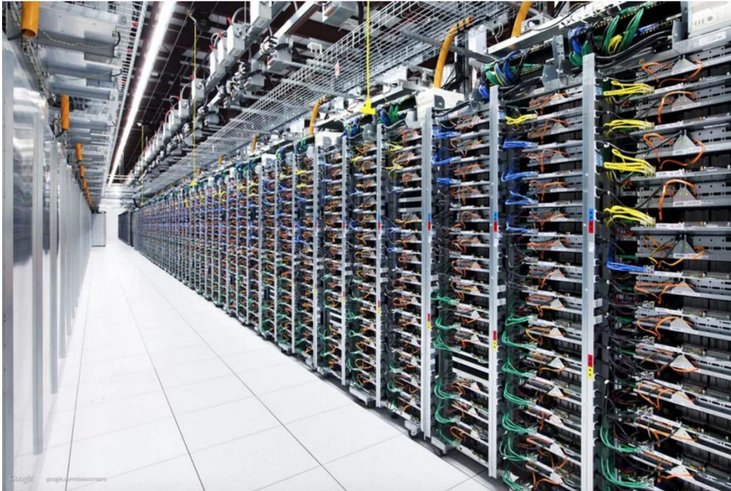
Fig 1-1: Typical Data Center
