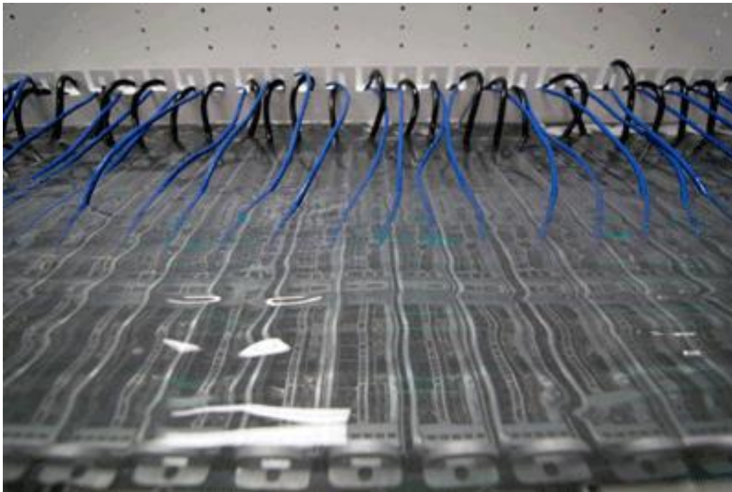
Figure 3 Dielectric Fluid Immersed Server
