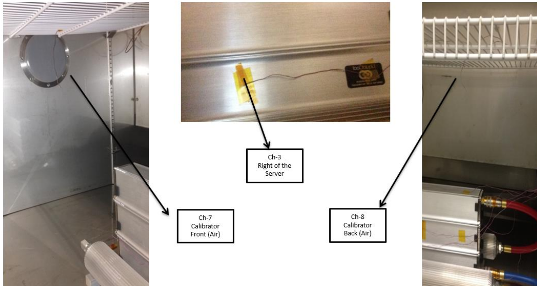
Figure 5-2 Back side of the server
