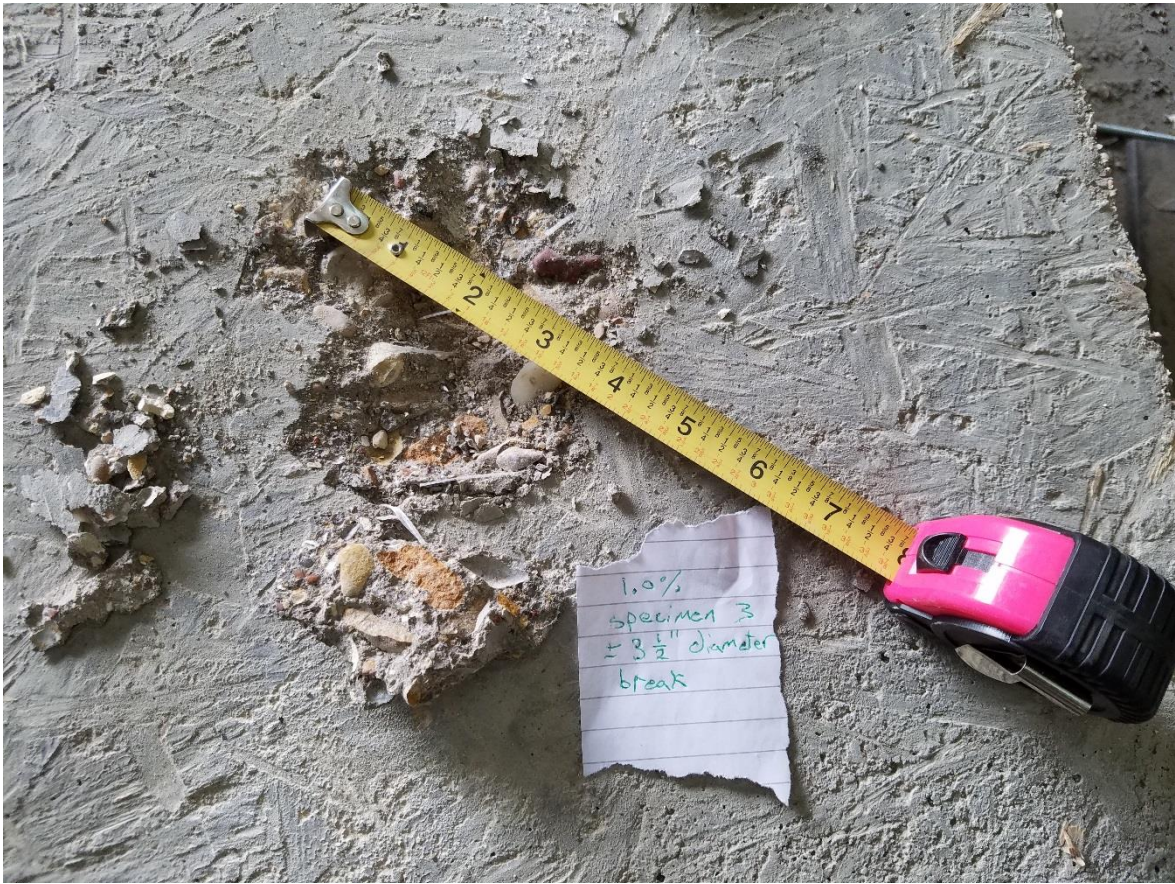
Figure 44: 1.0% Fiber - Specimen 3 Failure
