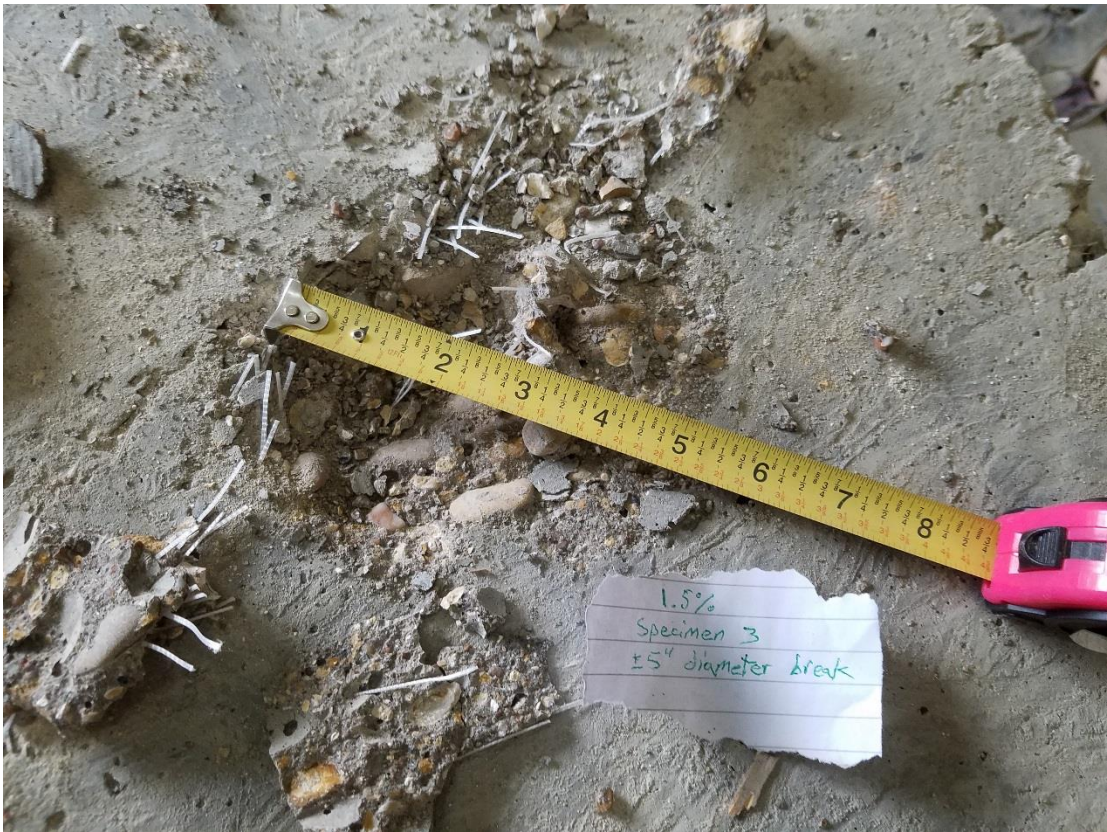
Figure 49: 1.5% Fiber - Specimen 3 Failure
