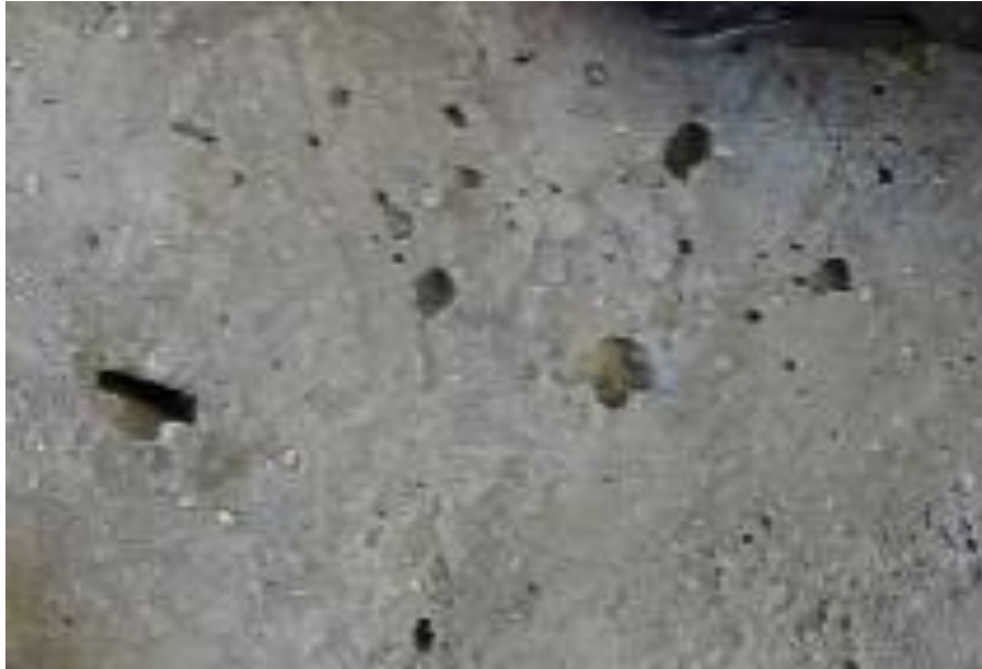
Figure 27: Bug holes seen on the surface of the 1.5% mixture specimen
