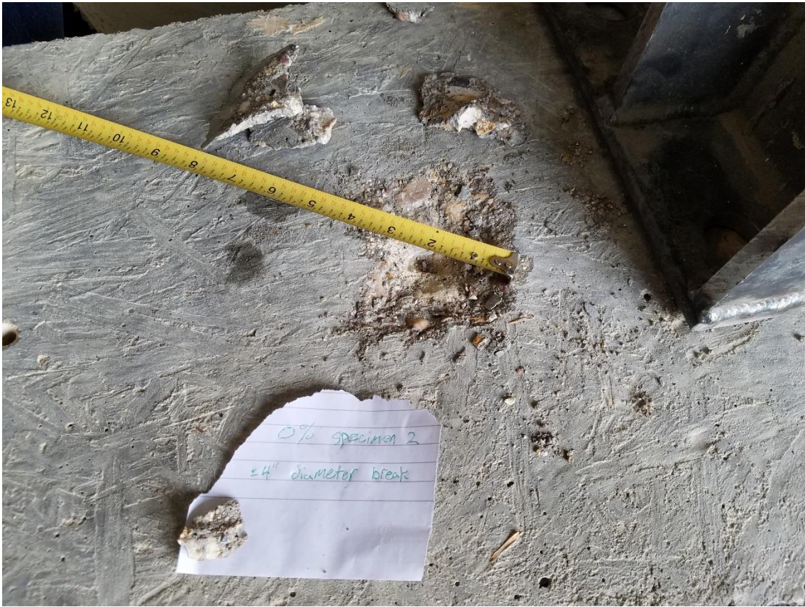
Figure 33: 0.0% Fiber - Specimen 2 Failure
