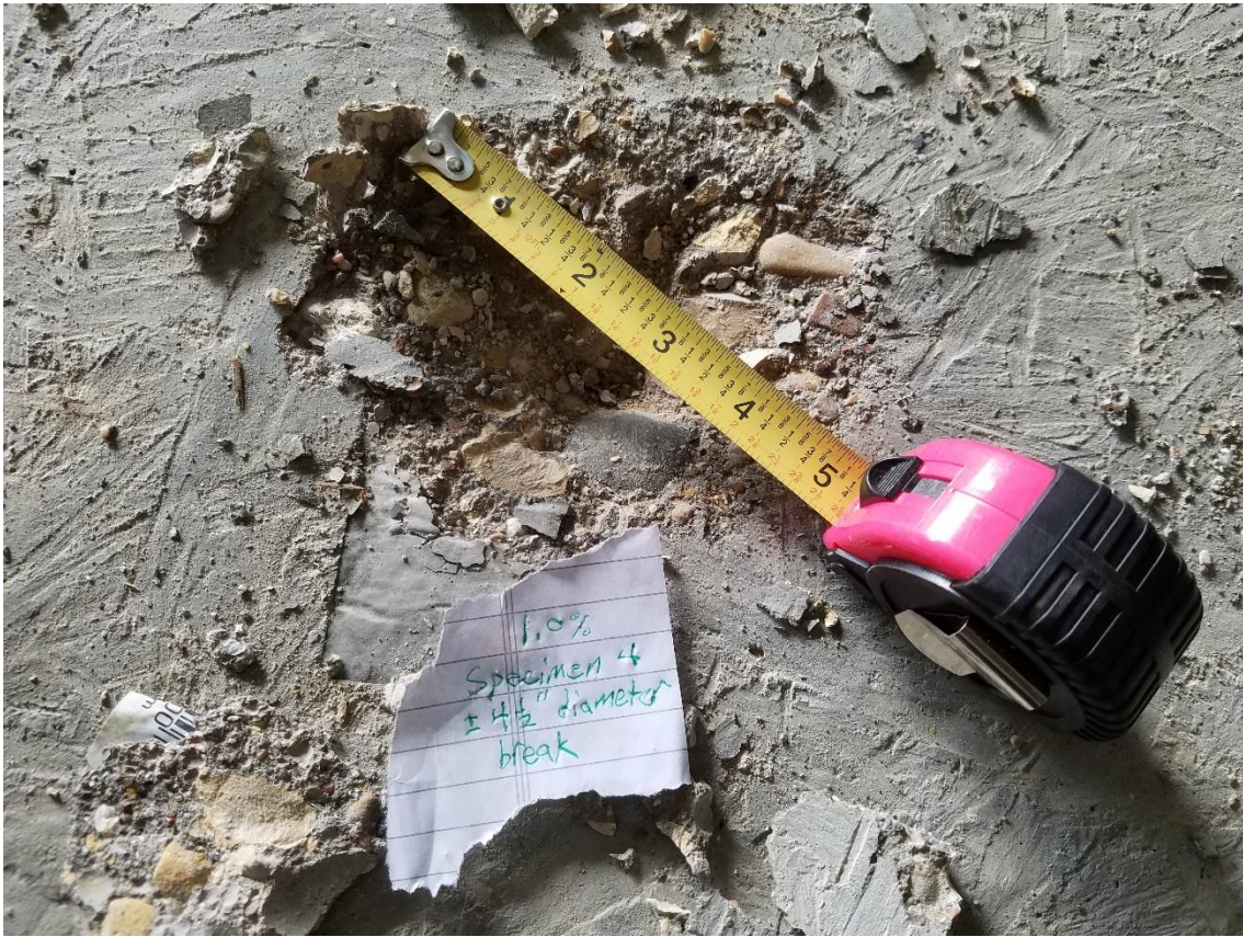
Figure 45: 1.0% Fiber - Specimen 4 Failure
