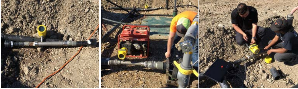
Figure 5-34 Flow meter installation
