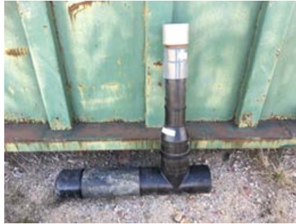
Figure 5-22 Leachate collection sump
