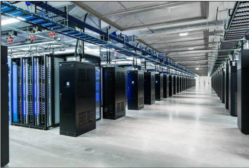
Figure 1-1 Facebook's Data Center
