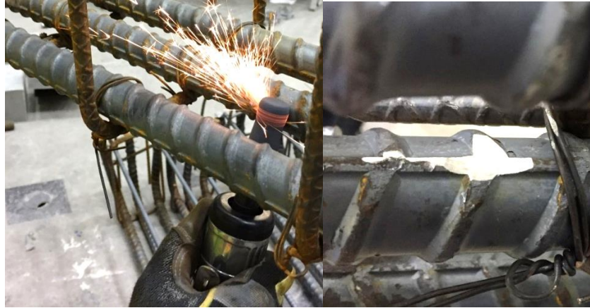
Figure 8 Typical photo of grinding the surface of the rebars with an Air Die Grinder
