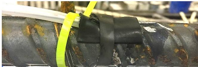
Figure 15 Typical photo of steel strain gage protected with a polyethylene tube
