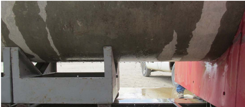
Figure 5-65 - Leakage on wall of the left concrete pipe
