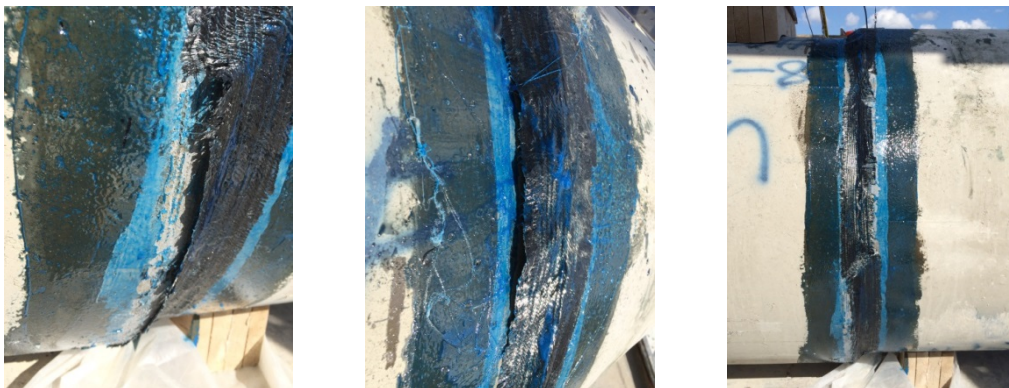
Figure 5-22: Slipped out CFRP fabric from assembled pipes on TW36-3W-2H
