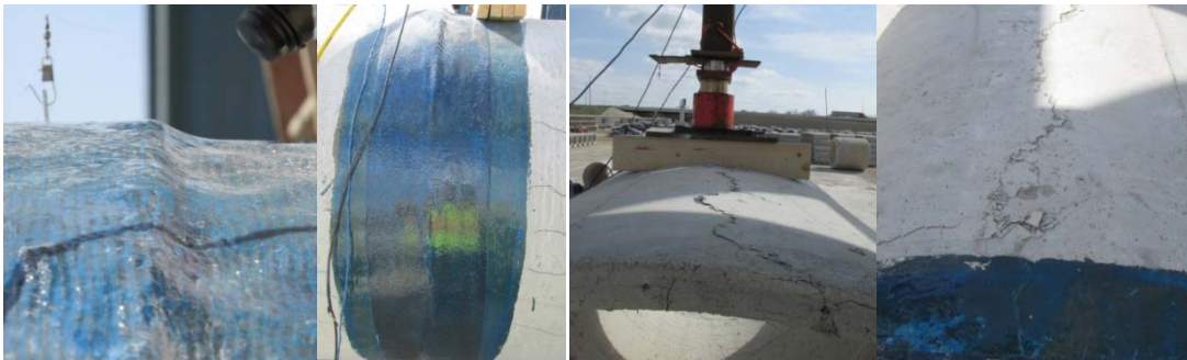
Figure 5-17: Concrete fracture of TW60-12W-24H
