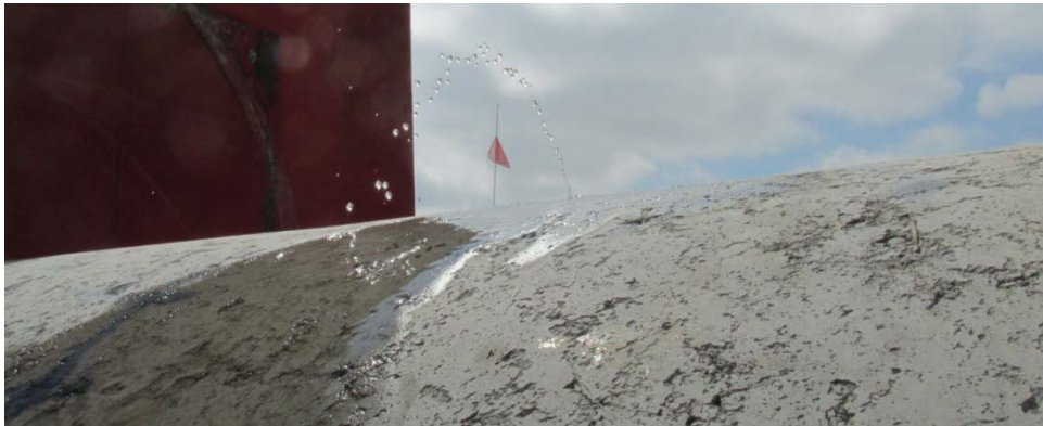
Figure 5-64 - The 2 nd leakage on the mid-wall of the concrete pipe
