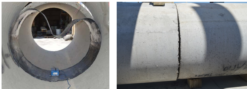
Figure 5-35 - CFRP coupler of 0.0625 inch failed; no visible damage on concrete pipe
