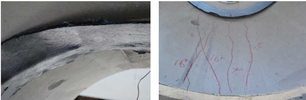
Figure 5-45 - Collapse of the CFRP internal coupler for TW-54-0.25 specimen
