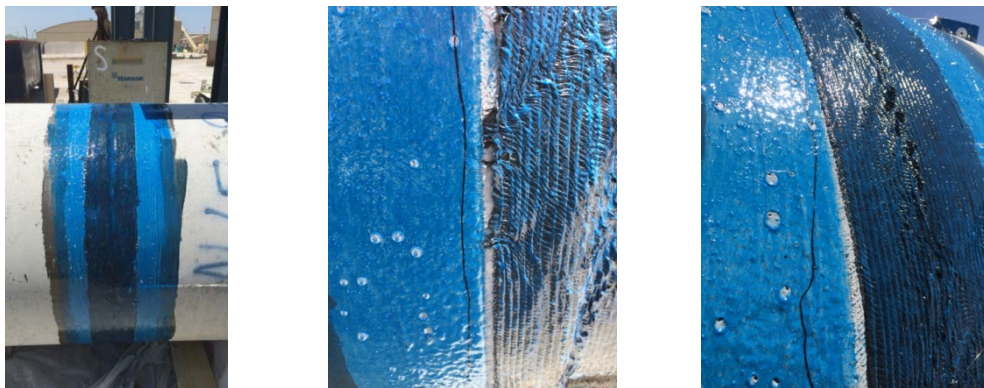
Figure 5-20: Slipped out CFRP fabric from assembled pipes on TW36-6W-1H
