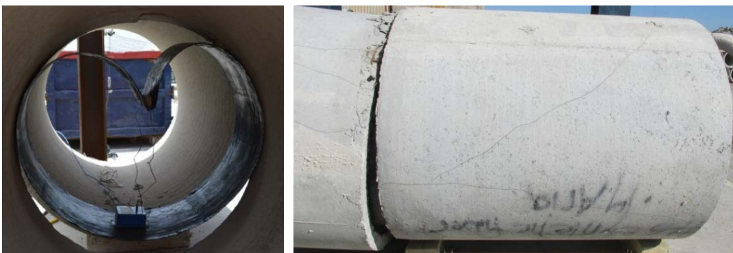
Figure 5-37 - Internal joint system failed for TW-36-0.125
