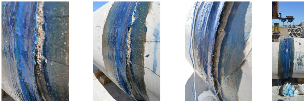
Figure 5-13: Flaking concrete of TW36-3W-24H with Dirty
