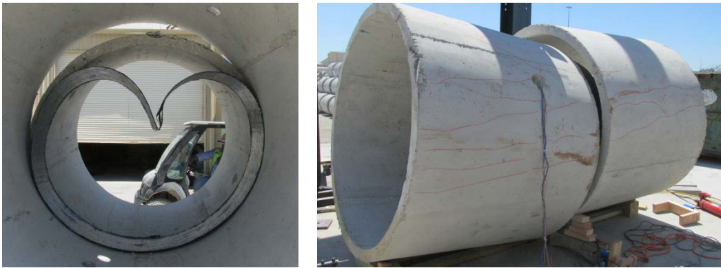
Figure 5-44 - Collapse of the CFRP internal coupler for TW-54-0.1875 specimen
