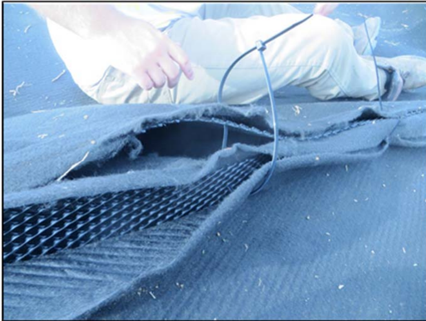
Figure A.298: Placing a zip-tie at the intersection of two (2) geocomposite drain sheets.
