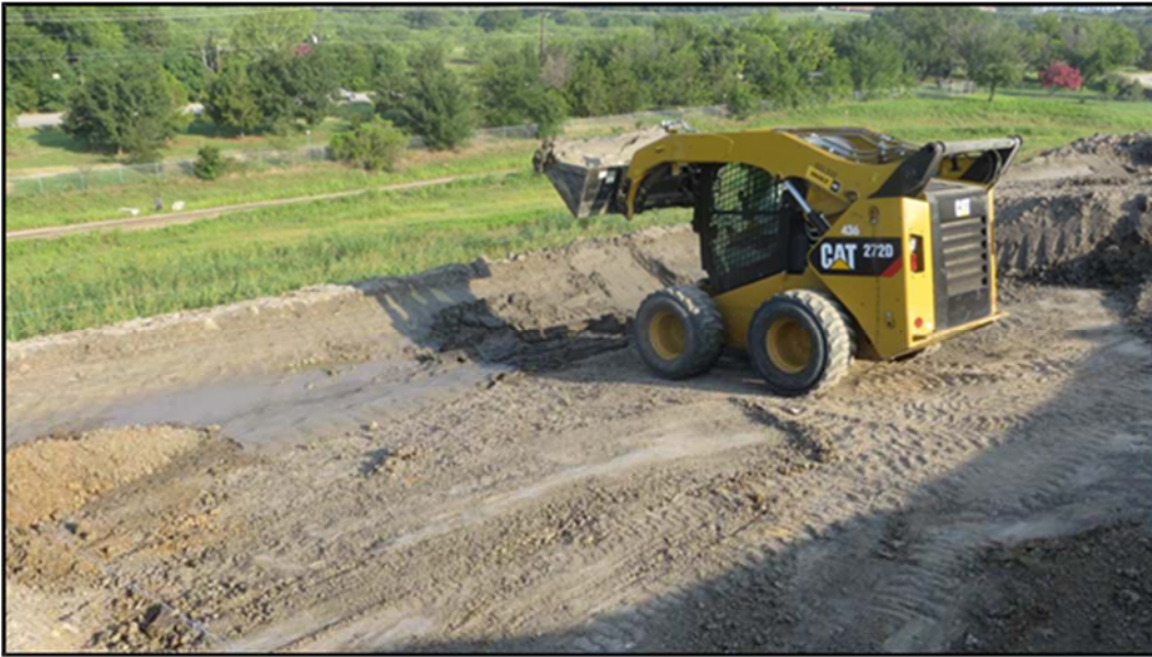
Figure A.253: Removal of water and damp soil from an inclined section by a skid steer.
