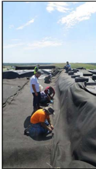
Figure A.143: Joining the geotextiles to the geocomposite drain along a sidewall.
