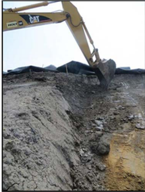
Figure A.256: Removal of the construction ramps in an inclined section by an excavator.
