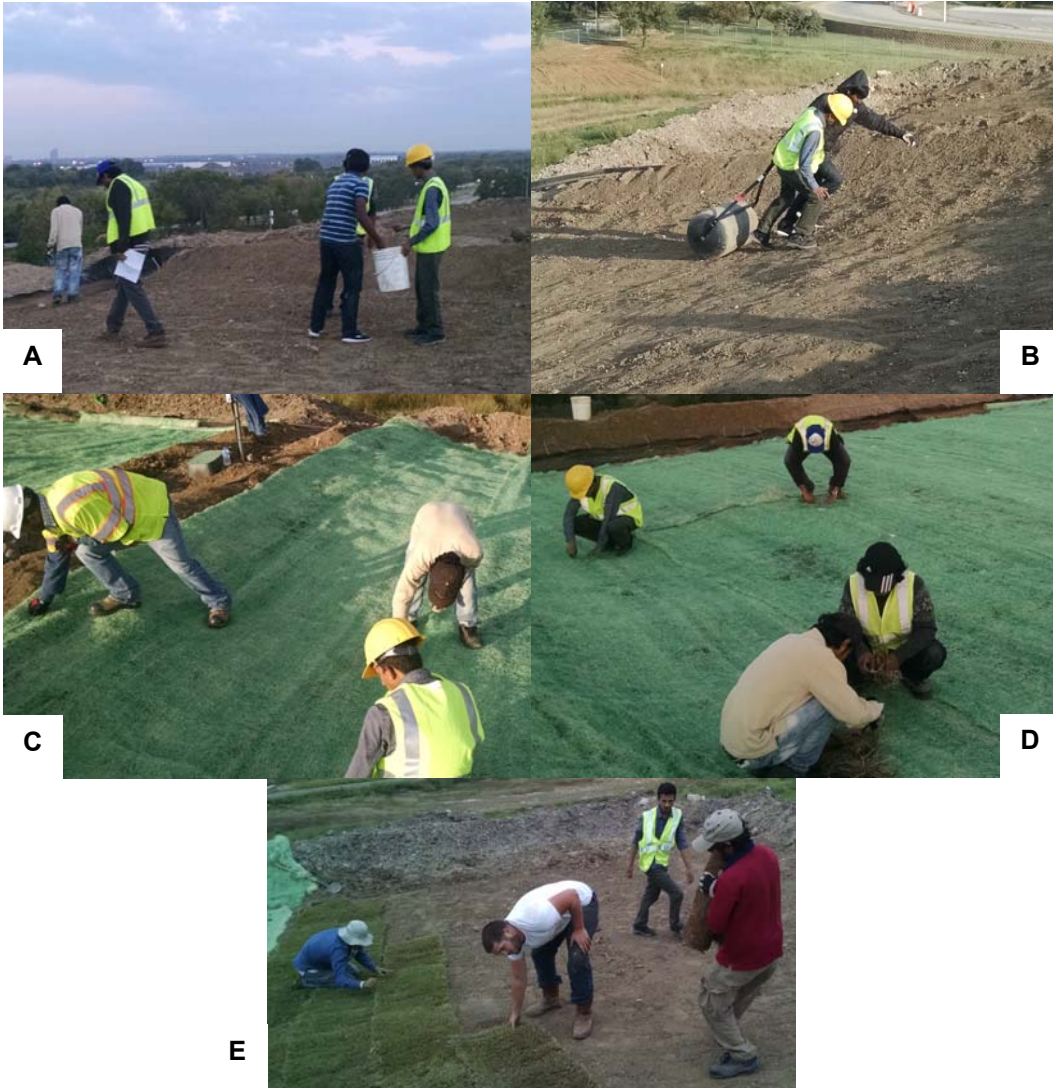
Figure 4.28: Vegetation placement procedure a) seed placement, b) rolling topsoil/seeds, c) erosion mat placement, d) switchgrass planting, and e) sod placement.
