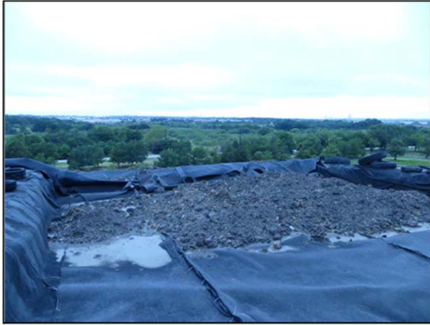
Figure A.202: Geomembrane disturbance by the wind in the middle top section.
