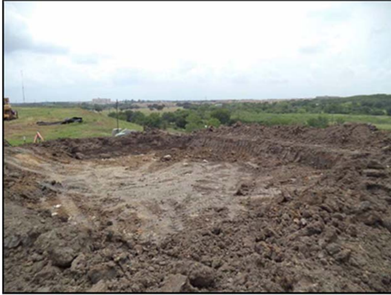
Figure A.54: Waste that was unearthed in the south top section excavation-one (1).
