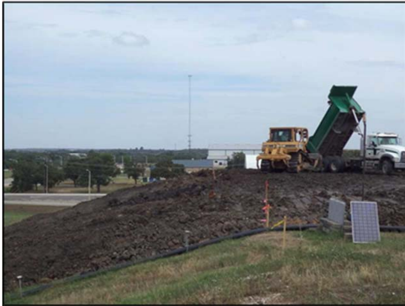
Figure A.17: Transporting soil by dump truck and moving/compacting soil by bulldozer.
