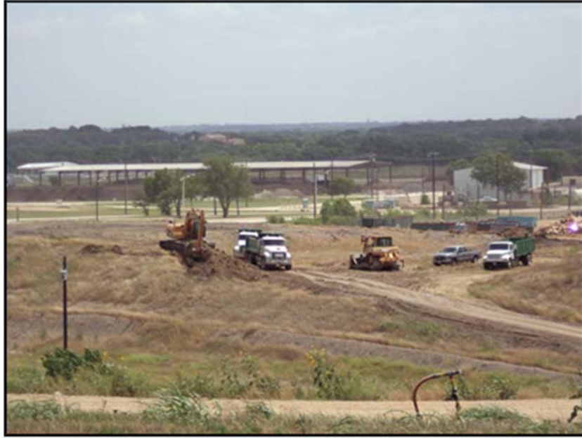
Figure A.9: Excavating the gray clay for transportation to the test section.
