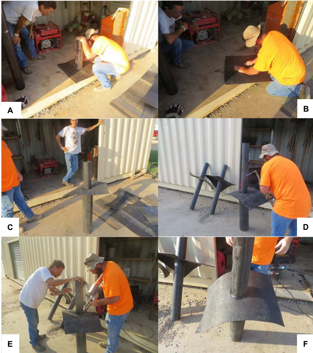
Figure 4.8: Geomembrane boot construction a) tracing the pipe to cut the hole in the geomembrane sheet, b) cutting a 4-inch hole in the geomembrane, c) placing the geomembrane sheet and 4-inch pipe in a 6-inch pipe in preparation of welding d) heating the 4-inch HDPE pipe for welding preparation, e) welding the geomembrane to the HDPE pipe, and f) results of the welding procedure.
