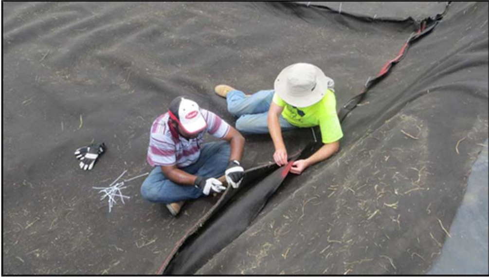
Figure A.144: Joining the geotextiles to the geocomposite drain along a sidewall by UTA.
