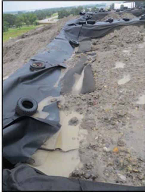
Figure A.187:: South top section details during a rainfall event.
