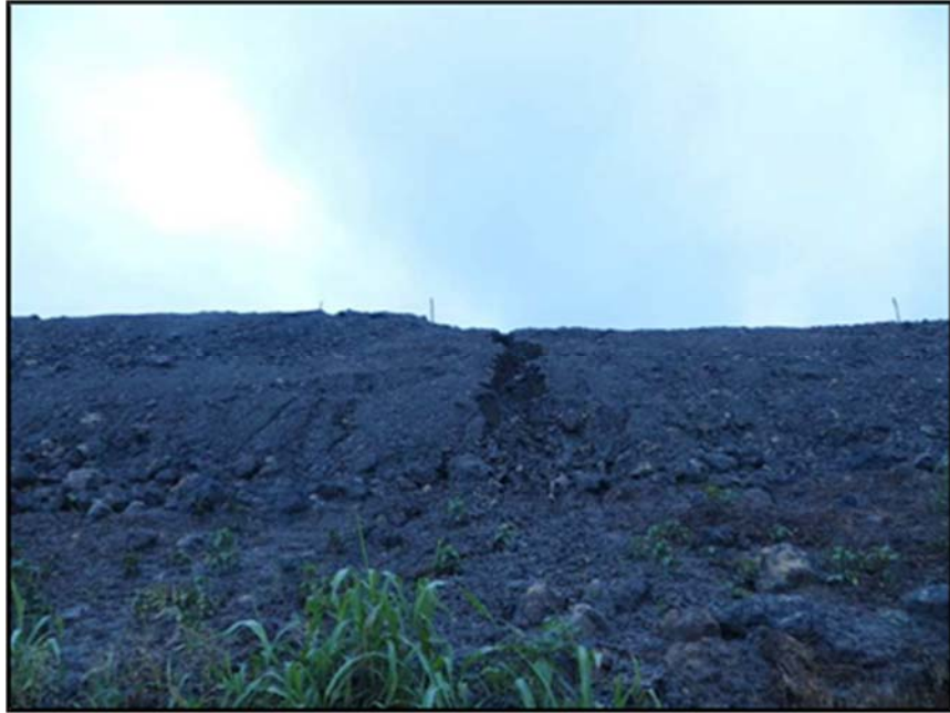
Figure A.188: Gully from the south inclined section.
