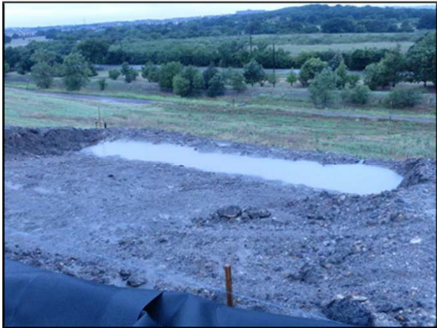
Figure A.189: Details of the south inclined section during a rainfall event.
