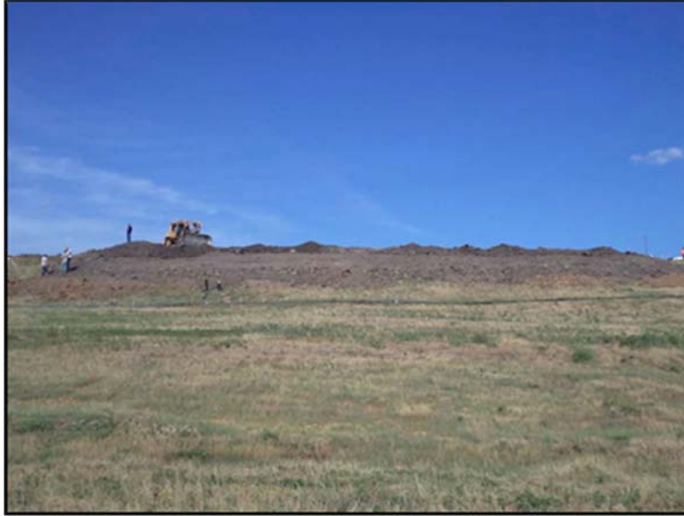
Figure A.26: View of the inclined section embankment from the bottom of the landfill slope.
