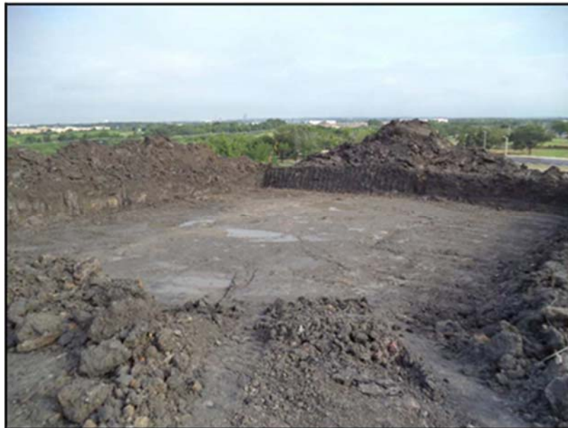
Figure A.53: Ponding as a result of a rainfall event in the morning.
