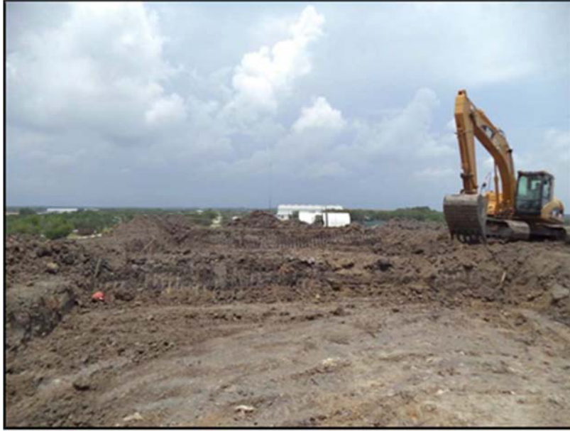
Figure A.57: Embankment addition construction and view of the top section excavations.
