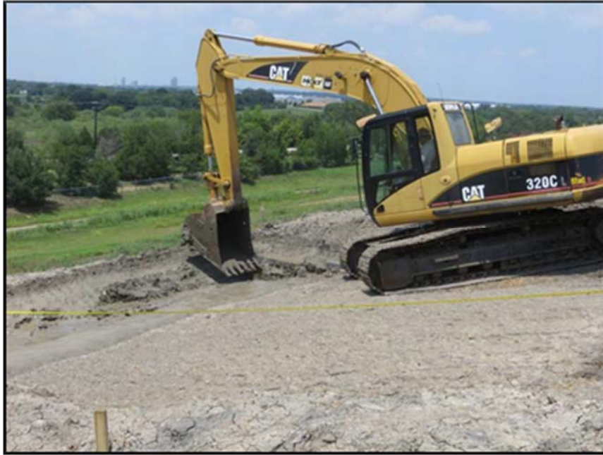
Figure A.250: Removal of soil and water from the bottom of an inclined section.
