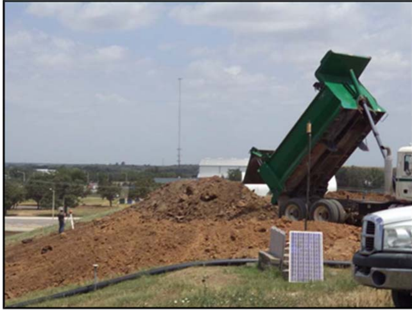
Figure A.7: Placing the gray clay on the test section prior to spreading and compaction.
