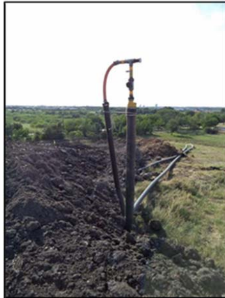
Figure A.25: Gas collection well, north of the test section.
