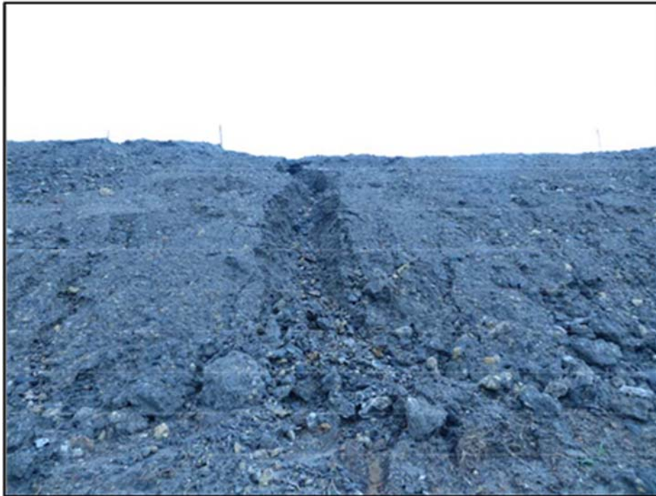
Figure A.211: Gully formed by water from the south inclined section.
