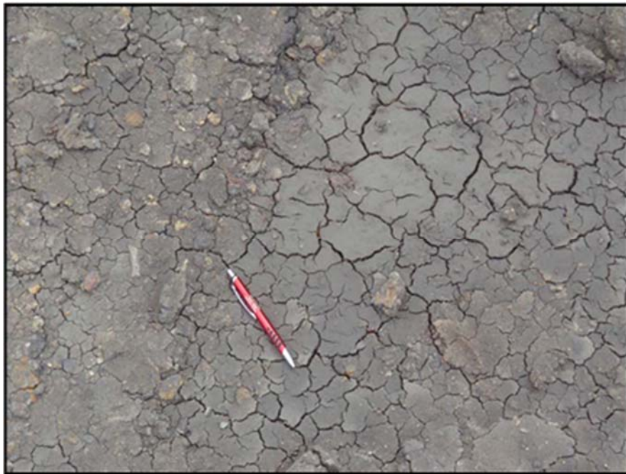
Figure A.75: Desiccation cracking of the subgrade at the beginning of the eleventh day.
