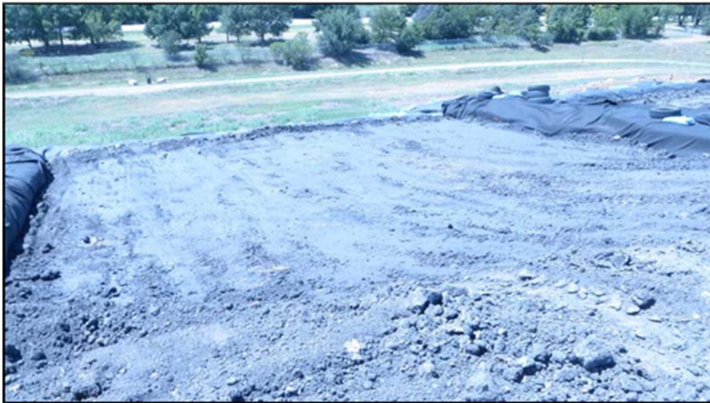
Figure A.320: End of the day details of the middle inclined section.
