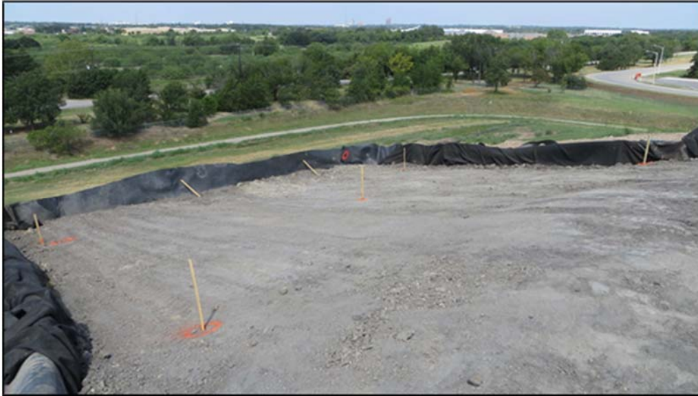
Figure A.364: End of the day details of the north inclined section.
