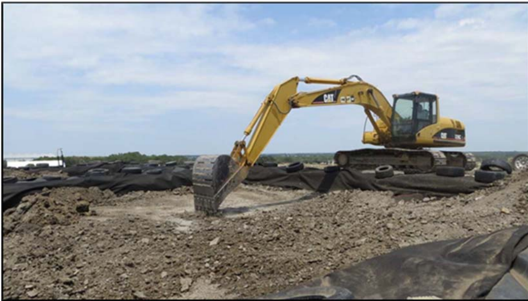
Figure A.159: Disturbing of the 1 st soil layer in the south top section lysimeter.
