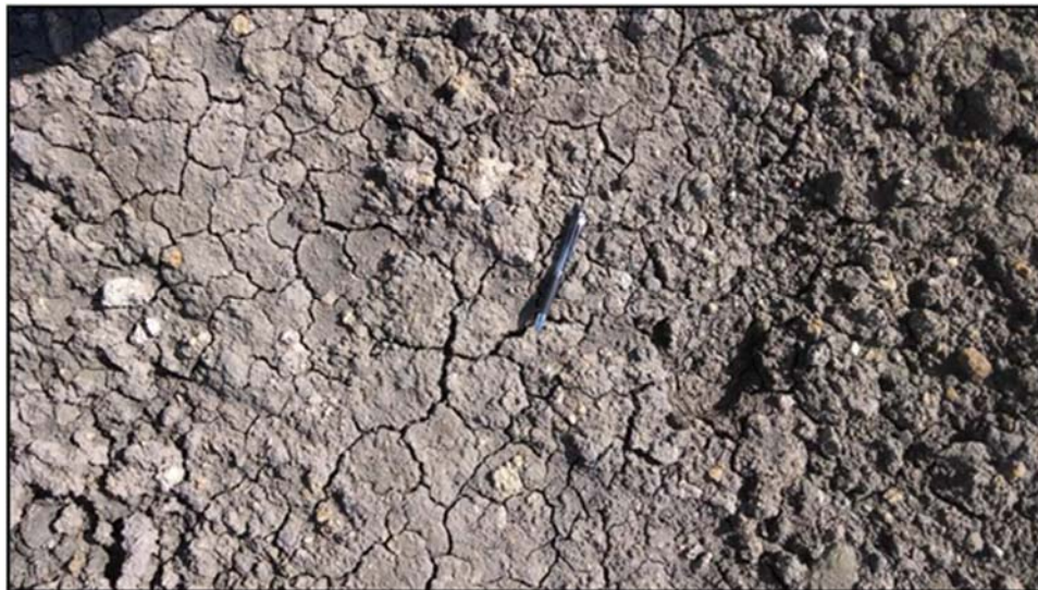
Figure A.52: Evidence of desiccation cracking on the surface of the embankment-two (2).
