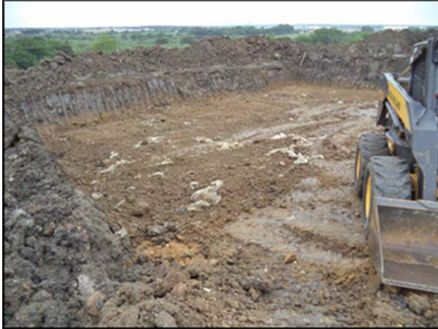
Figure A.55:Waste that was unearthed in the south top section excavation-three (3).
