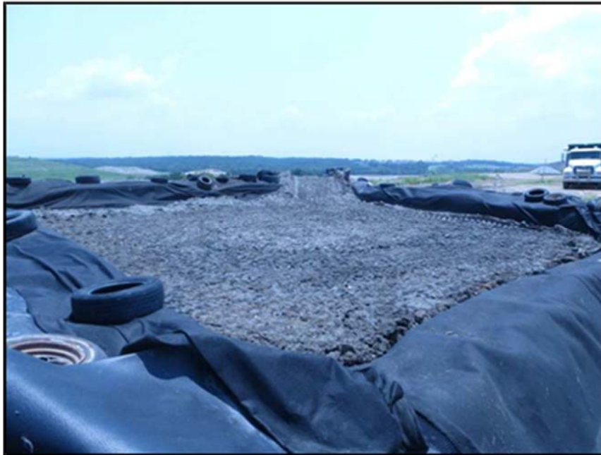
Figure A.231: First soil layer after compaction in the south top test section.
