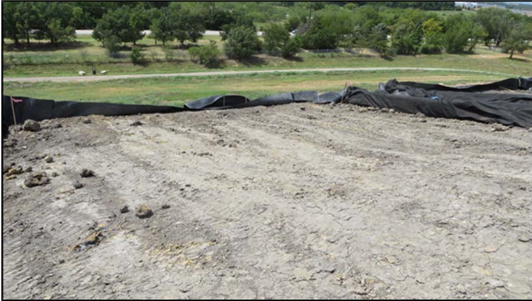
Figure A.341: End of the day details of the middle inclined section.
