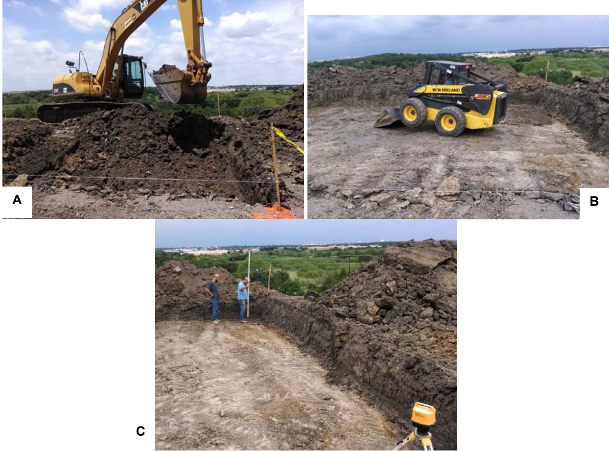
Figure 4.4: Lysimeter excavation a) excavation in preparation for a lysimeter, b) finalizing the lysimeter subgrade and compaction by a skid-steer, and c) subgrade slope and height verification.
