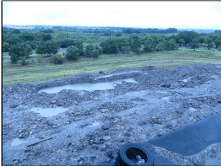
Figure A.191: Details of the north inclined section during a rainfall event.
