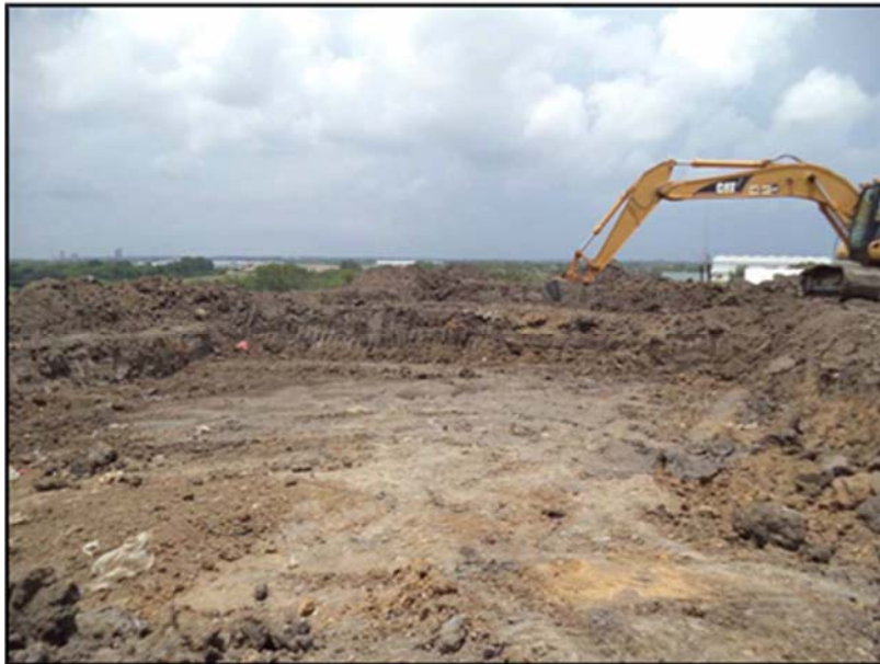
Figure 3: Waste that was unearthed in the south top section excavation-two (2).
