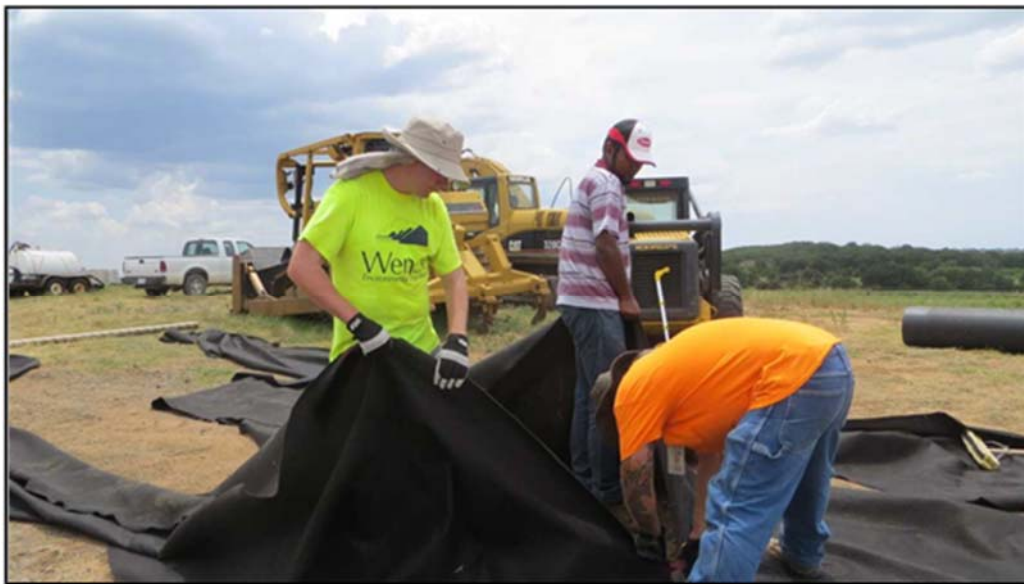
Figure A.141: Cutting the geotextile to the appropriate size for placement in the lysimeter.
