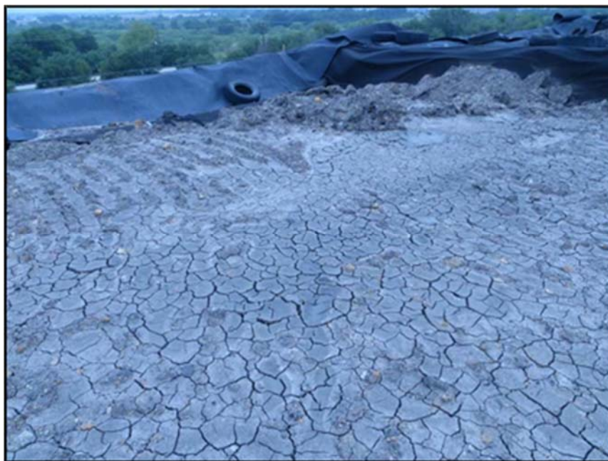
Figure A.212: Desiccation cracks present in the south top test section-one (1).
