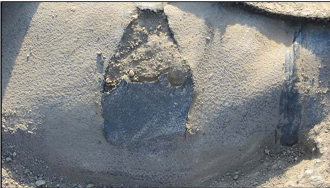
Figure A.366: Cut in the berm between the top and inclined middle sections-two (2).
