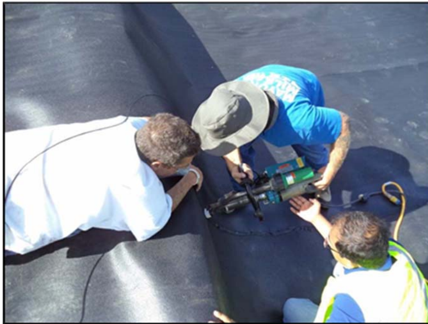
Figure A.84: Welding the geomembrane along the sidewall by the COD staff.
