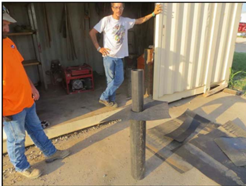
Figure A.272: Placing the geomembrane sheet and 4-inch pipe in a 6-inch pipe in preparation of welding.
