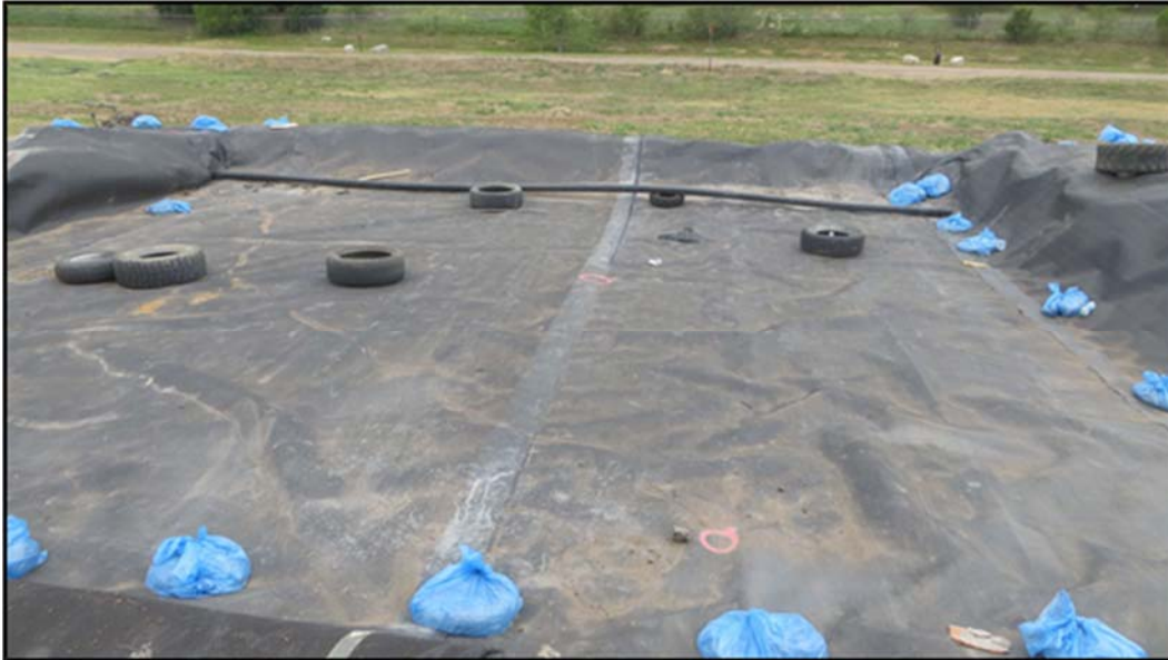
Figure A.284: South inclined section with geomembrane and HDPE piping system in place.
