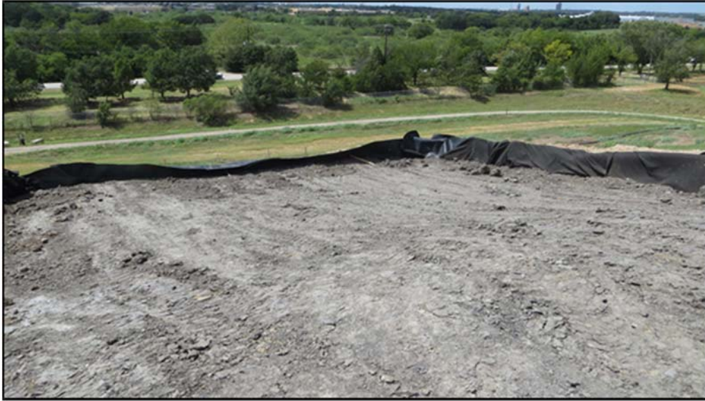
Figure A.343: End of the day details of the north inclined section.
