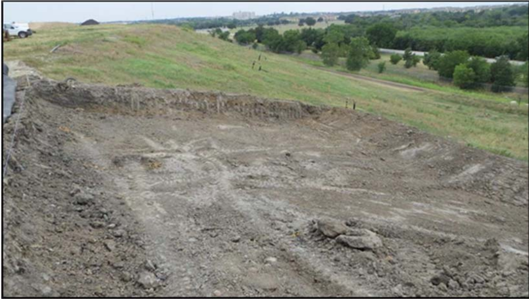
Figure A.177: End of the day details of the south inclined section-one (1).
