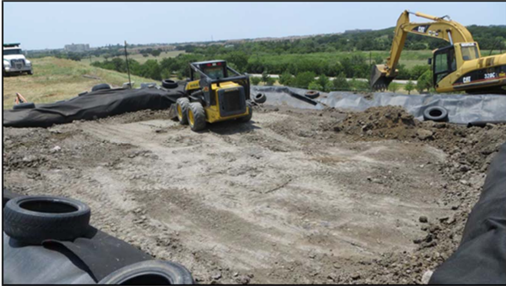
Figure A.158: 1 st soil layer preparation and compaction in the south top section lysimeter-two (2).
