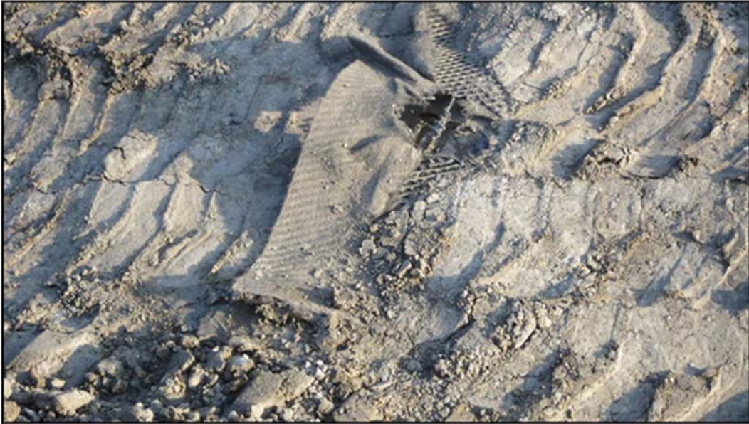
Figure A.365: Cut in the berm between the top and inclined middle sections-one (1).
