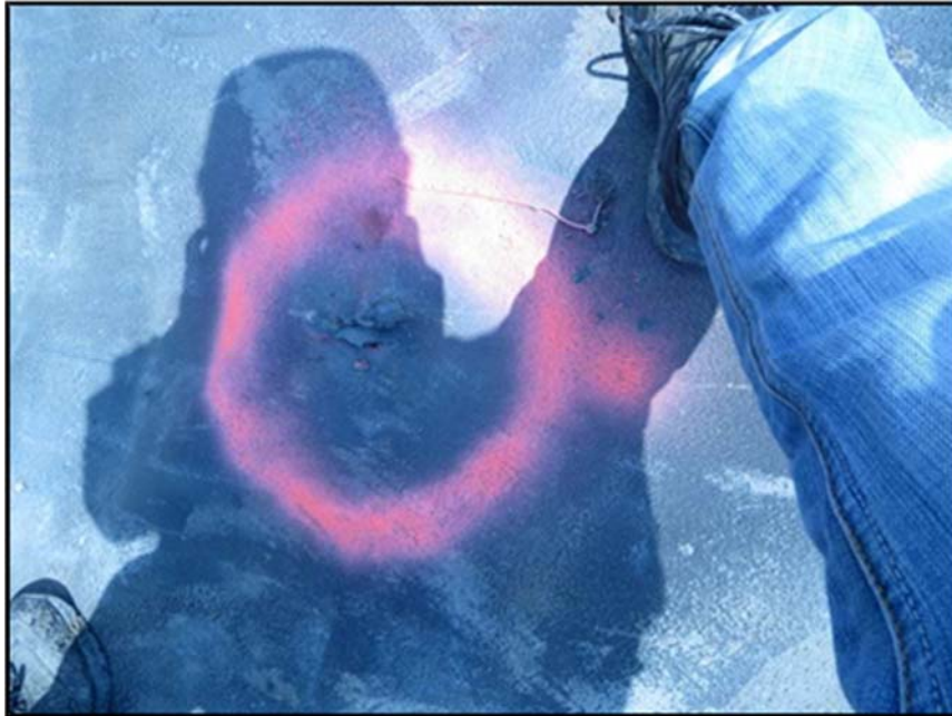
Figure A.237: Hole in the geomembrane-one (1).
