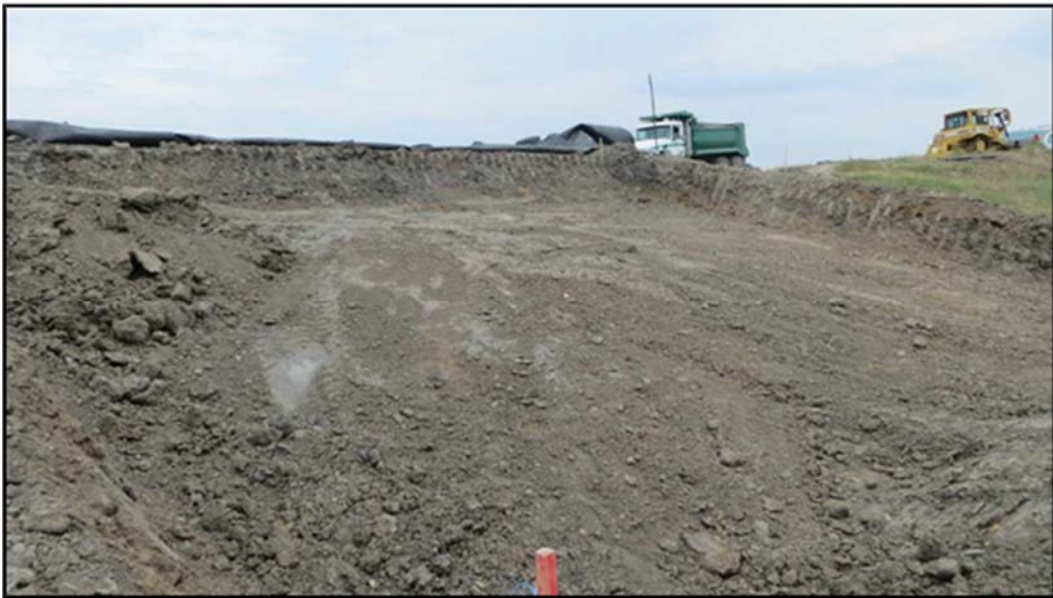
Figure A.178: End of the day details of the south inclined section-two (2).
