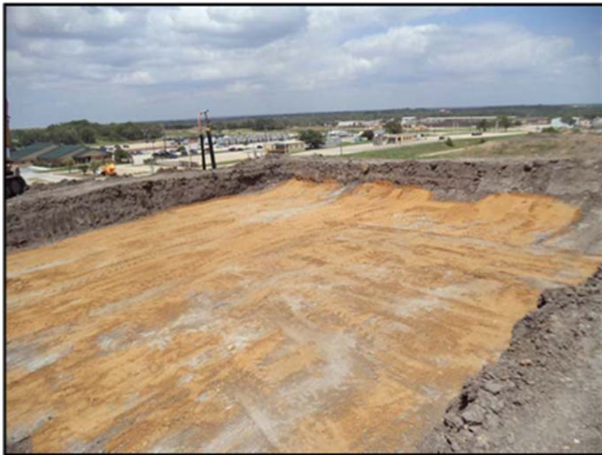
Figure A.77: Subgrade with sandy soil in low-lying areas.
