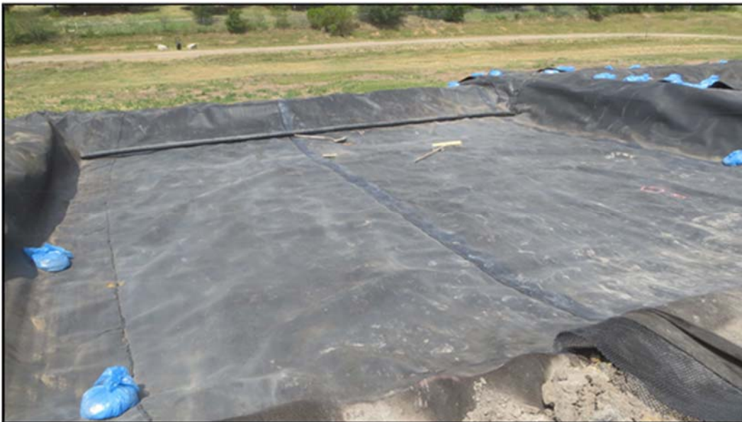
Figure A.283: Middle inclined section with geomembrane and HDPE piping system in place.
