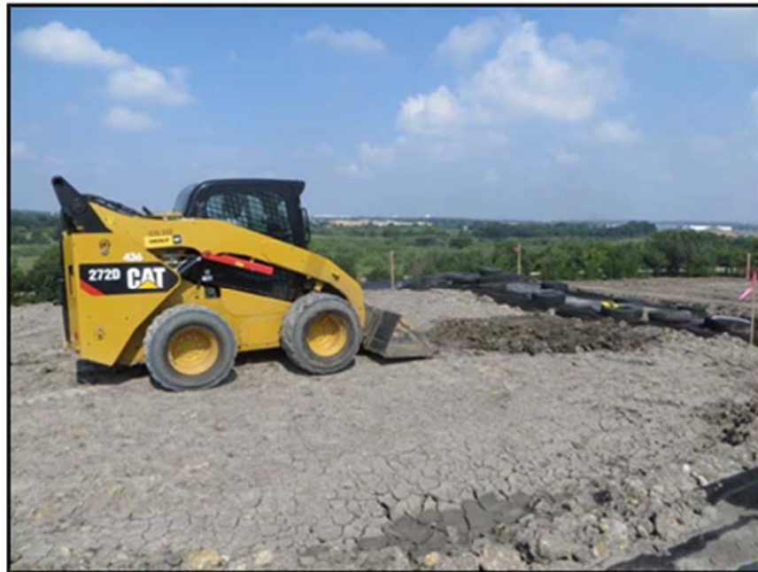
Figure A.249: Cover soil adjustment in a top section by a skid-steer.
