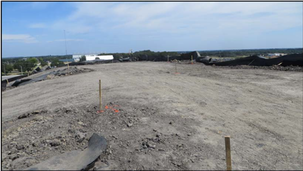
Figure A.361: End of the day details of the middle top section.
