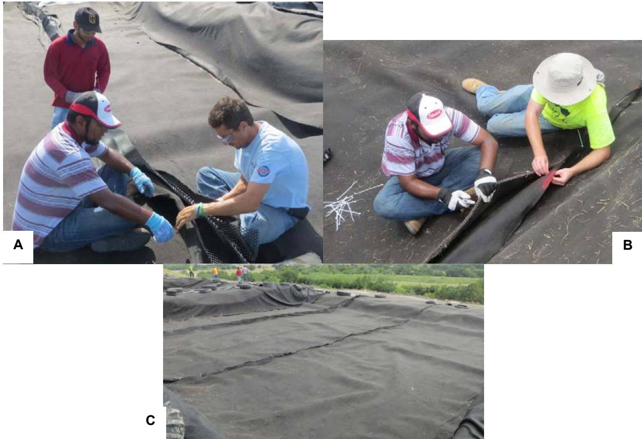
Figure 4.12: Geocomposite drain placement a) joining adjacent geocomposite drains, b) joining geocomposite drain and geotextile (located on the sidewall), and c) finished with geocomposite in a lysimeter.
