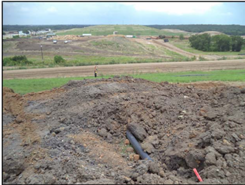
Figure A.58: View of the leachate injection pipe.
