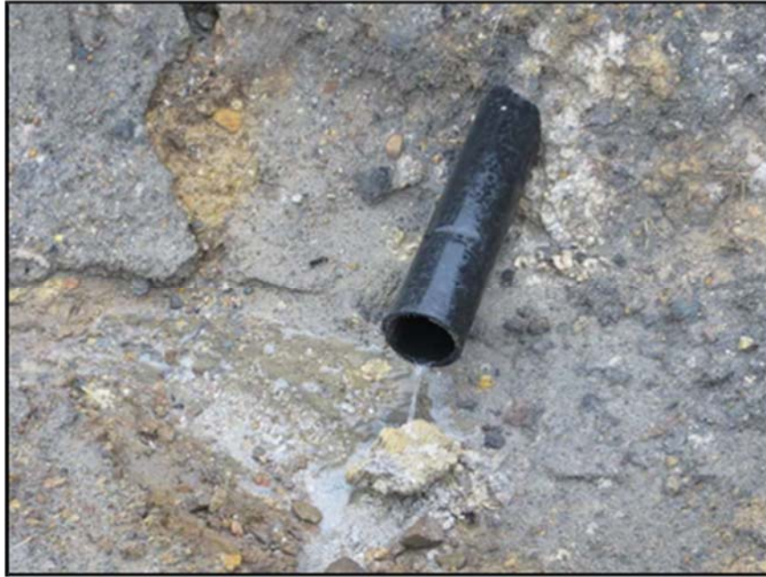
Figure A.180:: Flow of water from the south top section.
