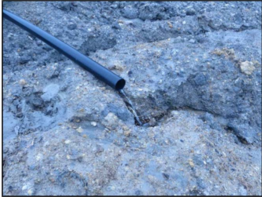
Figure A.182: Flow of water from the north top section.
