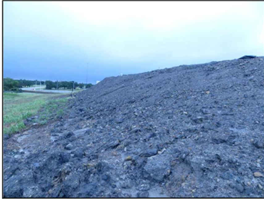
Figure A.208: North inclined section details after a rainfall event.
