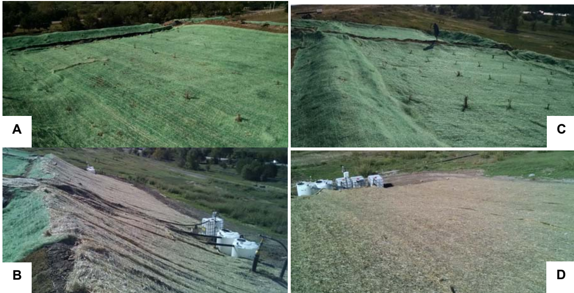
Figure 4.30: Finalized construction of a) a top section, b) an inclined section, c) west embankment and collection tanks, and d) north embankment and collection tanks.
