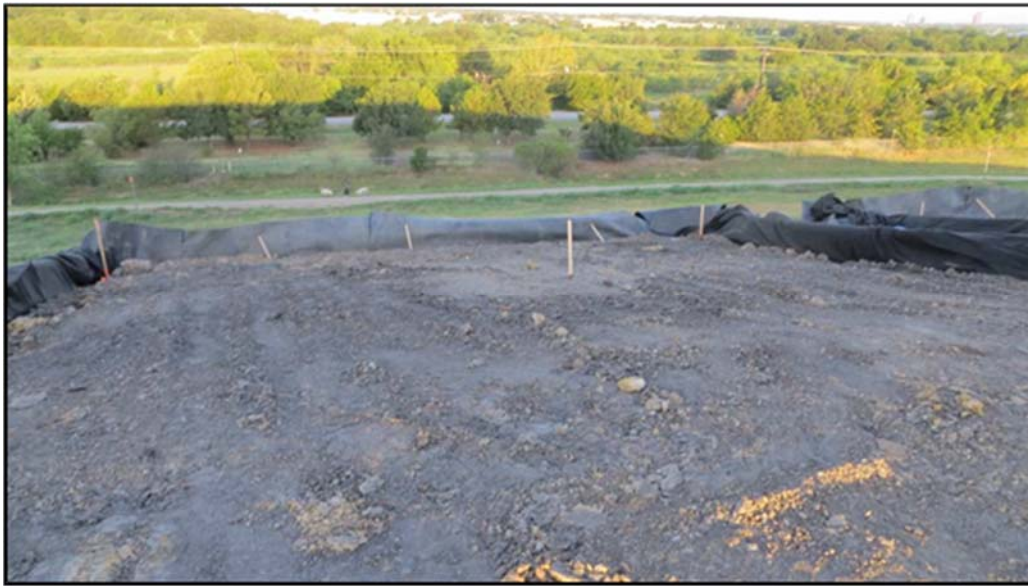
Figure A.347: Beginning of the day details of the middle inclined section.
