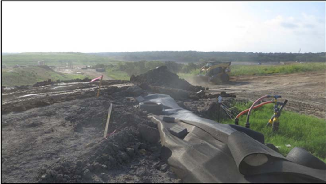
Figure A.304: Entrance ramp constructed in the southeast corner of the south top section.
