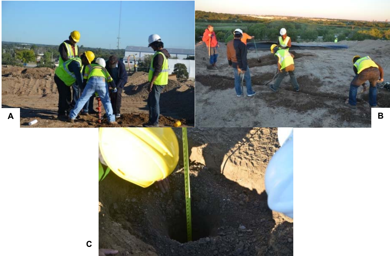
Figure 4.34: Moisture and tensiometers installation a) excavation by hand-held auger, b) digging of trenches for sensor wiring, and c) ensuring correct depth prior to sensor placement.
