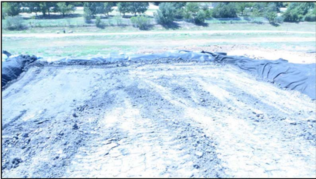
Figure A.319: End of the day details of the north inclined section.
