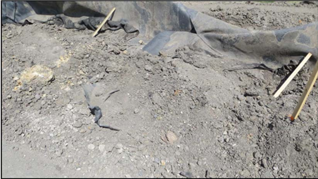
Figure A.351: Cut in the liner between the north and middle inclined sections.
