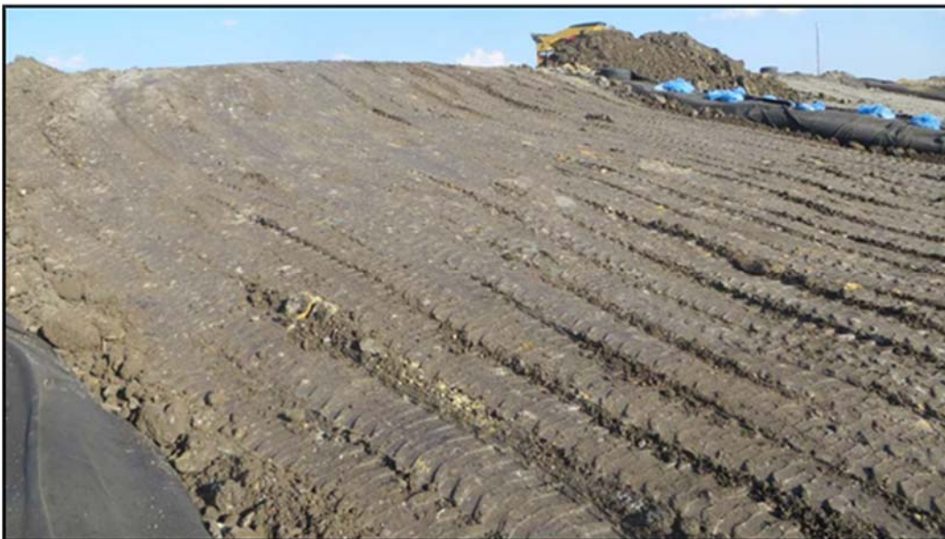
Figure A.326: End of the day details of the middle inclined section.
