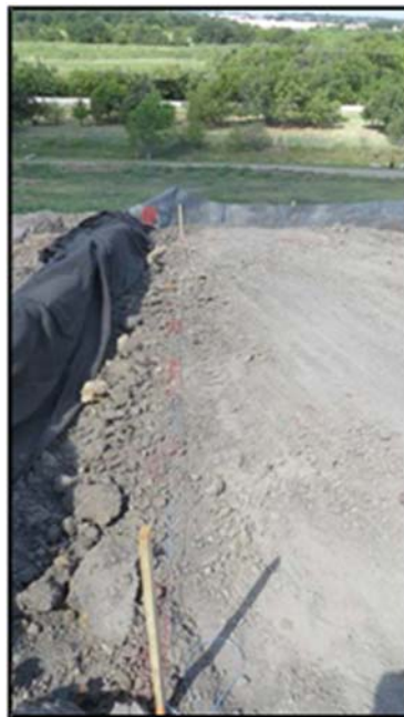
Figure A.352: String line placed to achieve the 3-foot of compacted clay requirement.
