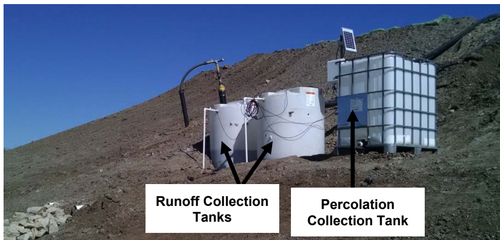
Figure 4.35: In-place runoff and percolation collection tanks.
