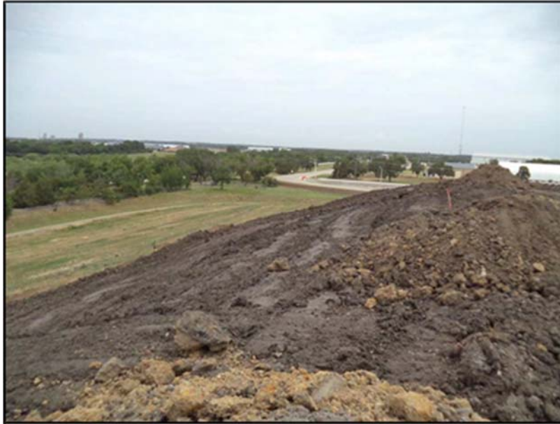
Figure A.36: View of the inclined section from the south on the sixth day (near completion).
