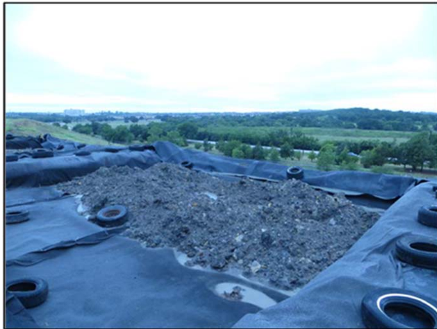
Figure A.197: Geocomposite drain details in a lysimeter (mud, not water present near the soil pile on the geocomposite drain).
