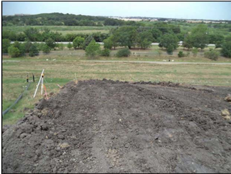
Figure A.35: View of the inclined section (south side) from the top section on the sixth day.
