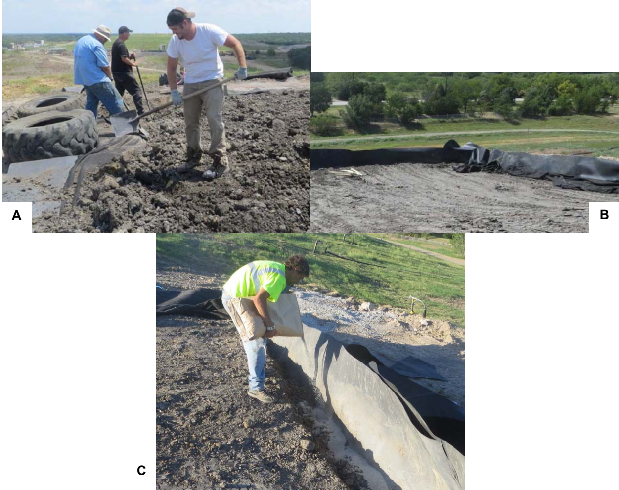
Figure 4.18: Top of sidewall preparation a) removal of excess soil around the lysimeter perimeters, b) results of placing geomembrane vertical, and c) placing bentonite along the lysimeter perimeters.
