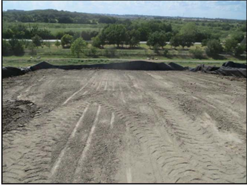
Figure A.353: End of the day details of the south inclined section.
