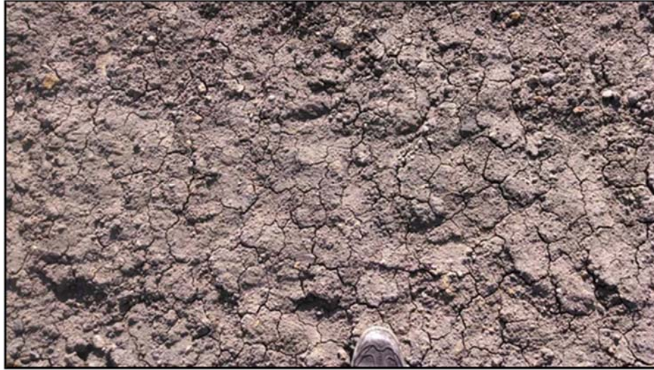
Figure A.51: Evidence of desiccation cracking on the surface of the embankment-one (1).
