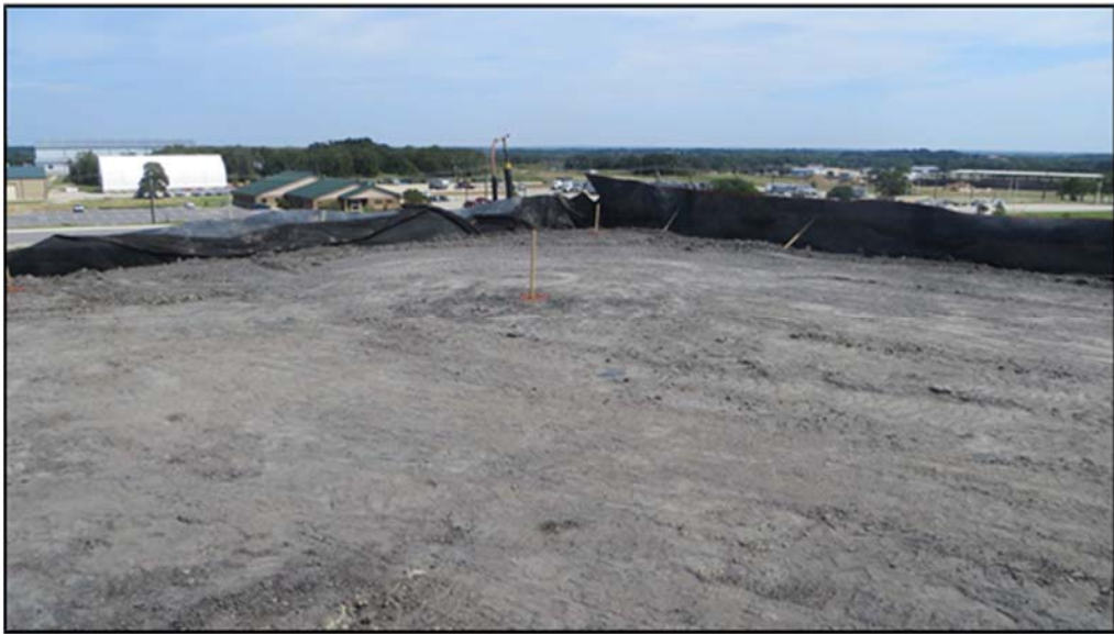
Figure A.363: End of the day details of the north top section.
