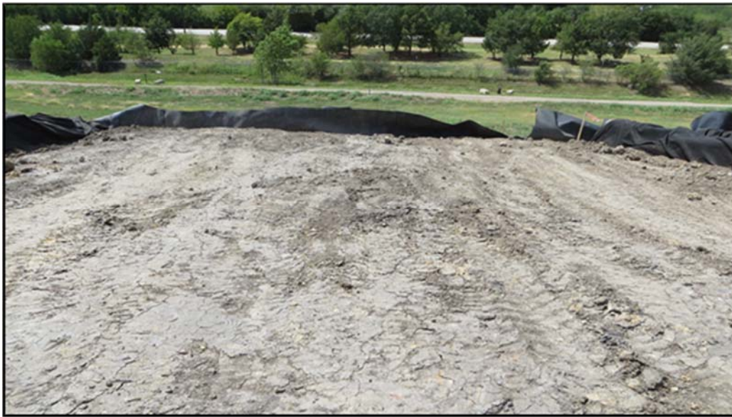
Figure A.340: End of the day details of the south inclined section.
