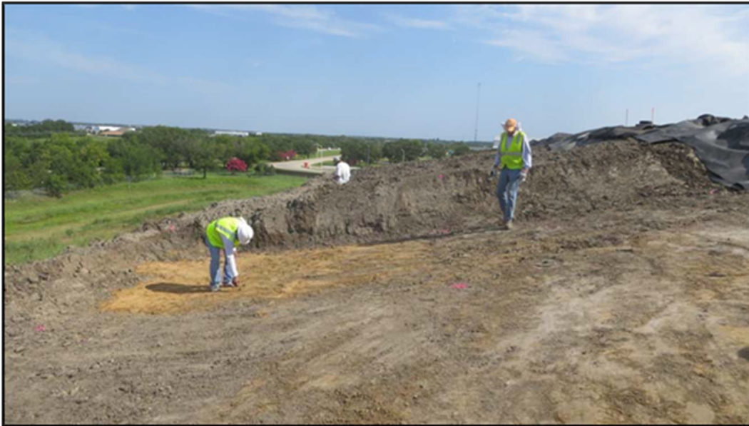
Figure A.266: Removing rocks and soil clods from the subgrade prior to geomembrane placement.
