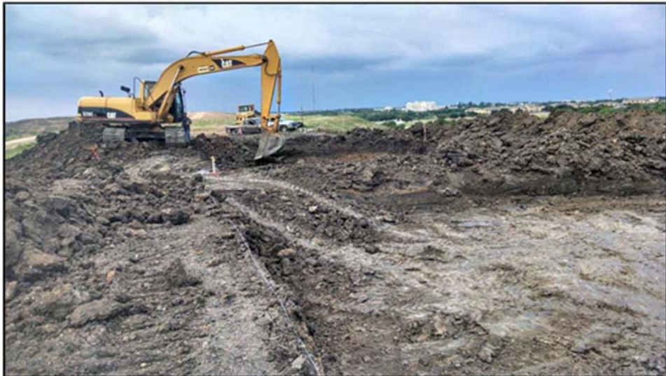
Figure A.48: Two (2) of the top test sections nearing completion of the excavation.
