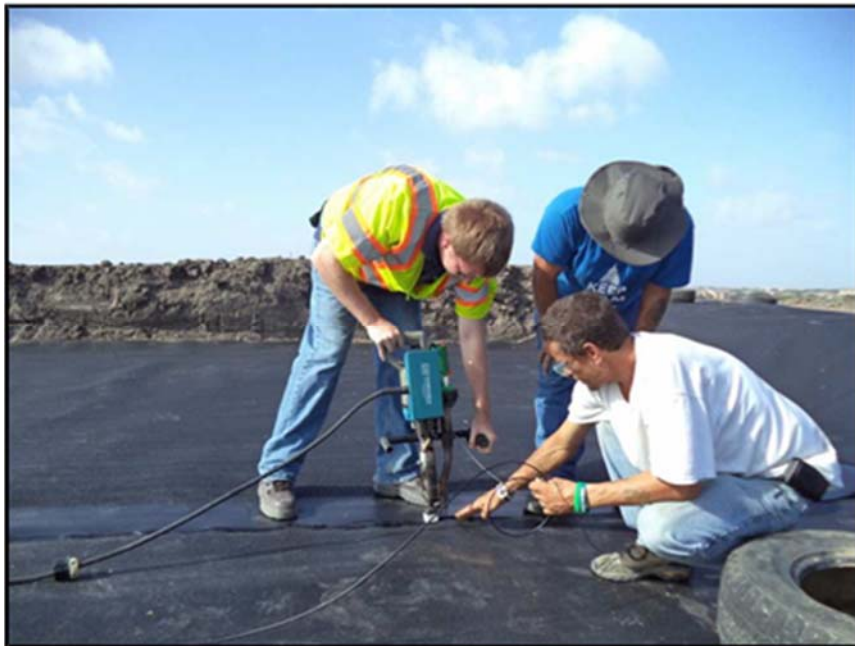
Figure A.81: Welding of the geomembrane by the University of Texas at Arlington (UTA)-
