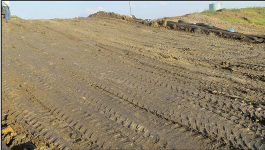
Figure A.327: End of the day details of the south inclined section.
