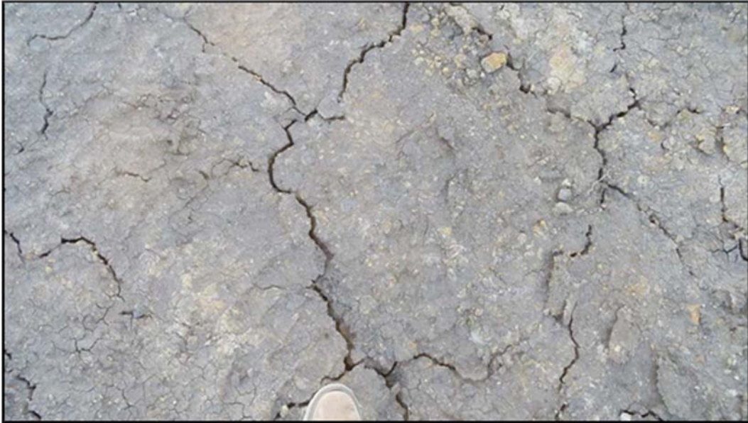
Figure A.349: Desiccation cracks present in an inclined section.
