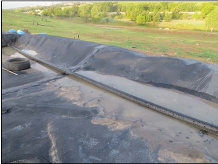
Figure A.290: After rainfall event details of the south inclined section.
