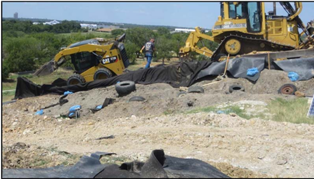
Figure A.375: Skid-steer stuck in the south inclined section.
