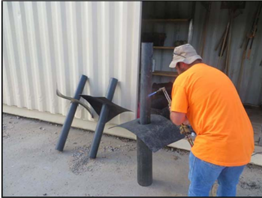
Figure A.273: Heating the 4-inch HDPE pipe in preparation of welding it to the geomembrane sheet.
