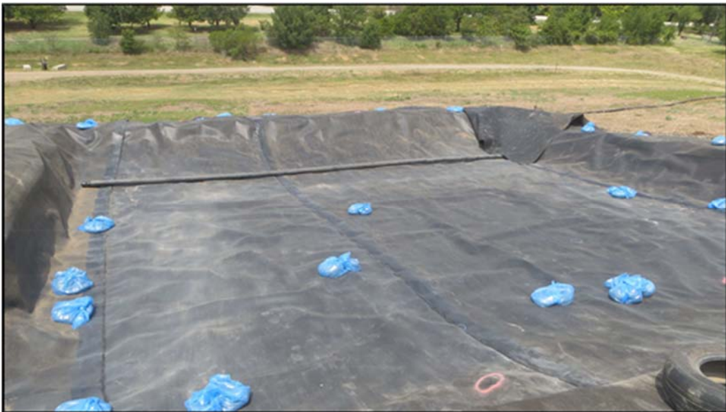
Figure A.282: North inclined section with geomembrane and HDPE piping system in place.
