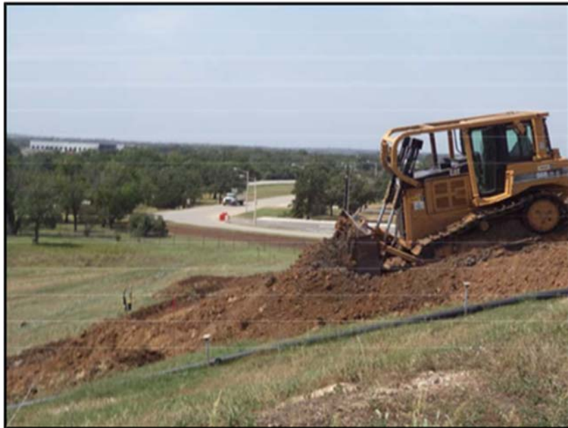
Figure A.8: Spreading and compacting the gray clay in the inclined section.
