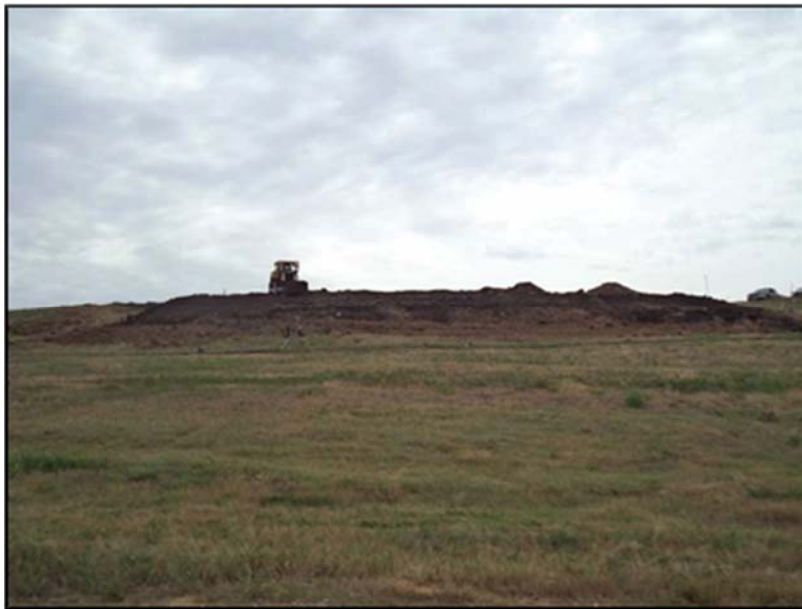
Figure A.37: View of the inclined section from the toe of the landfill slope on the sixth day (near completion).
