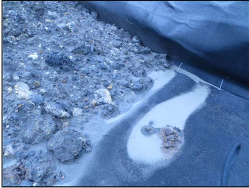
Figure A.198: Geocomposite drain and mud (not mud ridden water) details in a lysimeter.
