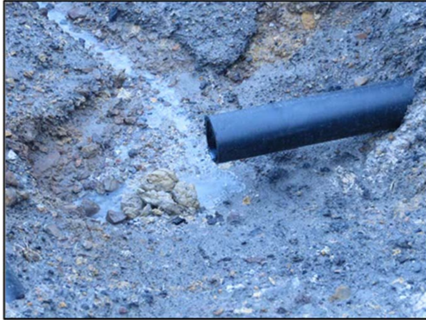
Figure A.196: Pipe details from the south top section lysimeter (trickling flow seen).
