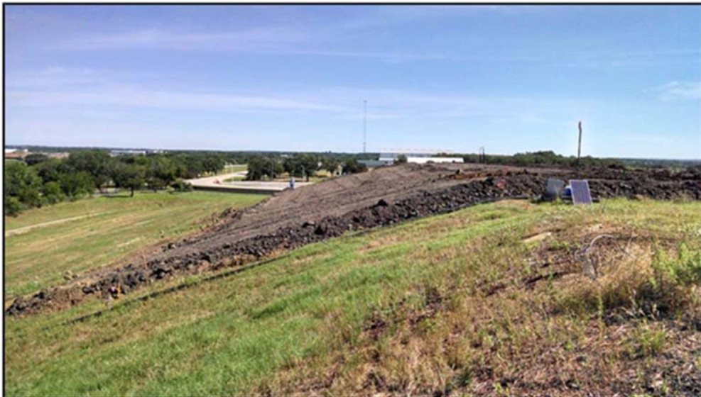
Figure A.38: Photograph of the embankment at the beginning of the eight day- one (1).
