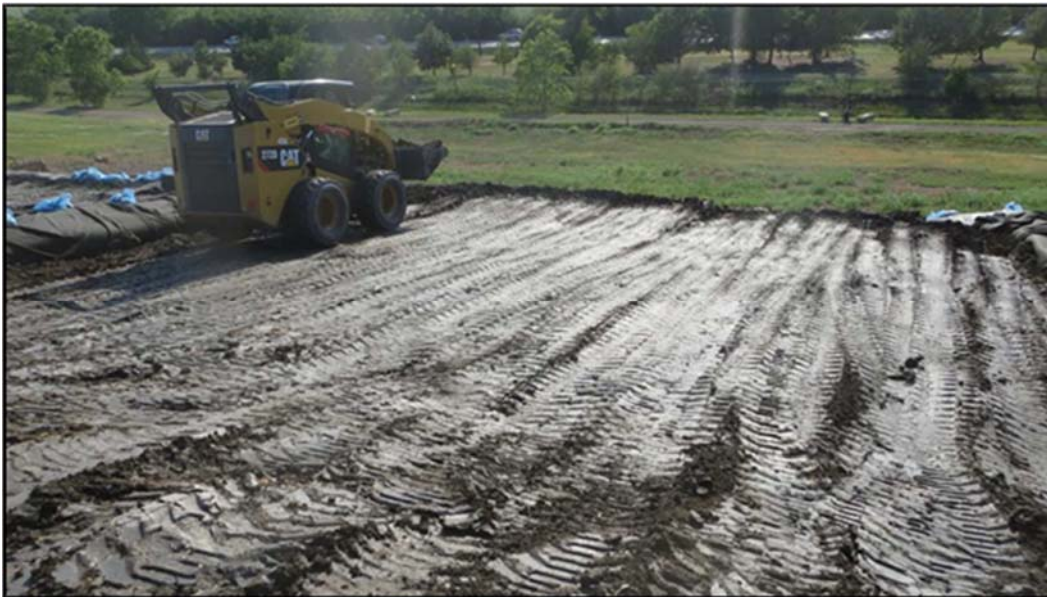
Figure A.325: End of the day details of the north inclined section.
