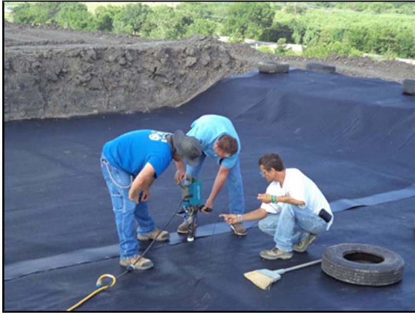
Figure A.80: Welding of the geomembrane by the City of Denton (COD) staff.
