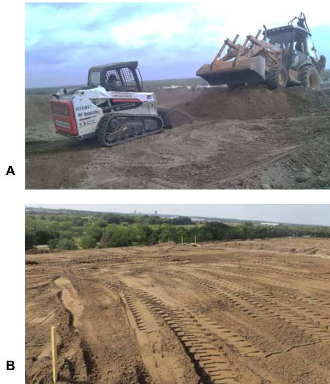
Figure 4.24: Topsoil placement a) placing the topsoil above compacted clay and b) 1-foot of topsoil placed.
