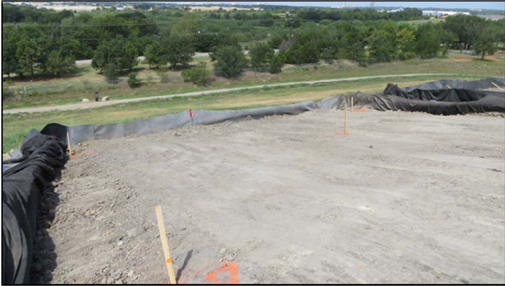
Figure A.362: End of the day details of the middle inclined section.
