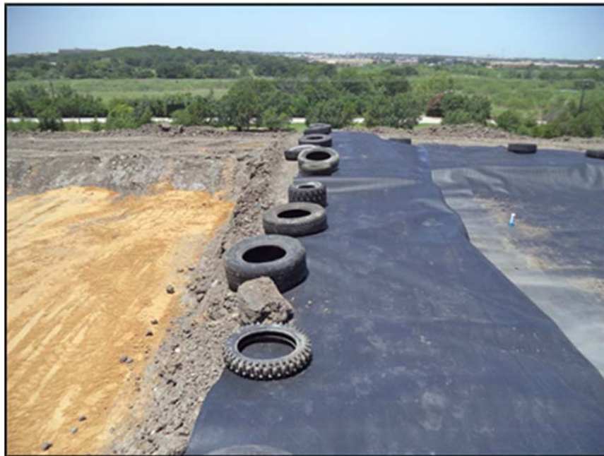
Figure A.87: Tires placed on the geomembrane on the top of the embankment.
