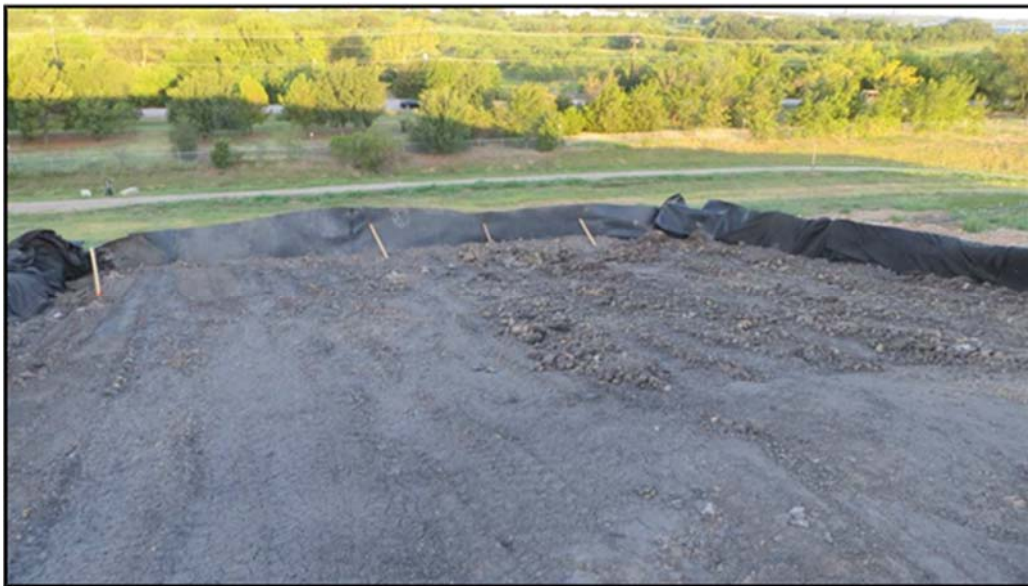
Figure A.348: Beginning of the day details of the north inclined section.
