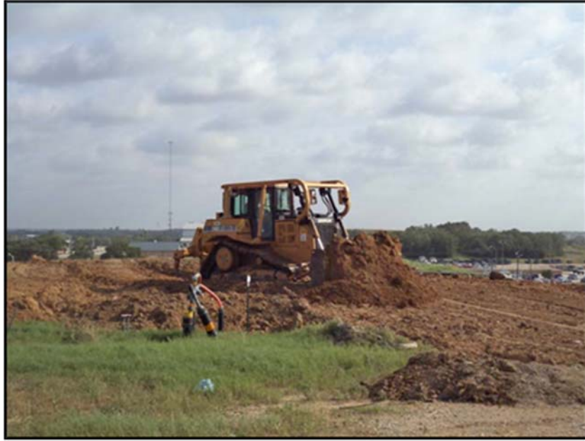
Figure A.5: Placement and compaction of the embankment base in the top section.
