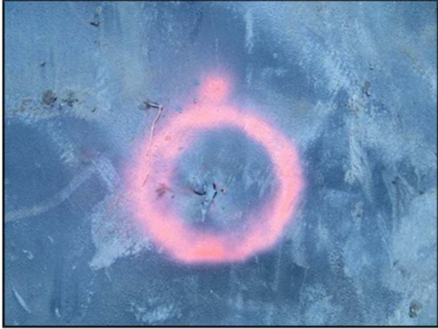
Figure A.238: Hole in the geomembrane-two (2).
