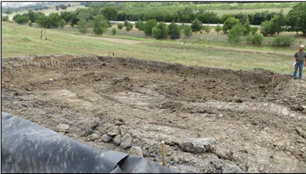
Figure A.163: South inclined section lysimeter excavation at the end of the day.
