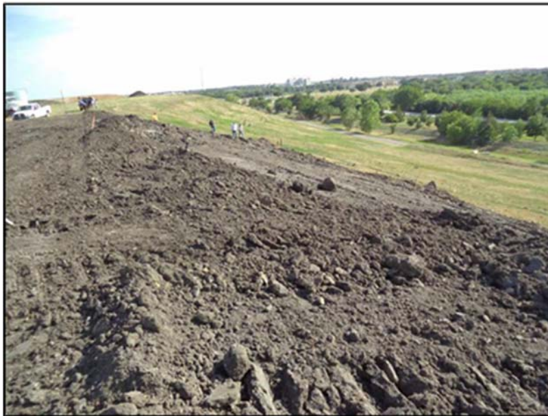
Figure A.27: View of the inclined section embankment from the top section.
