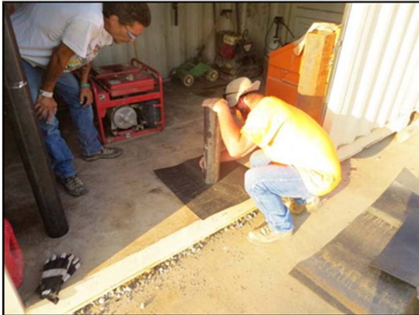
Figure A.270: Tracing the pipe to effectively cut the hole in a geomembrane sheet.
