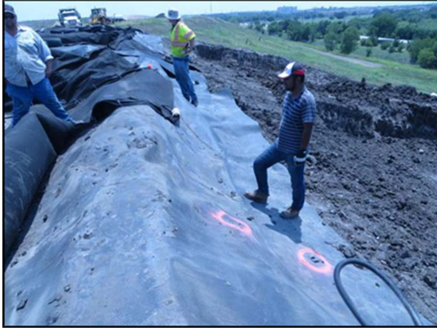
Figure A.236: Locations of the holes in the geomembrane (circled by the paint).
