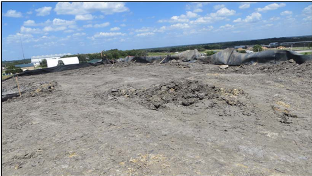
Figure A.342: End of the day details of the middle and north top sections.
