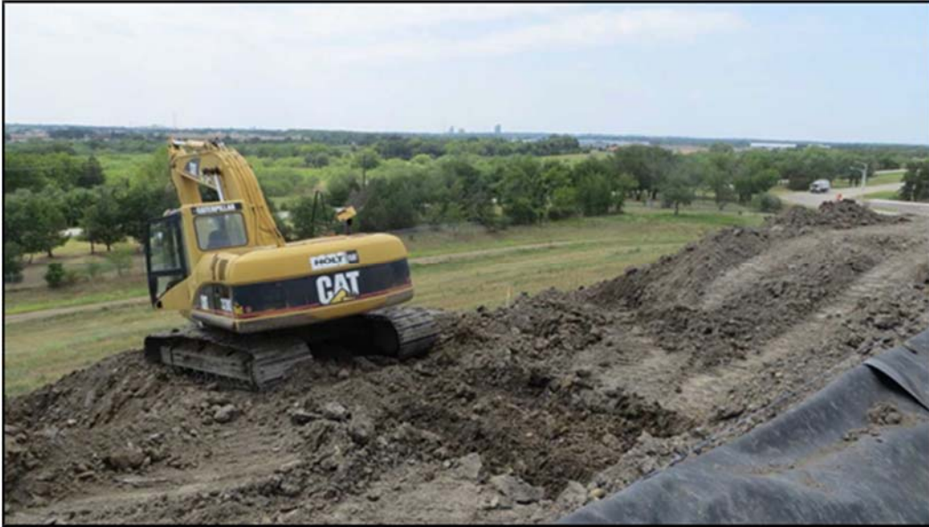
Figure A.164: Middle inclined section lysimeter excavation at the end of the day.
