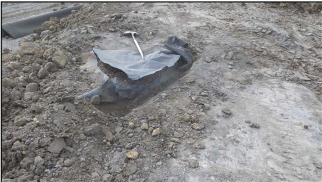
Figure A.305: Liner cut details in the southeast corner of the south top section.
