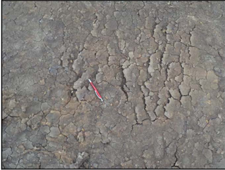
Figure A.76: Subgrade cracking at the beginning of the eleventh day.
