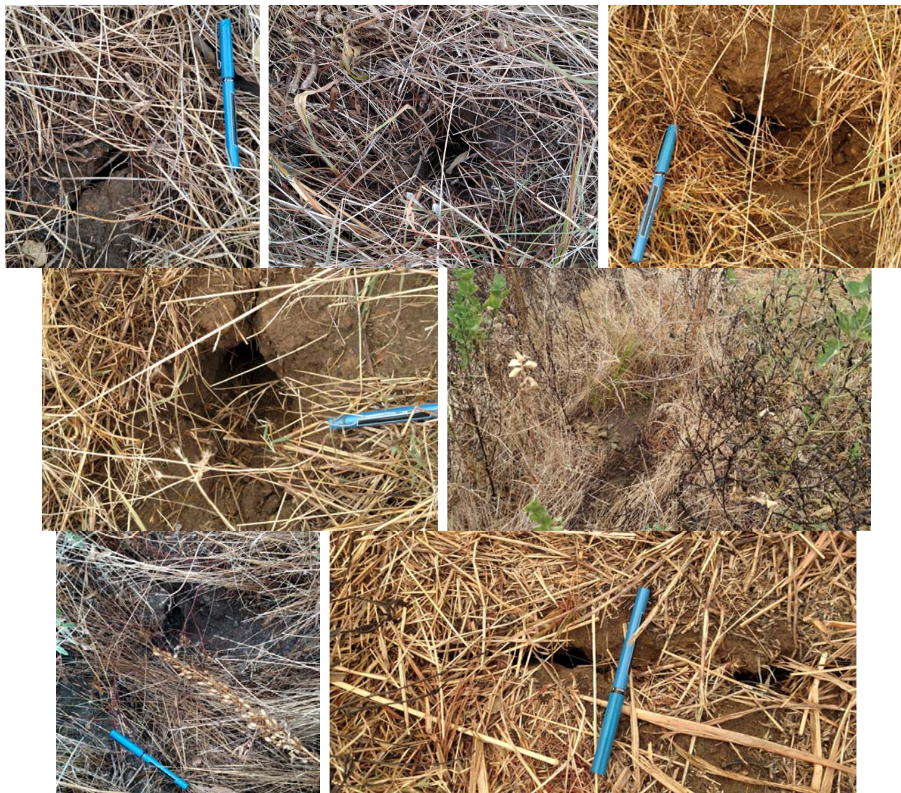
Figure 5.38: Rodent burrows and cracking – August 2016
