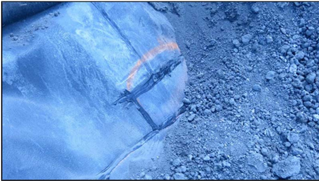
Figure A.316: Results of re-welding the separation in the liner.
