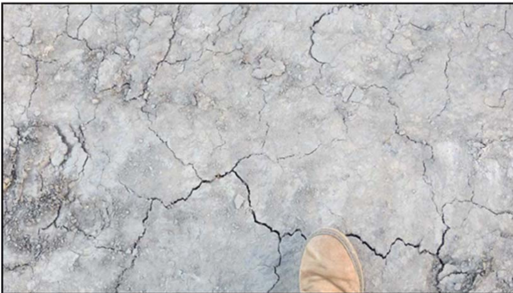
Figure A.315: Desiccation cracks found in the top of the soil layer.
