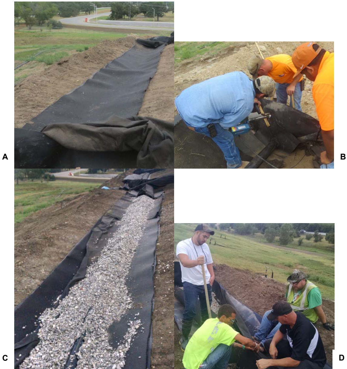
Figure 4.22: Runoff collection system a) geomembrane and geocomposite drain placement, b) welding geomembrane boot, c) runoff collection pipe and pea-gravel placement, and d) placing zip-ties to join the geocomposite drain.
