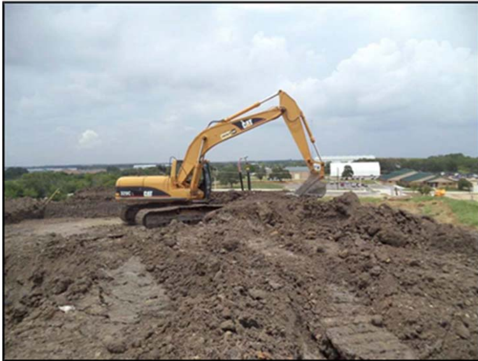
Figure A.56: Construction of an additional 1-foot of embankment around the excavation areas.
