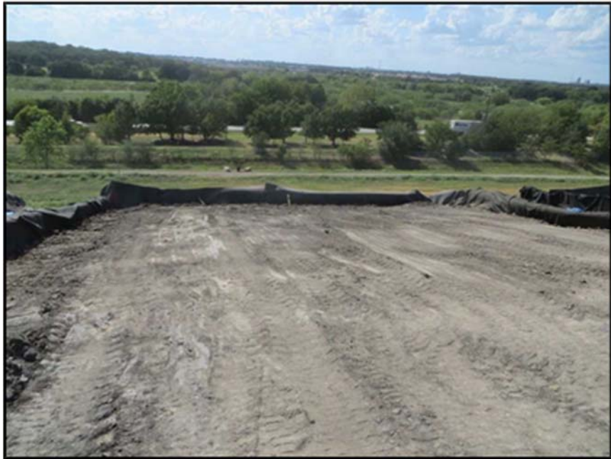
Figure A.354: End of the day details of the middle inclined section.
