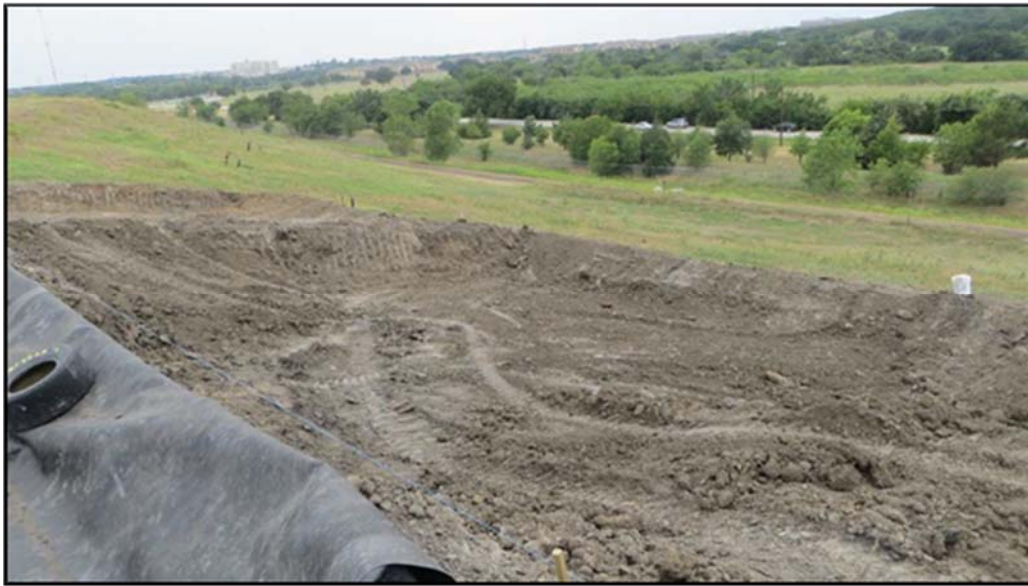
Figure A.175: End of the day details of the middle inclined section-one (1).
