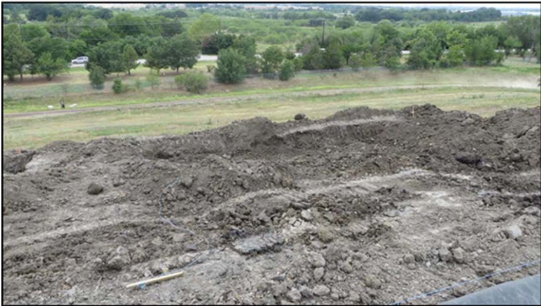
Figure A.174: End of the day details of the north inclined section.
