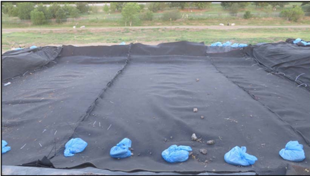
Figure A.301: All of the geosynthetics placed in the south inclined section.
