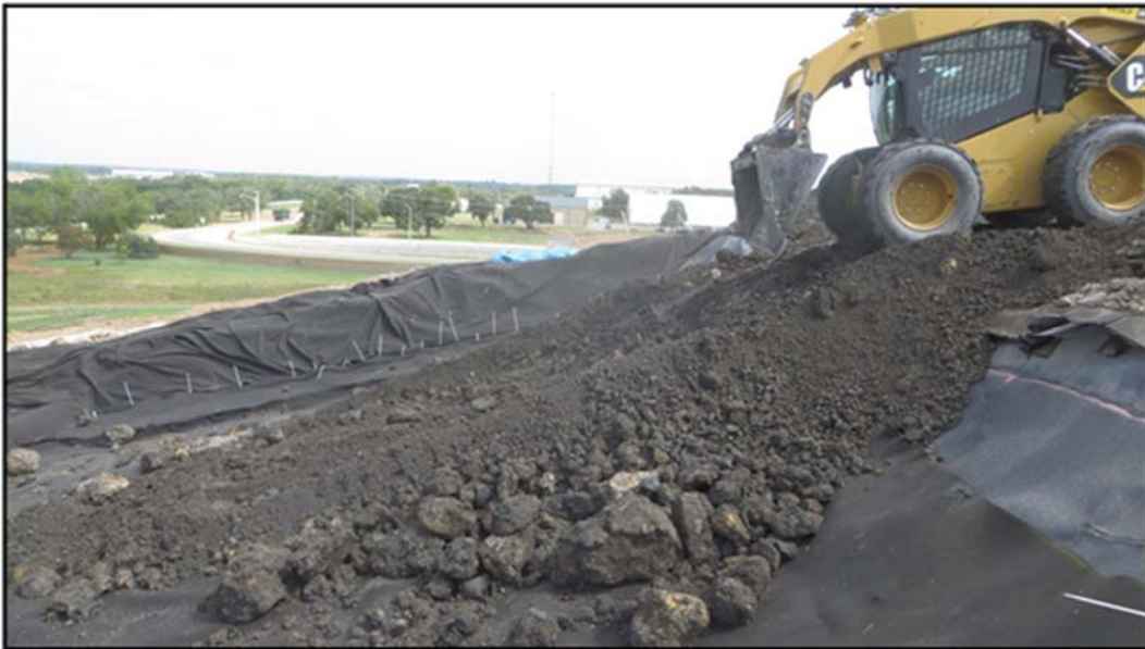
Figure A.307: Entrance ramp construction for soil placement in an inclined section.
