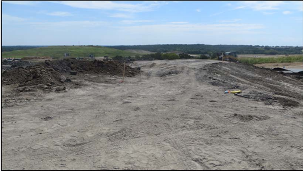
Figure A.360: End of the day details of the south top section.
