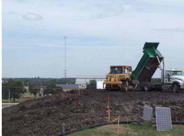
Figure 4.2: Embankment construction a) construction by bulldozer, b) water application for compaction purposes, and c) transportation of soil to the site.
