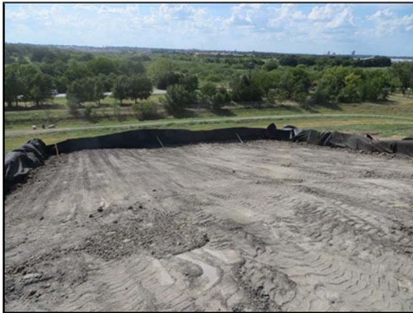
Figure A.355: End of the day details of the north inclined section.
