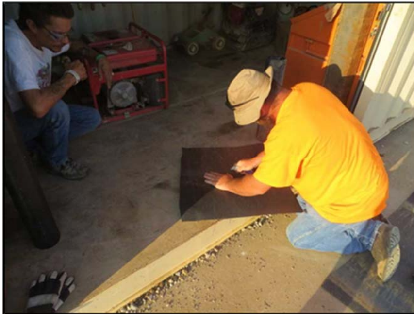
Figure A.271: Cutting the hole in the sheet for the 4-inch HDPE pipe.
