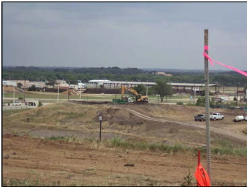
Figure A.13: Excavation from the borrow pit to utilize as the embankment.
