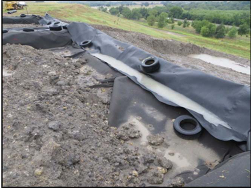
Figure A.186: Middle top section details during a rainfall event.
