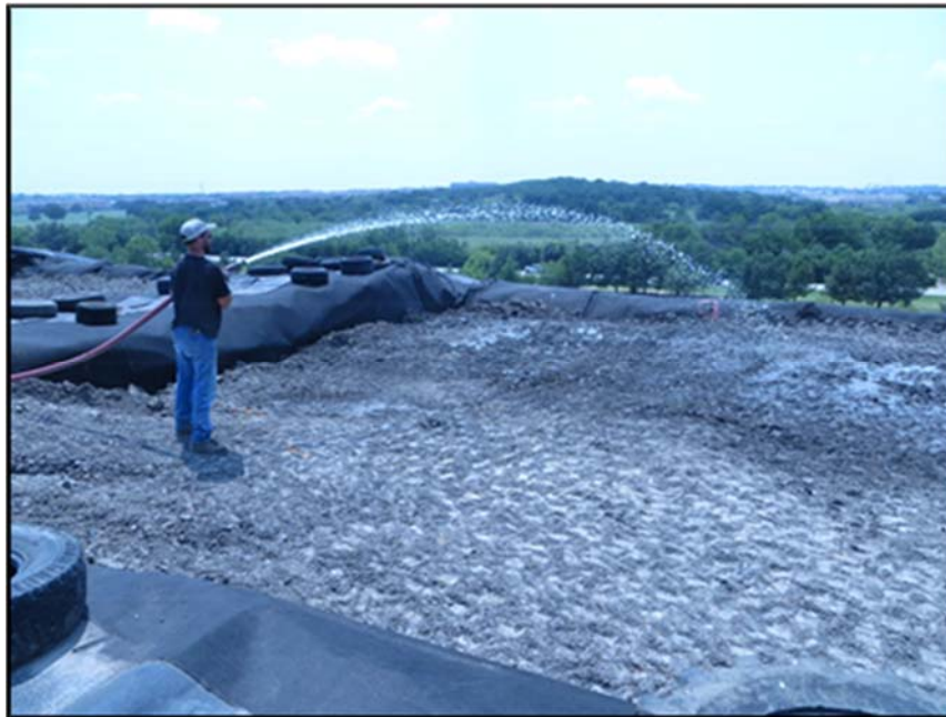
Figure A.245: Water application to the 1 st soil layer in a top section.
