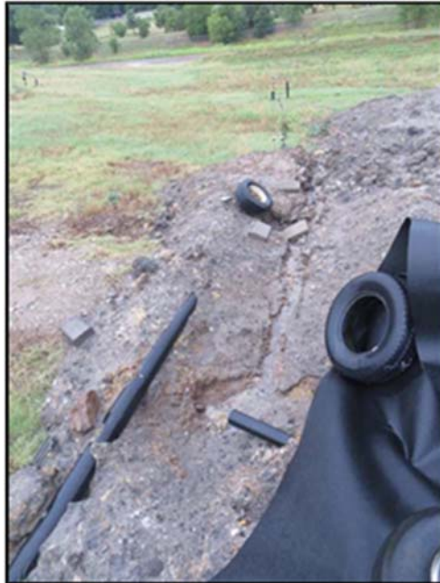
Figure A.181: Gully formed by the flow of water from the south top section.
