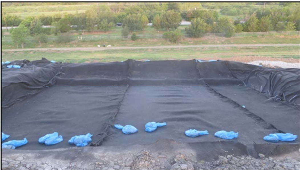
Figure A.303: All of the geosynthetics placed in the north inclined section.
