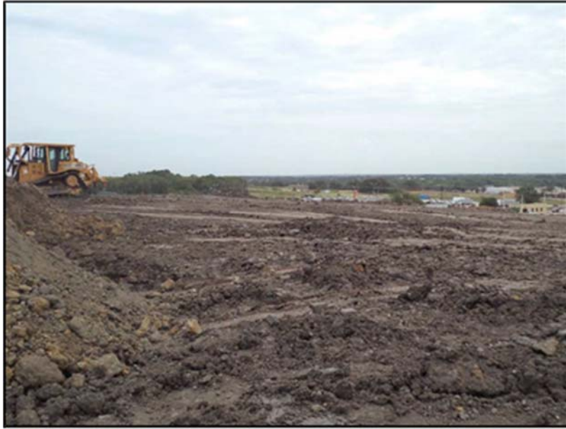
Figure A.34: View of the top section during the sixth day of ET Cover construction.
