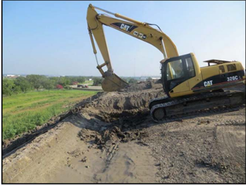
Figure A.254: Removal of water and damp soil from an inclined section by an excavator.
