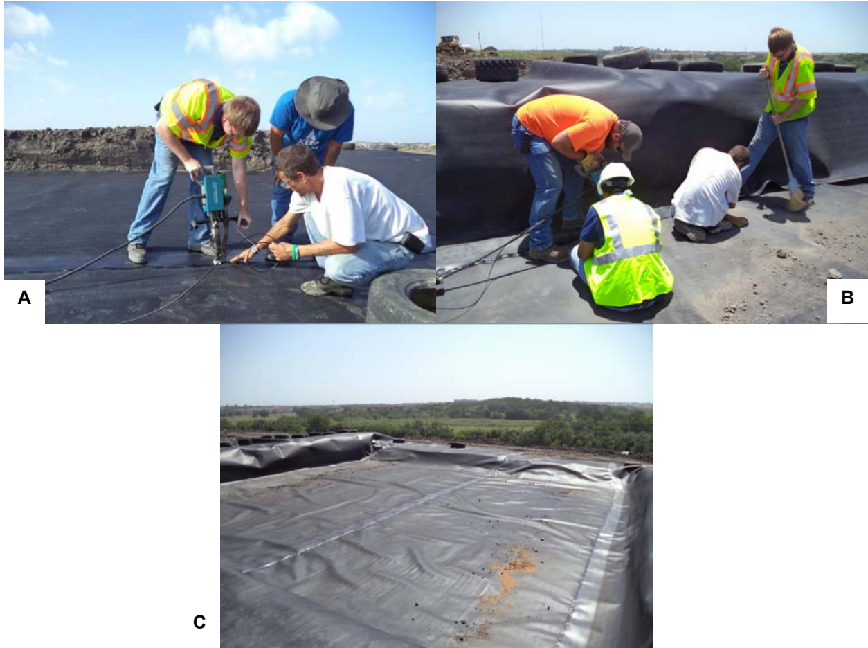
Figure 4.6: Geomembrane placement a) welding the geomembrane, b) sidewall geomembrane welding, and c) finished with the geomembrane in a lysimeter.
