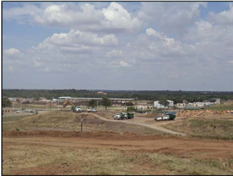
Figure A.19: Obtaining embankment soil from the borrow pit on the fifth day.
