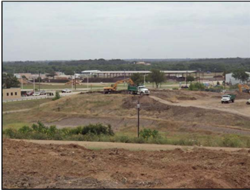
Figure A.33: Obtaining embankment soil from the borrow pit on the sixth day.
