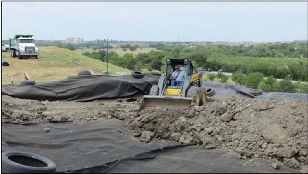
Figure A.157: 1 st soil layer preparation and compaction in the south top section lysimeter-one (1).
