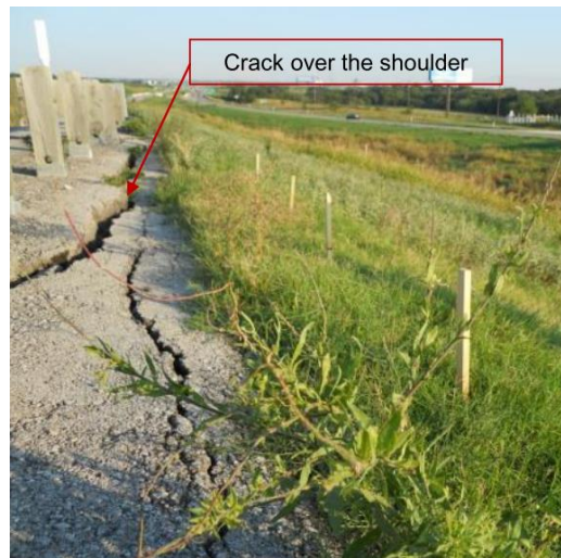
Figure 2-23. Cracks observed in US Highway 287 (Khan, 2014).
