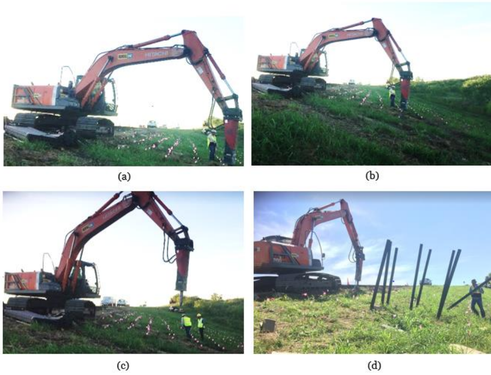
Figure 4-1. RPP installation process: (a) Excavator equipped with a hydraulic hammer, (b) RPP layout using flags, (c) Excavator equipped hydraulic hammer using steel pin to make 1.5 feet deep holes at flag location, (d) RPP placement.
