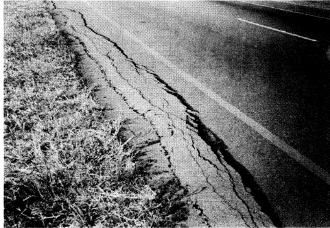
Figure 2-46. Observed edge cracks over pavement stabilized with vertical moisture barrier (Steinberg, 1989).
