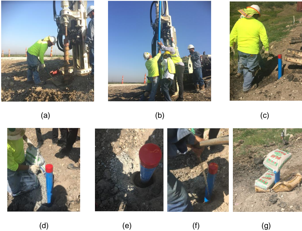
Figure 4-9. Installation of inclinometer: (a) Drilling of boreholes, (b) Placement of inclinometer casing in borehole, (c) Inclinometer casing after placement in borehole, (d) Placement of bentonite, (e) Completely inserted inclinometer casing and bentonite, (f) Pouring of water in bentonite (g) Placement of sandbags on top of inclinometer casing to prevent lifting due to groundwater.
