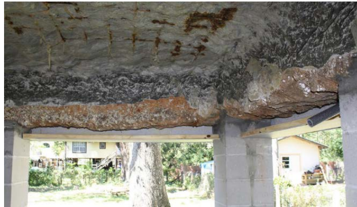
Figure 3-1 Additional beam supports for deteriorated edge beams
