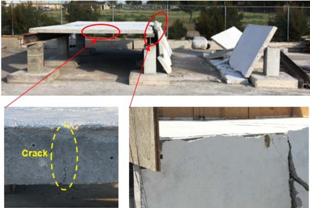
Figure 4-20 Collapse of the control specimen
