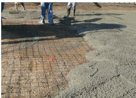
(a) Improper WWF placement
