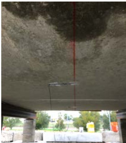
(b) Bottom surface of the slab
