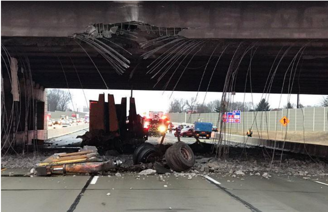
Figure 1-1 Overheight vehicle crash causes significant bridge damage in Indianapolis, Indiana. (FOX59, 2017)
