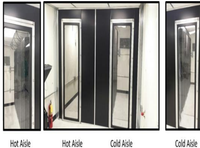
Figure 2-8: Inside the IT Pod [13,14]
