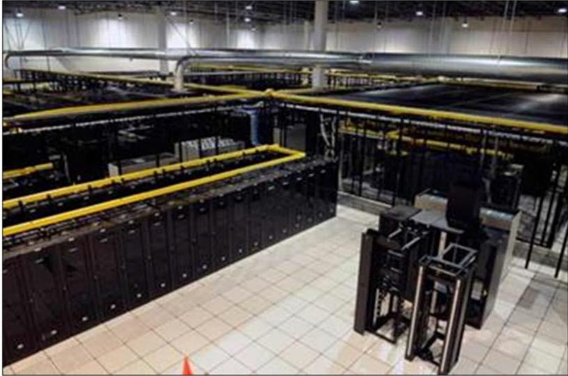
Figure 1-1 Typical interior floor space of a large data center
