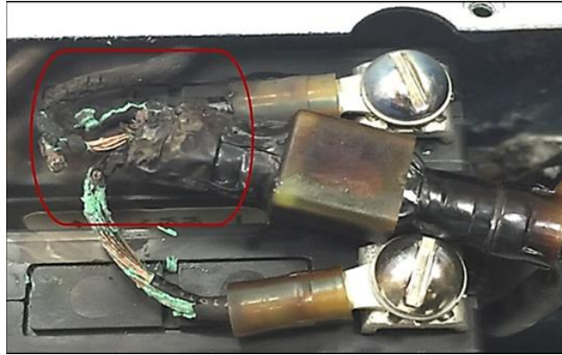
Figure 3-16 Failed PDU-1 at hot aisle
