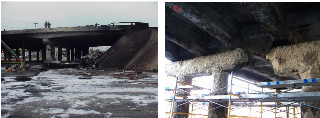
Figure 3-4 Fire damage of MacArthur Bridge (Okafor, Fisher 2005)
