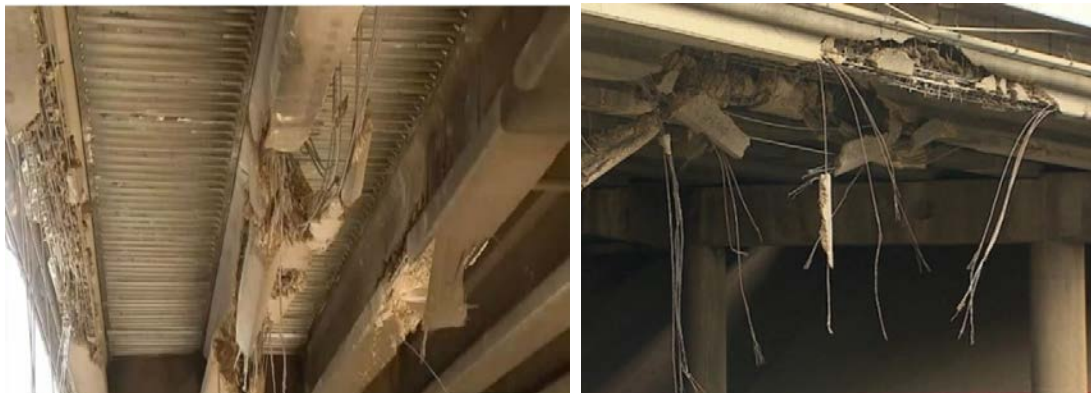
Figure 3-13 Damage of Loop 12 Bridge by over-height vehicle
