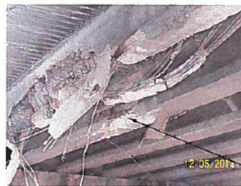
PHOTO - TYPICAL DAMAGE
