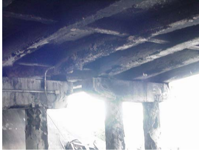
Figure 5-20 Damage on the girders, bent cap and columns
