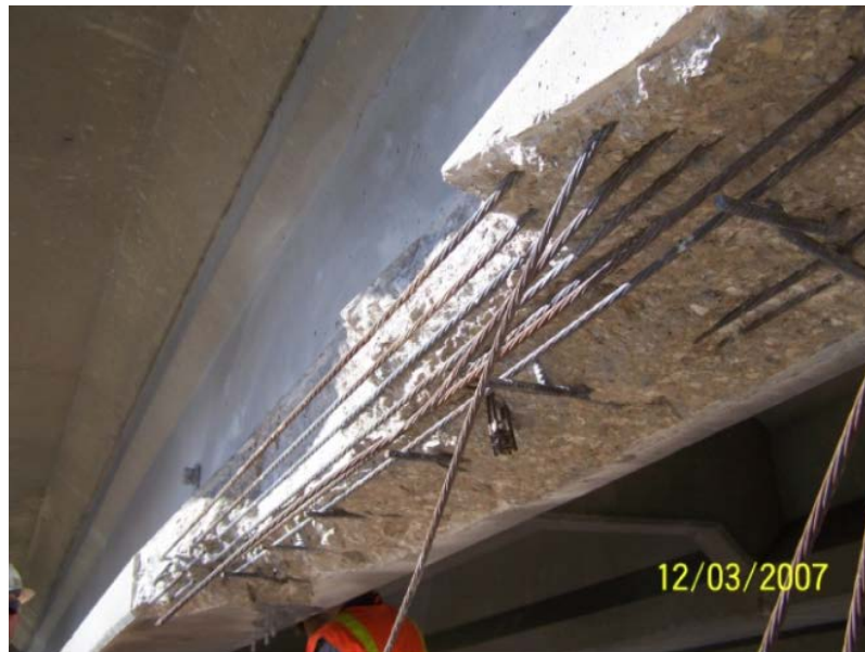
Figure 2-7 Impact-damaged prestressed bridge girder (Kasan et al. 2013)
