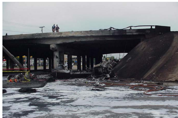
Figure 5-13 Aftermath of fire on MacArthur Bridge
