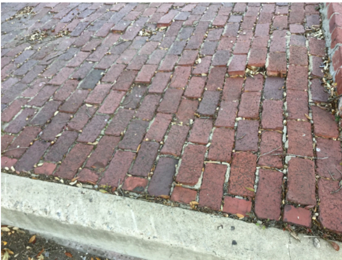
Figure 27. Poor conditioned street (Alamo Street) in downtown Commerce (picture taken on March 16, 2017 by Colby Collins).
