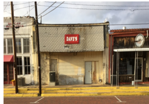
Figure 20. A building in poor condition in downtown Commerce (picture taken on March 16, 2017 by Colby Collins).
