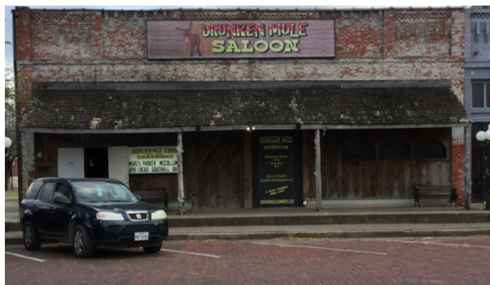
Figure 24. Occupied poor conditioned building in downtown Commerce (Drunken Mule Saloon) (picture taken on March 16, 2017 by Colby Collins).
