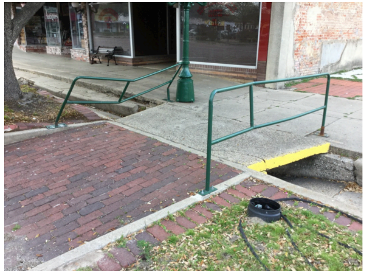
Figure 25. Poor conditioned, hazardous walking rail in downtown Commerce (picture taken on March 16, 2017 by Colby Collins).
