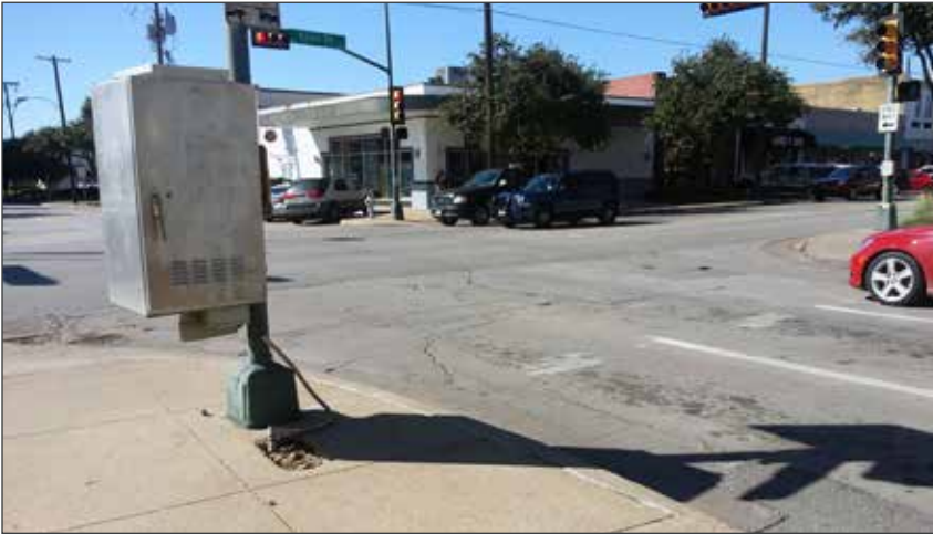
Signalized intersection at Knox Street and Cole Avenue where the pedestrian crosswalk treatments have worn off and not been maintained.
