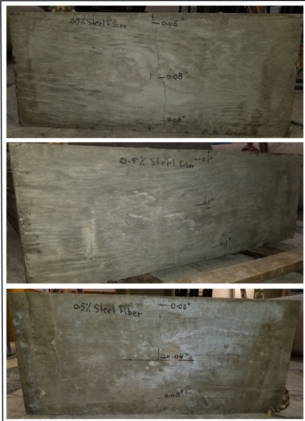
Figure 4- 6. Specimen Failure of SFRC (0.5%)
