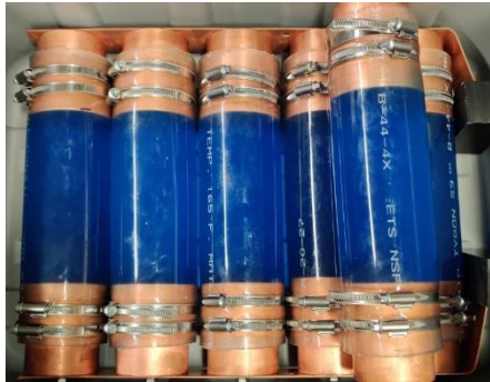
Figure 26: Pictured are the water resistors that will act as part of load the for the CLC charging circuit.
