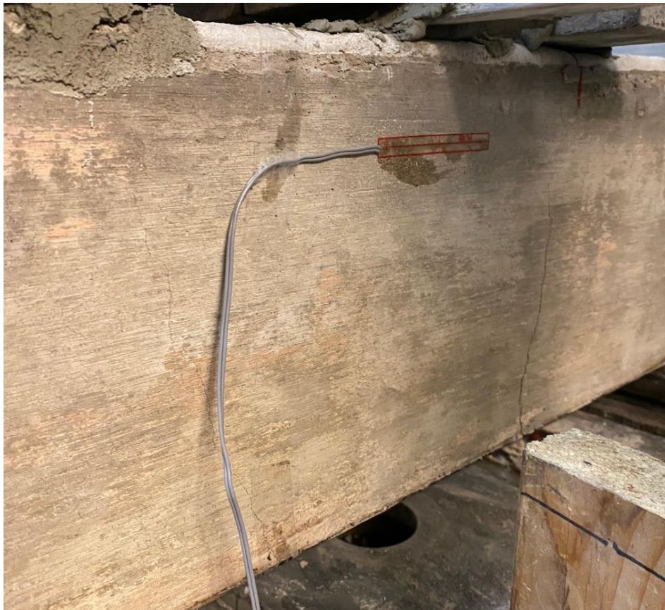
Figure 4.24 Cracks Developed on Beams with Glass Components with 30 Minutes Heat Treatment
