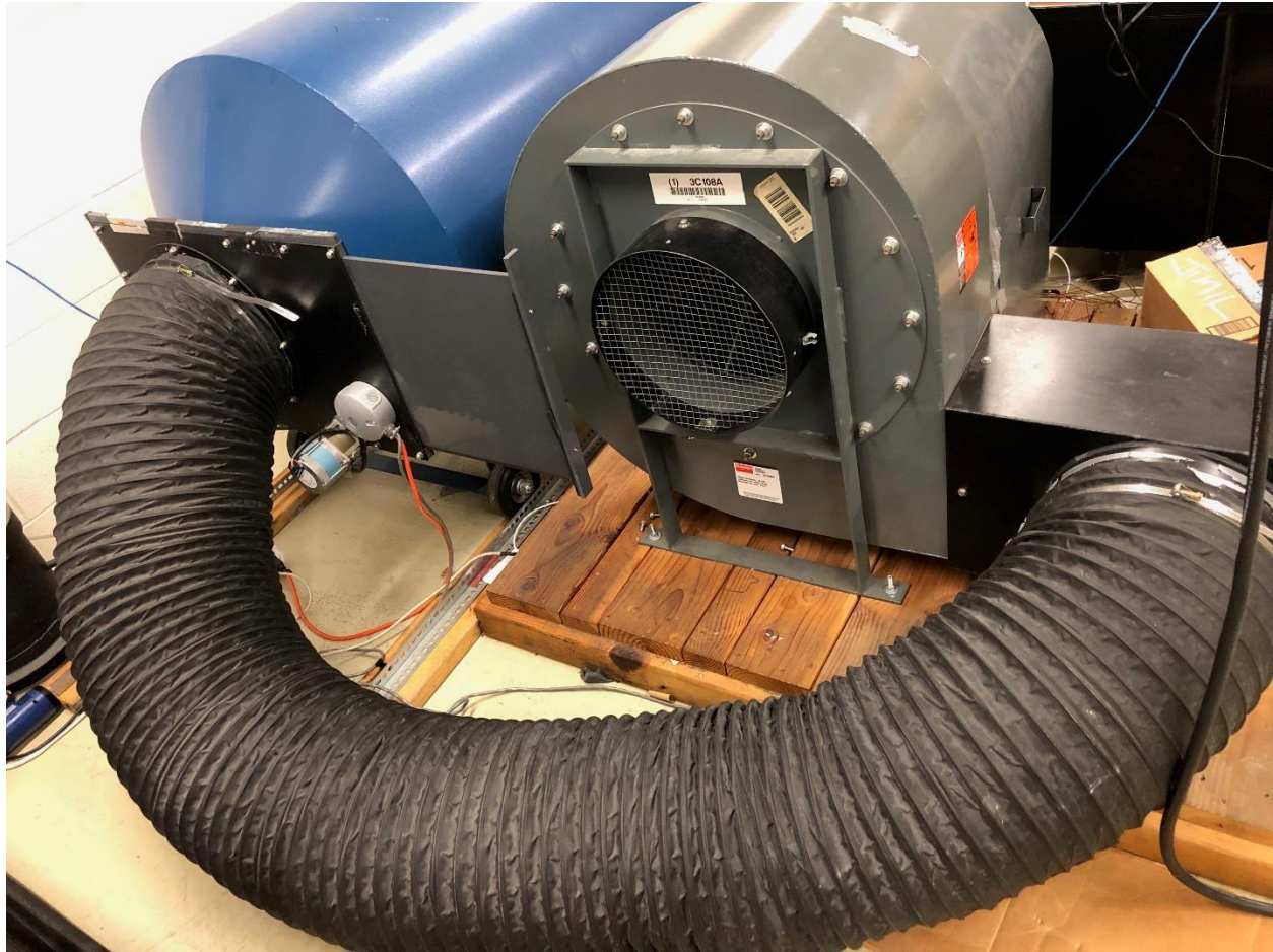
Figure 23 Flexible hose connecting blower with airflow chamber
