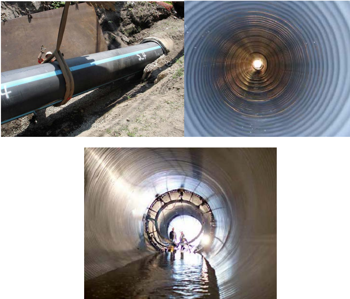
Figure 1-2: Culvert rehabilitation using (left to right): sliplining (DEWCON Infrastructure Rehabilitation 2019), fold-and-form lining and spiral wound lining (Matthews et al. 2012).
