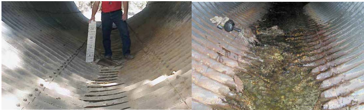
Figure 2-4: Invert damage due to abrasion (left) and corrosion (right) (Matthews et al. 2012)
