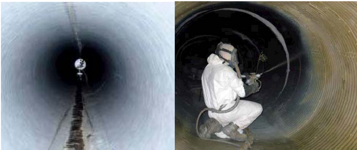
Figure 1-3: Pipe repair using (left to right): CIPP and spray applied liner (Matthews et al. 2012).
