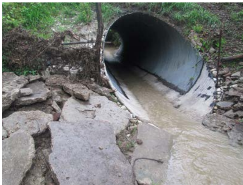
Figure 1-1: 9 ft. diameter CMP with corrugated invert on Elba Township in Knox County, Ill (Miliken Infrastructure Solutions 2016).
