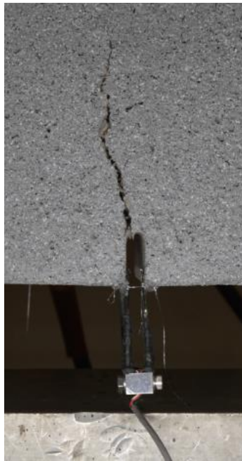
Figure 4.2 Clip Gauge crack measurement
