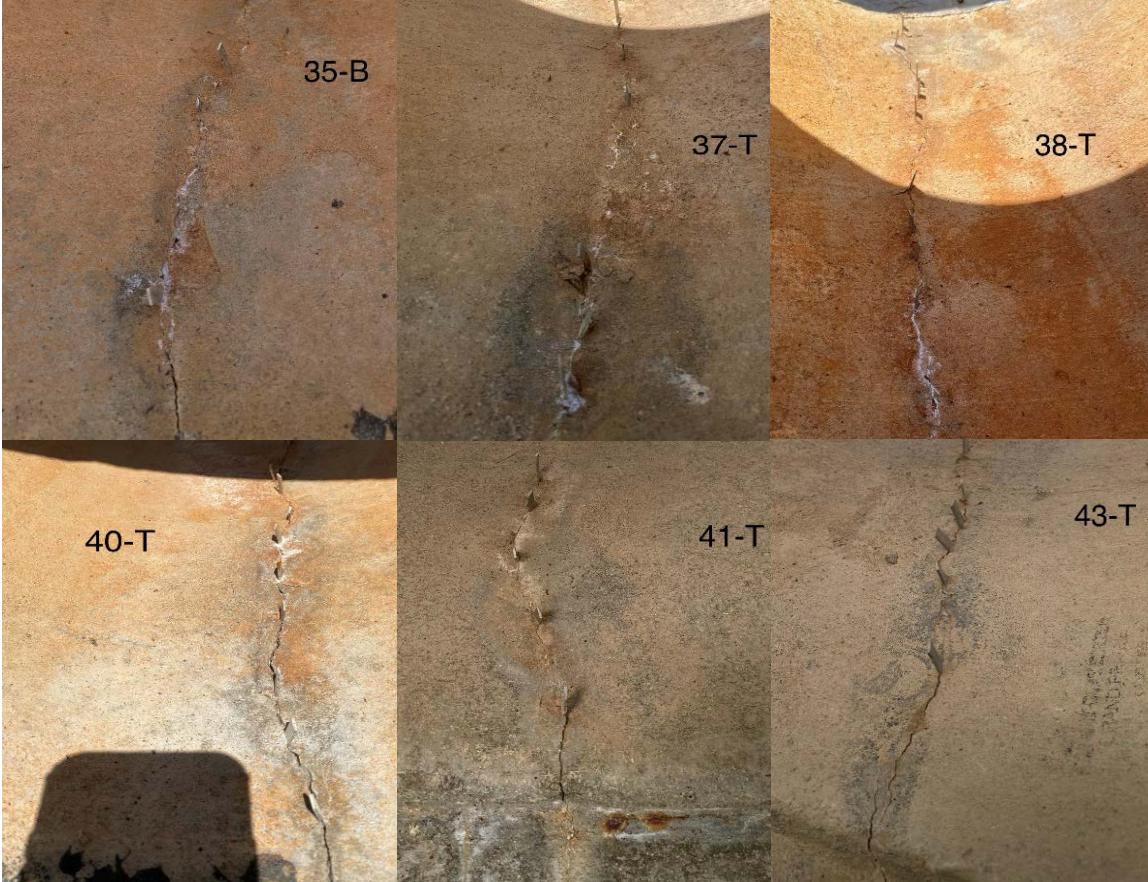
Figure 112: Autogenous healing and cracks sealing in the 30,000 PPM solutions.
